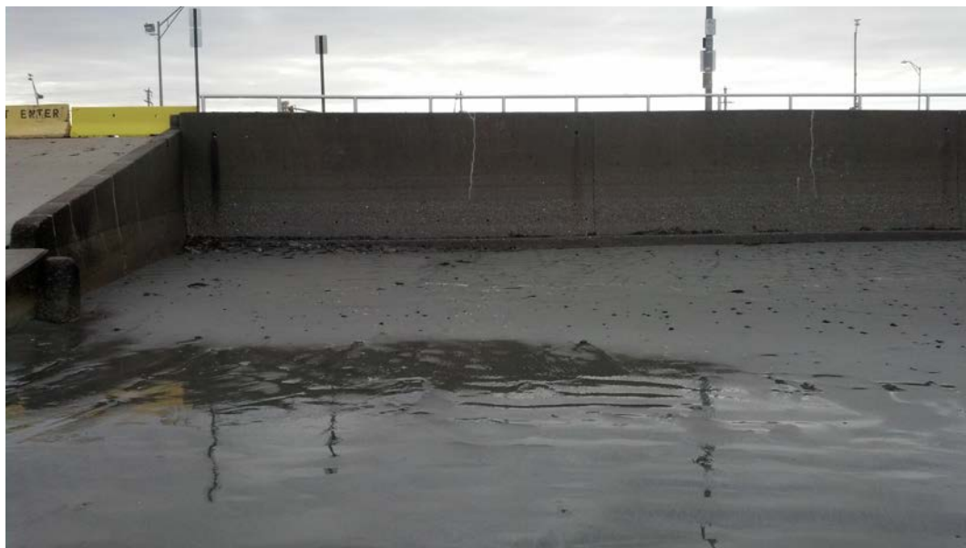
Photo 3 This view of the sea wall taken after a storm shows the portion of the wall footing is exposed.
