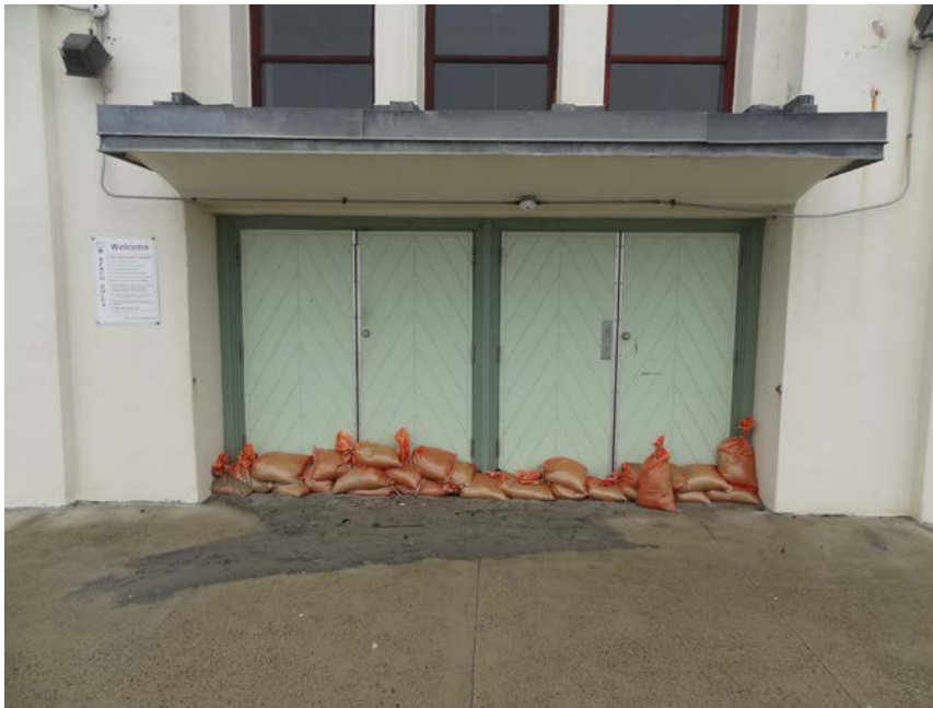
Photo 8 These sand bags are a necessary off season measure to prevent water coming over the sea wall from entering the DCR bath house.
