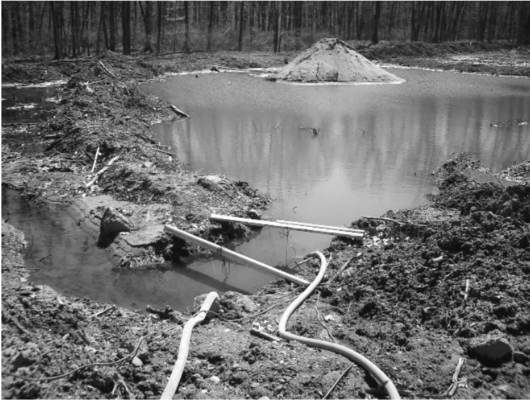
FIGURE 12.1 Direct vernal pool destruction still occurs, despite wetland regulations. Here, a vernal pool is being drained prior to filling during construction of a single-family house in Plainfield, CT. Photo courtesy of Vin Mullin.
