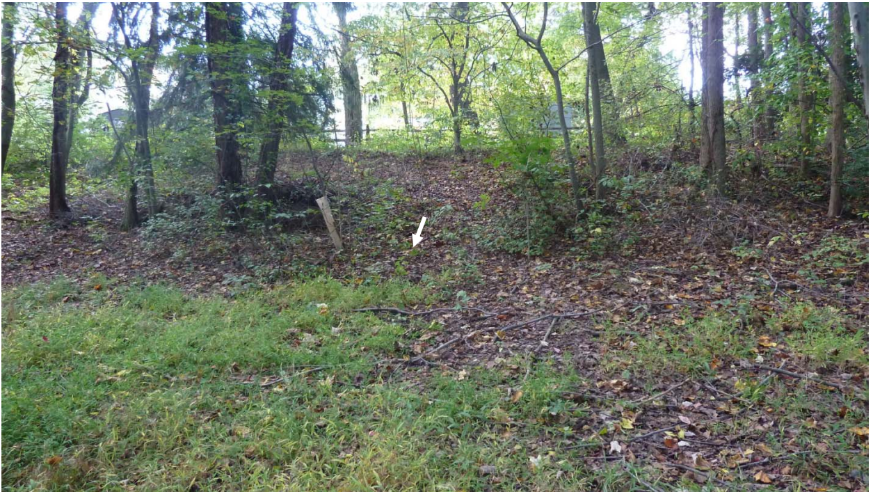
Photo 11. HR1. R.O.W. is in the foreground. Arrow indicates backslope seep.
