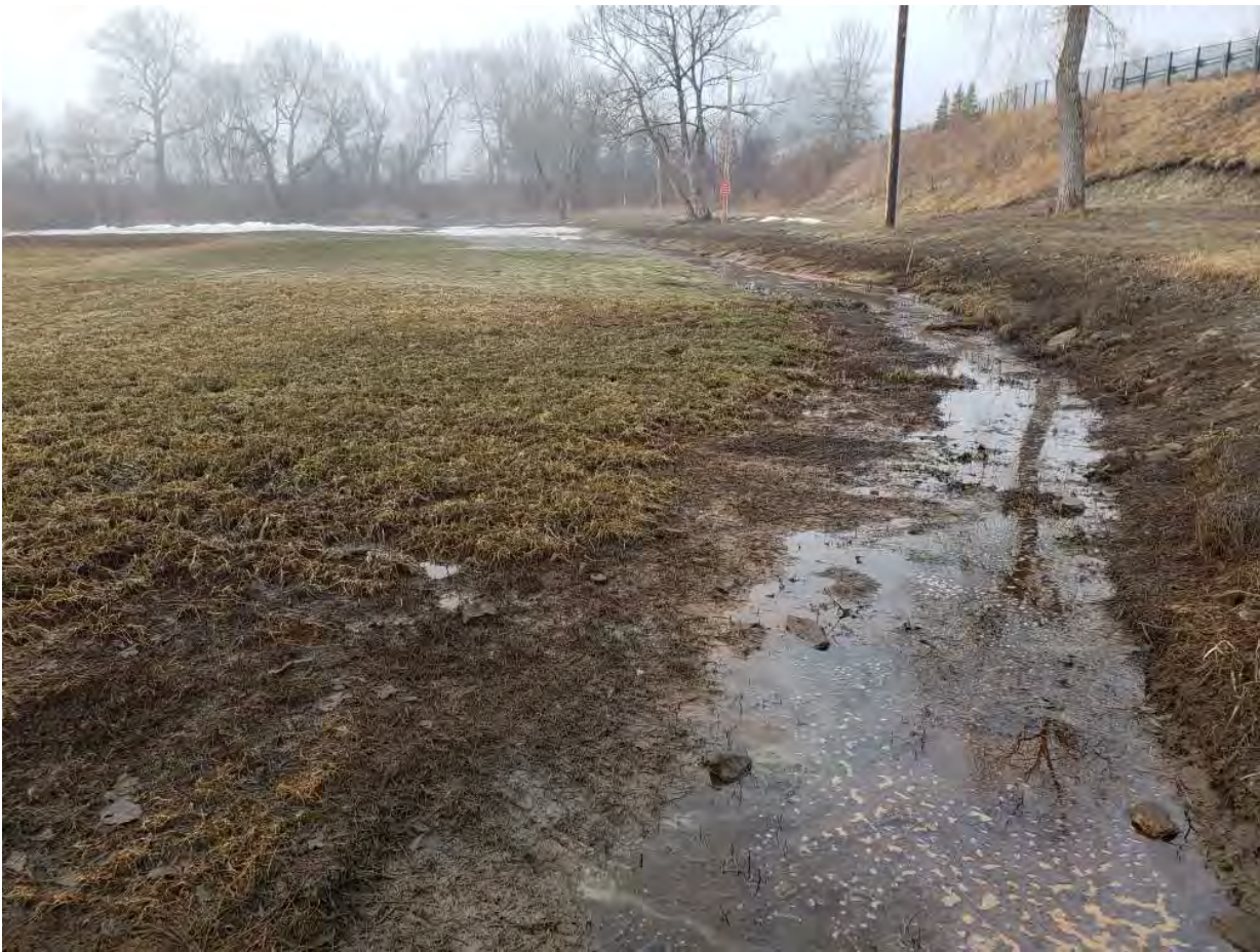
Photo 5: View looking at southwest channelized flow at toe of U.S. Route 1 embankment.
