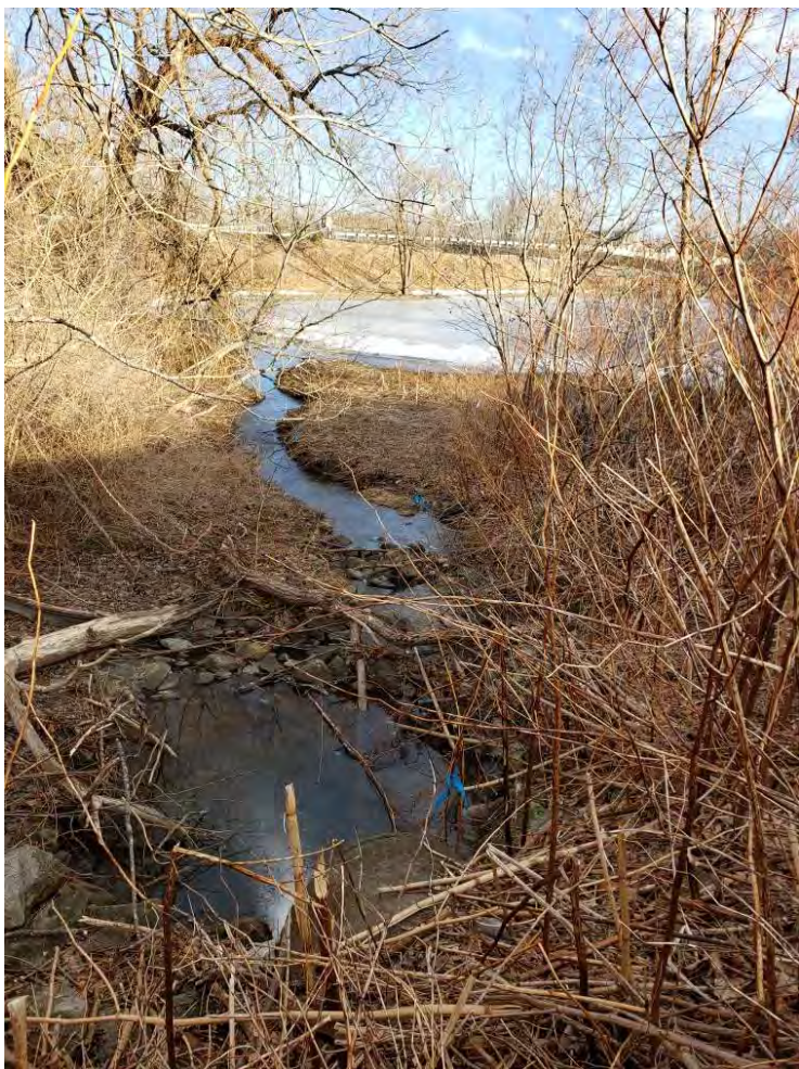
Photo 7: View looking north/northwest at flowing water from outlet of culvert beneath athletic field.
