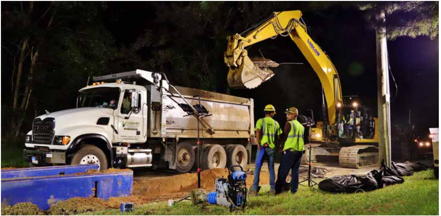
Ludlow Construction Company, Inc., performs work on the Durham Meadows Water Main Construction project.
