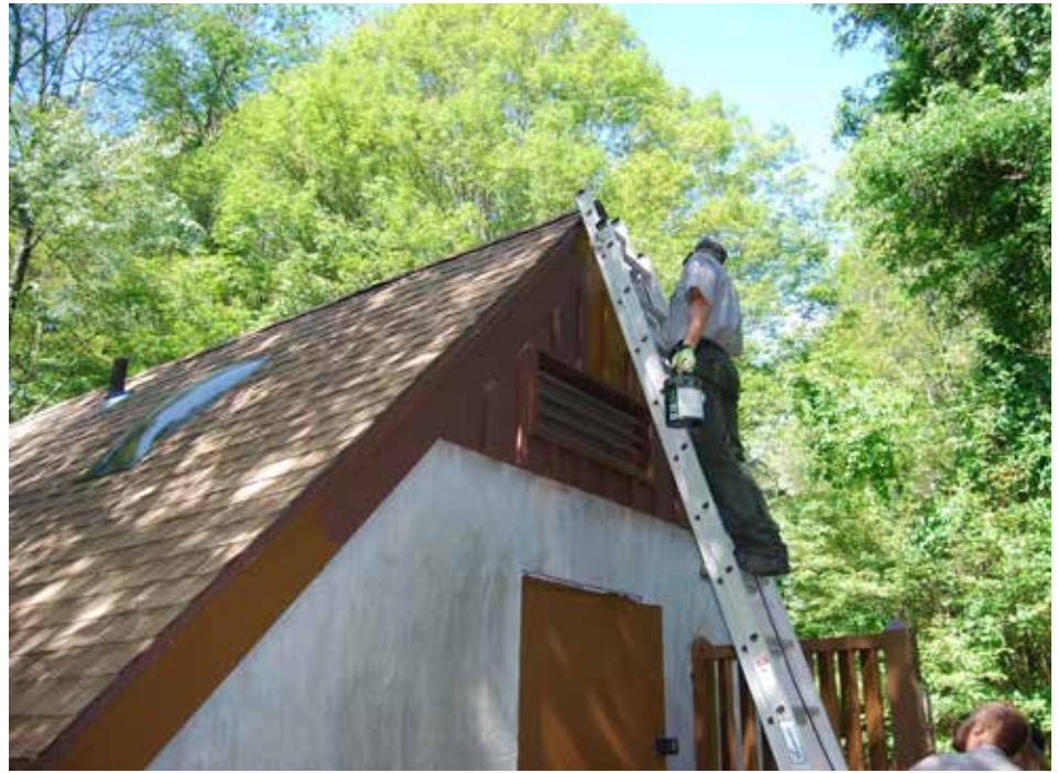
A summer ranger works on a roof at Hop Brook Lake while another holds the ladder.
