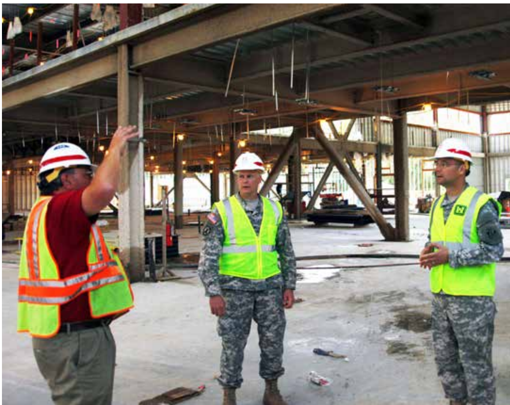
Steve Chase briefs Col. Christopher Barron and Brig. Gen. William Graham during a tour of the Hanscom AB Middle School project.
