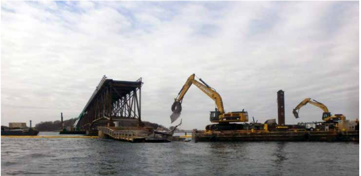
Contractor Walsh Construction removes and sorts bridge debris with barges and excavators
