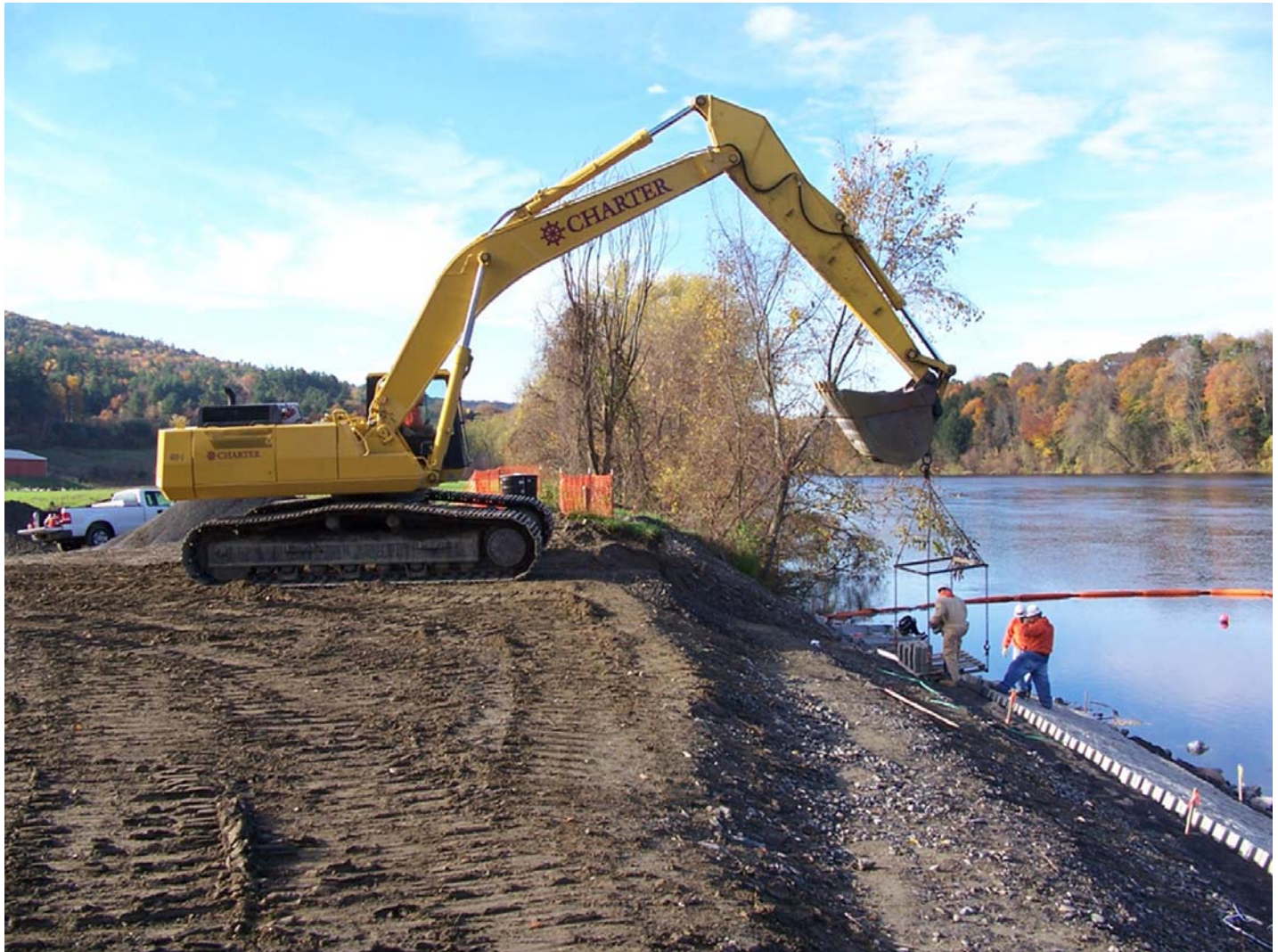
The Emergency Streambank Protection of Partridge Brook, Westmoreland, N.H., is one of many contract awards that Eva Marie D'Antuono has handled. The contractor is a small business, Charter Environmental, Inc.
