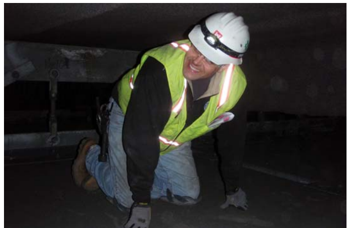
Scott Acone inspects a Ceiling Plenum during the Big Dig Stem to Stern Safety Review.
