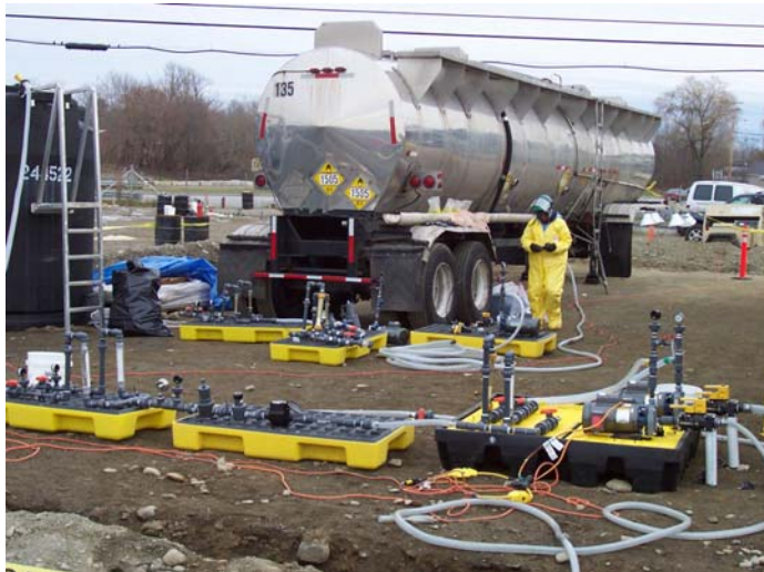
Eastland Woolen Mill Superfund Site in Corrina, Maine.
