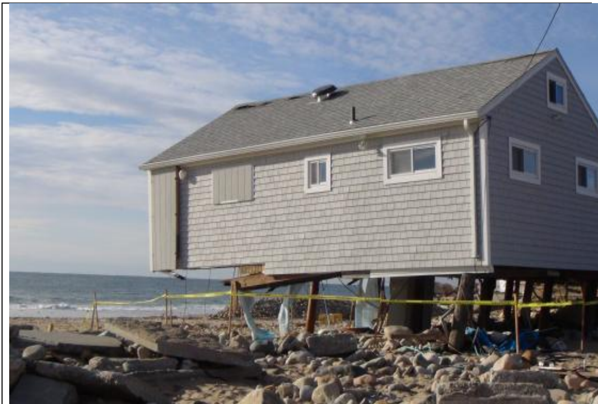
Figure 10. Damaged Home after Hurricane Sandy (October 2012)
