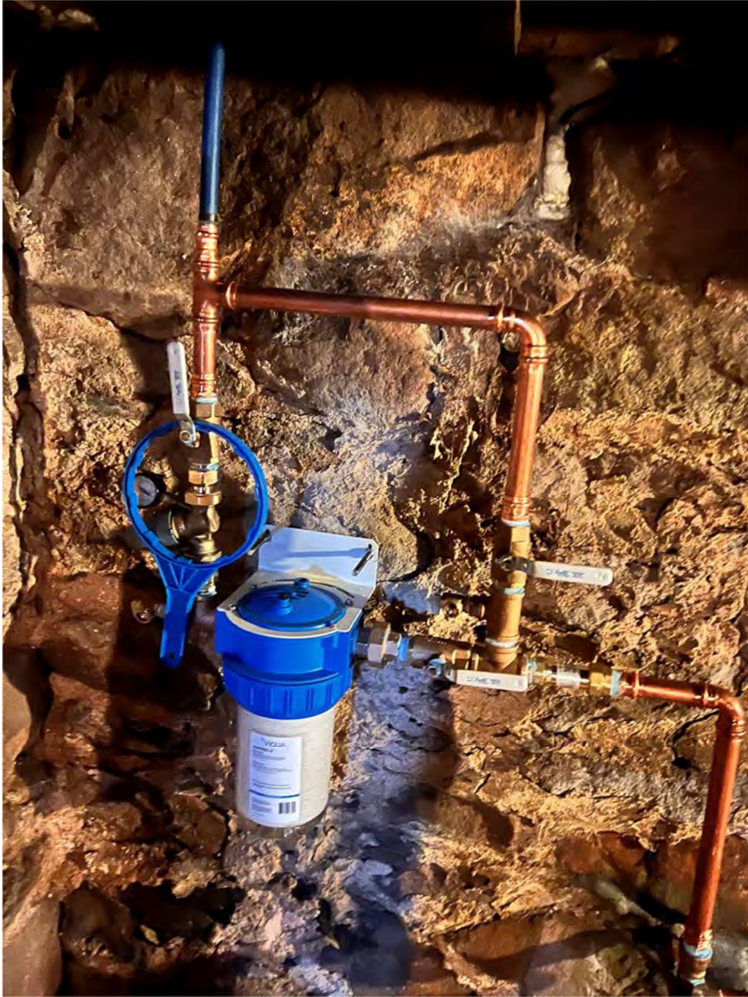
Picture 6: Fazzino Plumbing new water service components in the basement of 55 Main Street.
