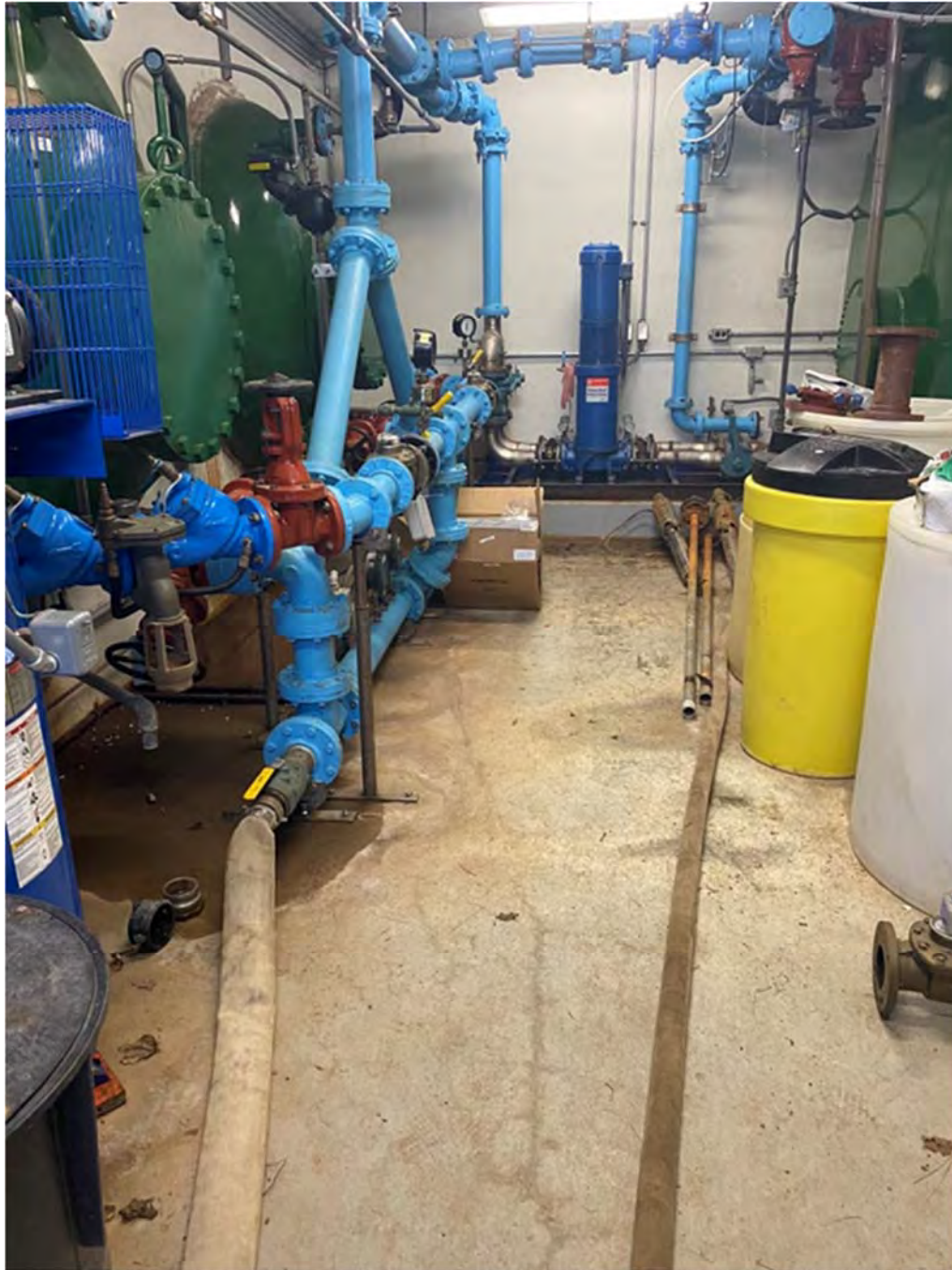
Picture 1: Ludlow connects hoses and drains the hydropneumatic tanks and atmospheric water storage tank at the Durham booster station. View to the east.
