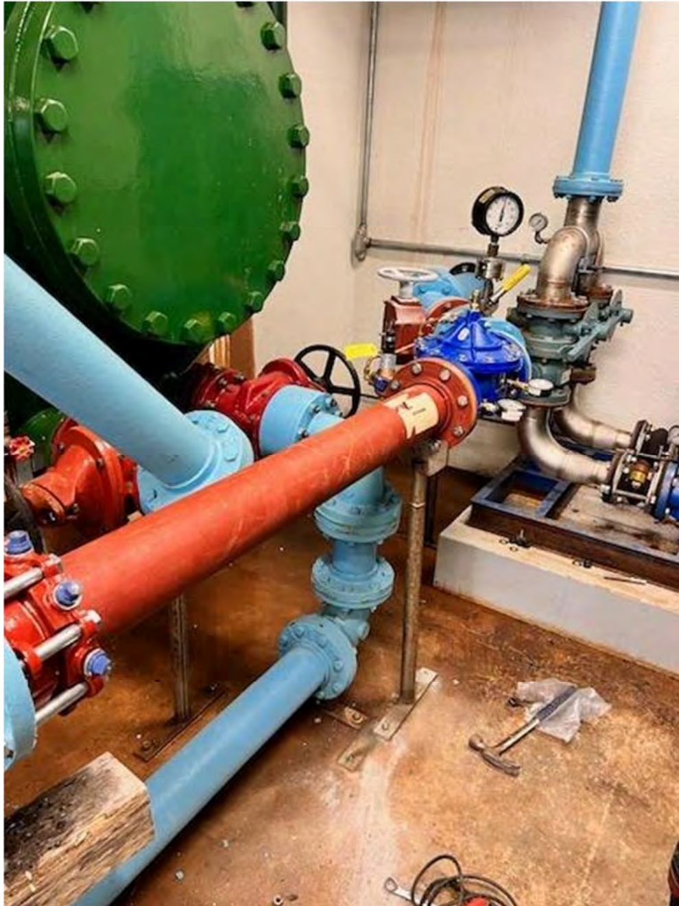
Picture 4: Ludlow removes 4" water meter and installs a pressure reducing valve at the Durham booster station for a water supply to the Durham Fairgrounds.
