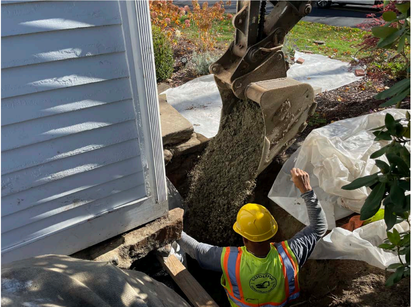
Picture 4: Ludlow placing 1.25" processed gravel around the southwest corner of the 24 Maiden Lane, Durham, residence. View to the south.
