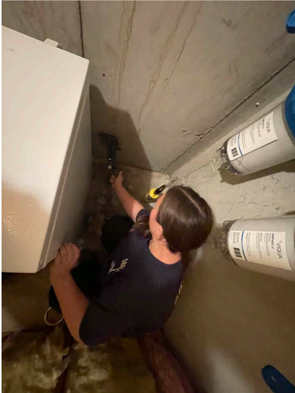
Picture 1: Grela installing a plug into the HDPE well line that enters the north side of the 228 Maple Avenue, Durham, residence. View to the north.
