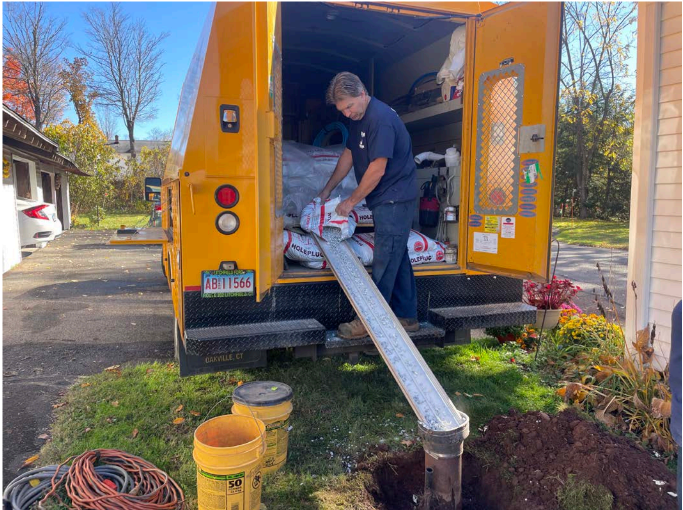
Picture 3: Grela placing bentonite chips into the well located on the northeast corner of the 228 Maple Avenue, Durham, residence. View to the east.
