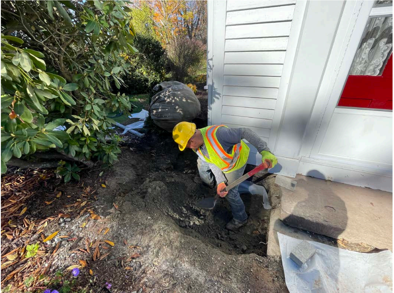
Picture 6: Ludlow placing 1.25" processed gravel around the southwest corner of the 24 Maiden Lane, Durham, residence. View to the northwest.
