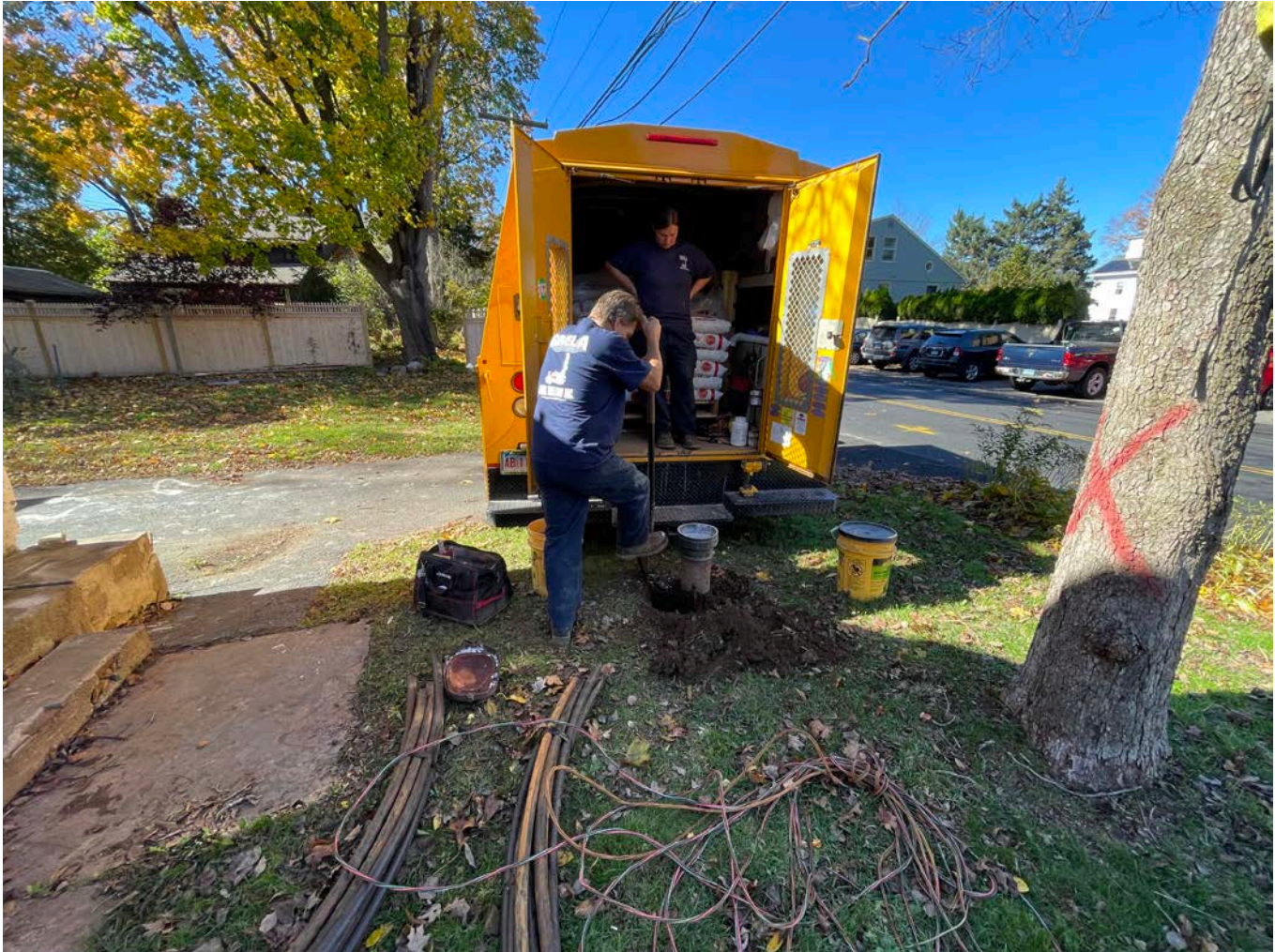
Picture 5: Grela hand excavating around the steel riser of the well located on the north side of the 11 Maiden Lane, Durham, residence in order to cut it below grade. View to the northwest.
