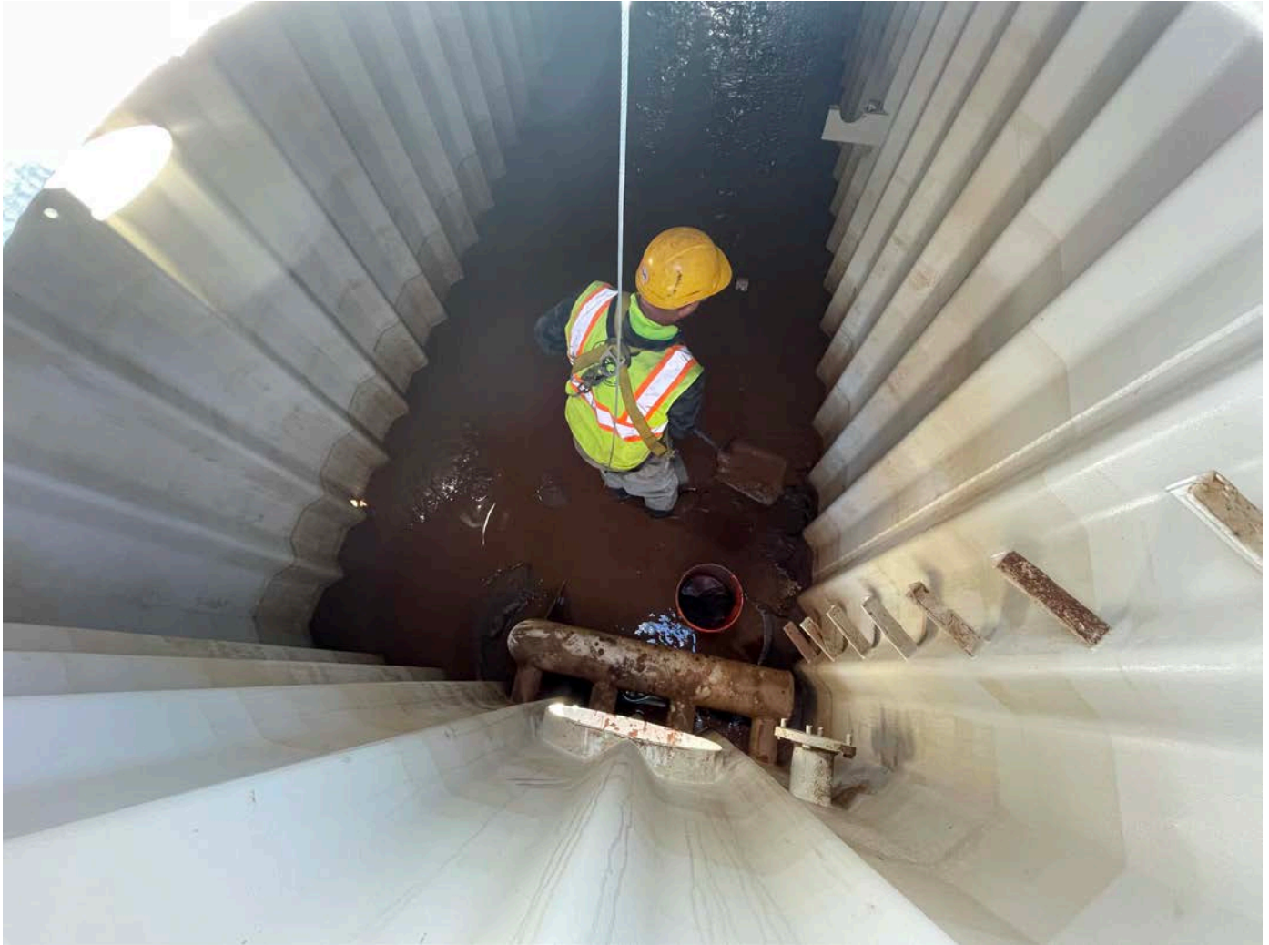
Picture 4: Ludlow removing sediment from the bottom of the frac tank located on the 281 Main Street, Durham, property.
