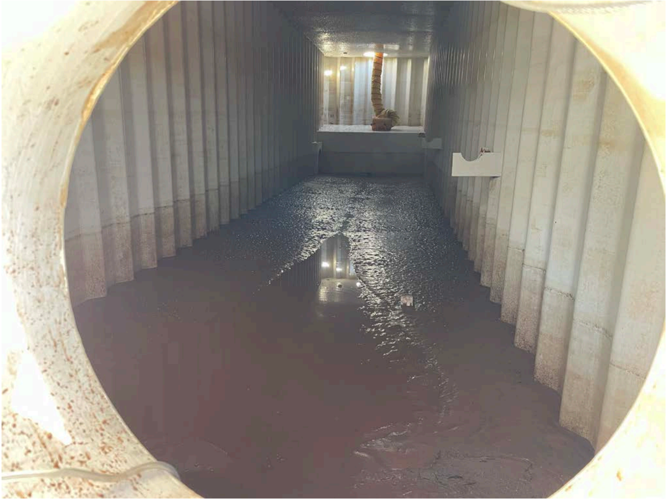
Picture 2: Accumulated sediment located inside of the frac tank located on the 281 Main Street, Durham, property. View to the north.
