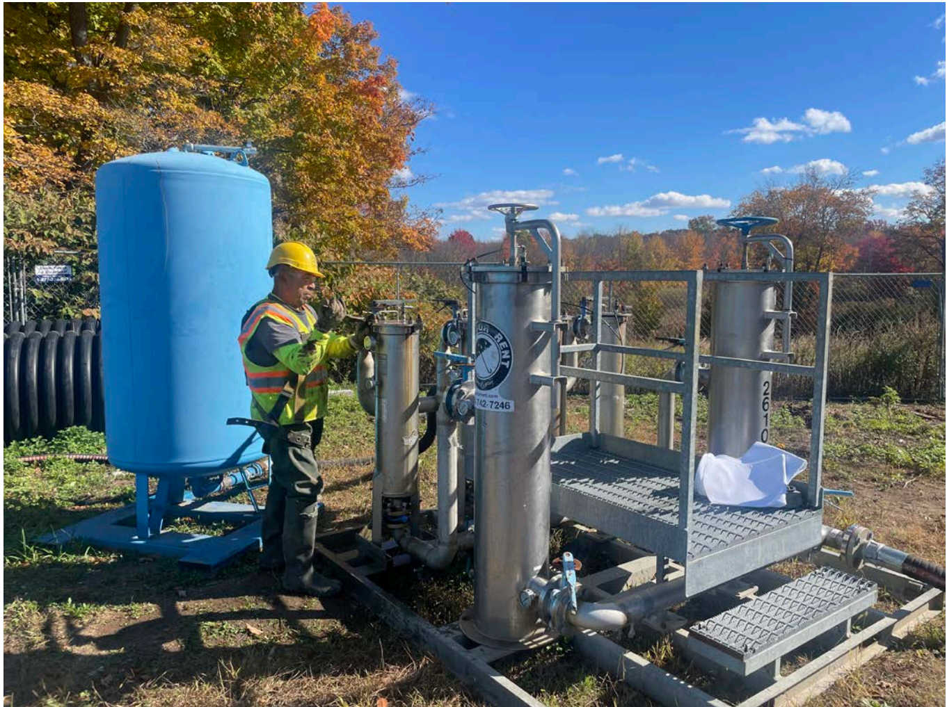
Picture 5: Ludlow dismantling the temporary treatment system located at the 281 Main Street, Durham, property. View to the east.
