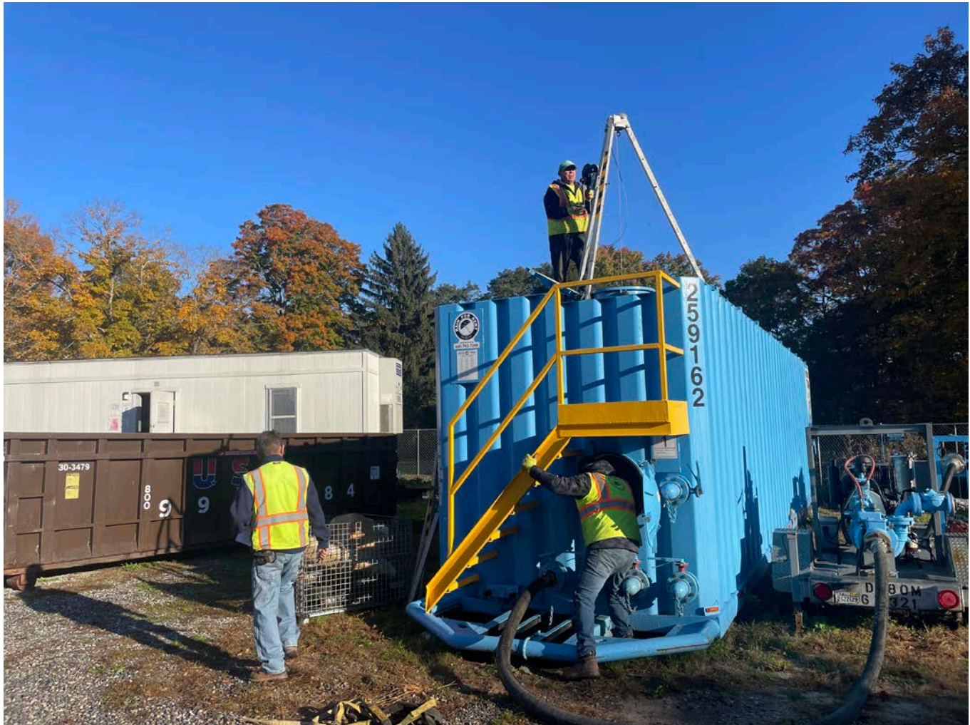
Picture 1: Ludlow setting up to perform a confined space entry into the frak tank located on the 281 Main Street, Durham, property. View to the north.
