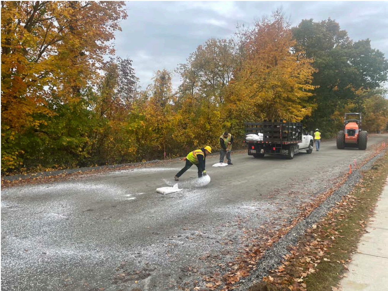
Picture 2: Ludlow spreading calcium chloride onto the 1.25" processed gravel they placed between Stations 10+00 and 18+13 on Pickett Lane. View to the southwest.
