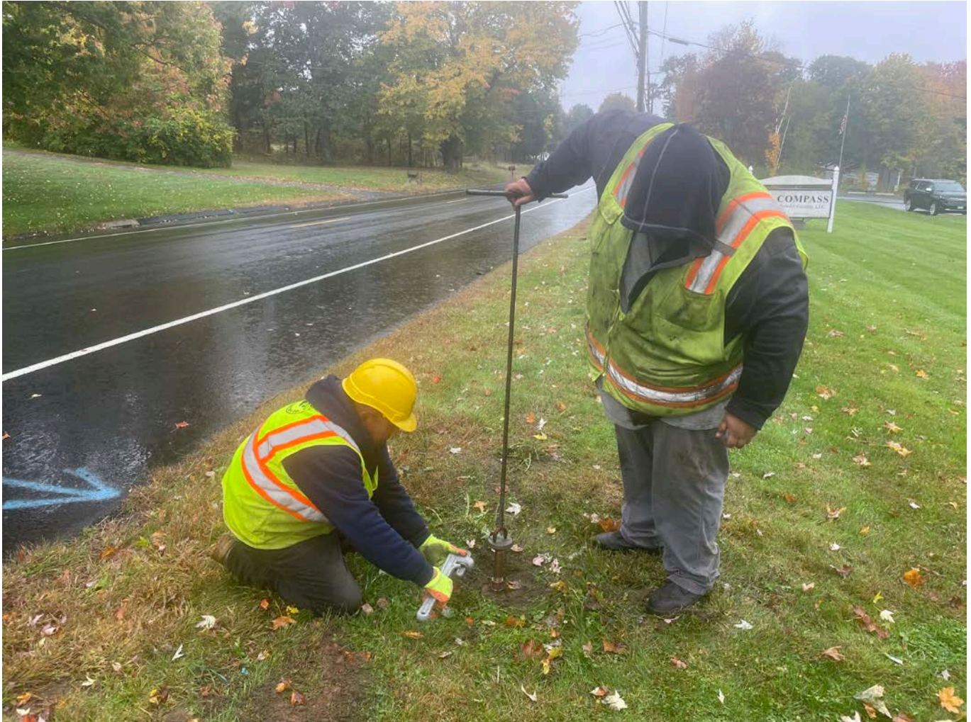
Picture 3: Ludlow adding a 6" riser to the curb box located on the 2303 S. Main Street, Middletown, property. View to the southeast.
