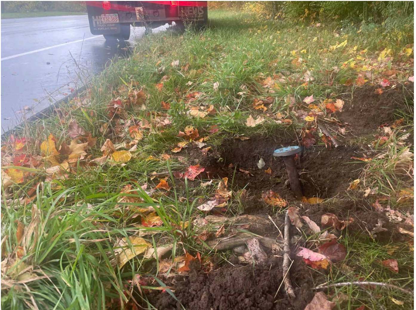
Picture 4: View of a damaged curb box on the 2246-2266 S. Main Street, Middletown property that Ludlow daylighted to assess repair options. View to the north.
