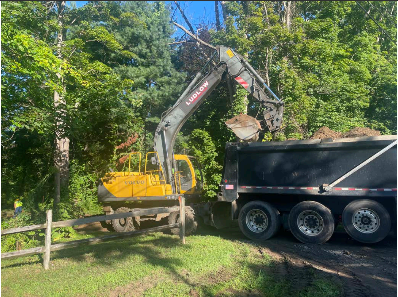
Picture 1: Ludlow is excavating fill on the east side of the driveway for the 212R Main Street property. View to the north.
