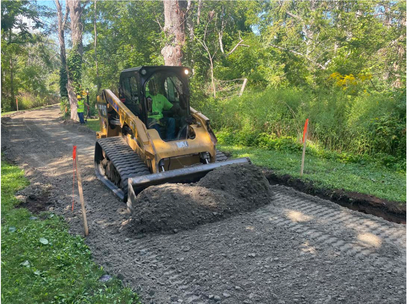
Picture 4: Ludlow grading 1.25" processed gravel on the footprint of the 212R Maple Avenue driveway. View to the west.
