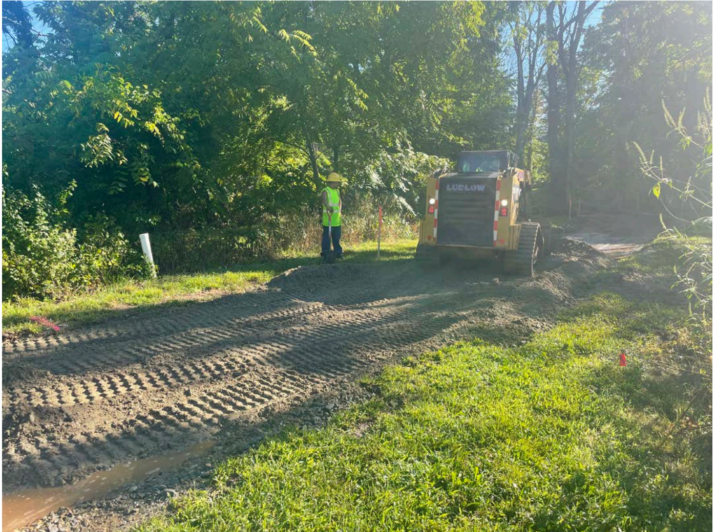
Picture 2: Ludlow grading 1.25" processed gravel on the footprint of the 212R Maple Avenue driveway. View to the east.
