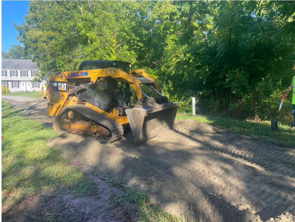
Picture 3: Ludlow grading 1.25" processed gravel on the footprint of the 212R Maple Avenue driveway. View to the west.
