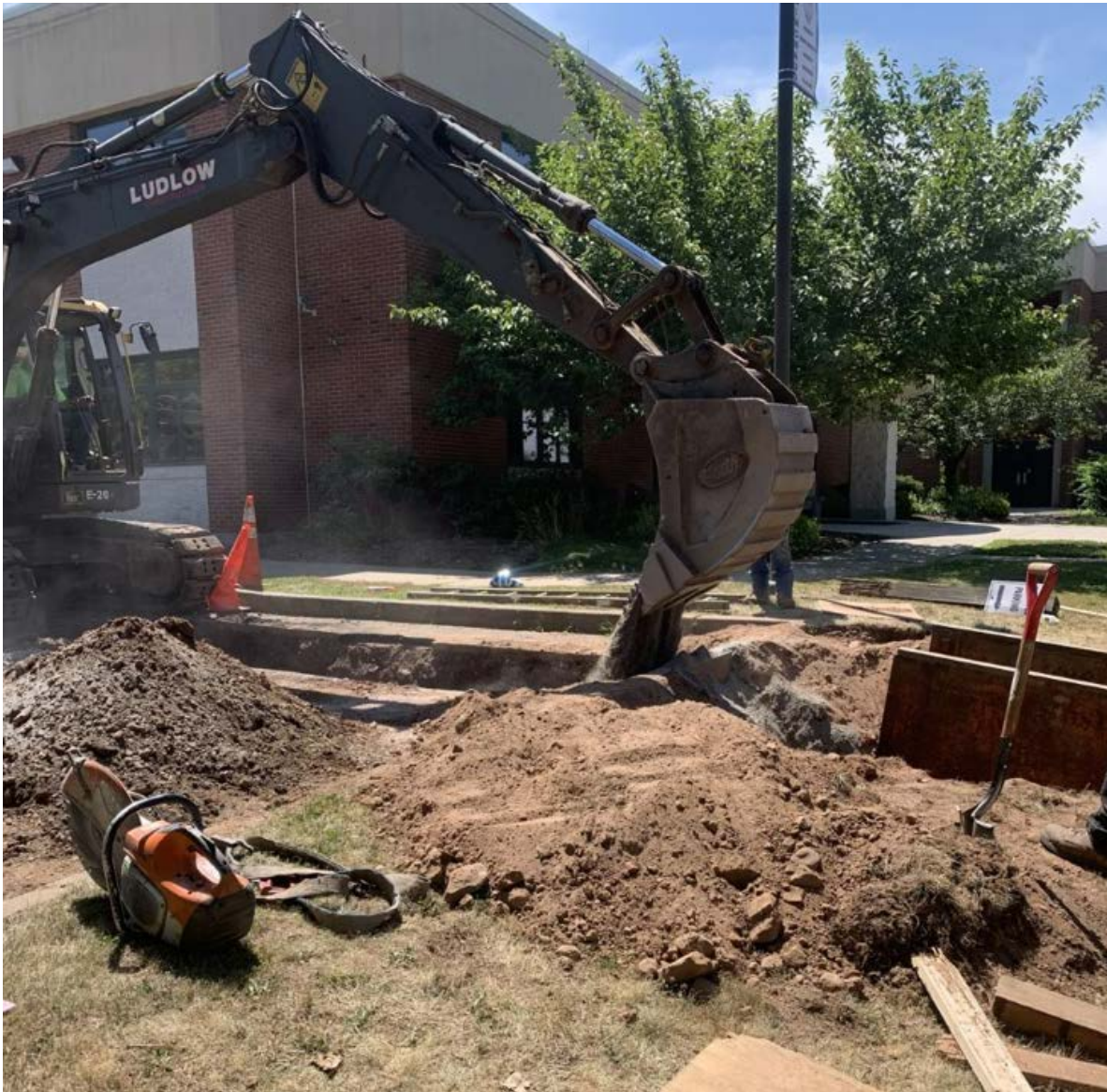
Picture 2: Ludlow Construction is backfilling the trench with soil, sand, and gravel at Cuginchaug High School.
