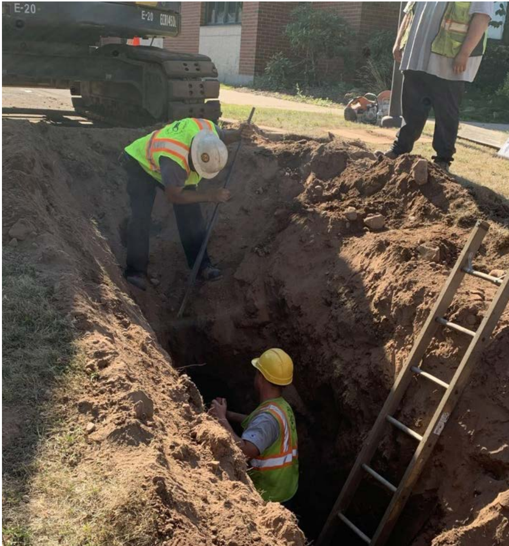
Picture 1: Ludlow construction is excavating a trench to install a 4" water service line at Coginchaug High School using personnel and an excavator.
