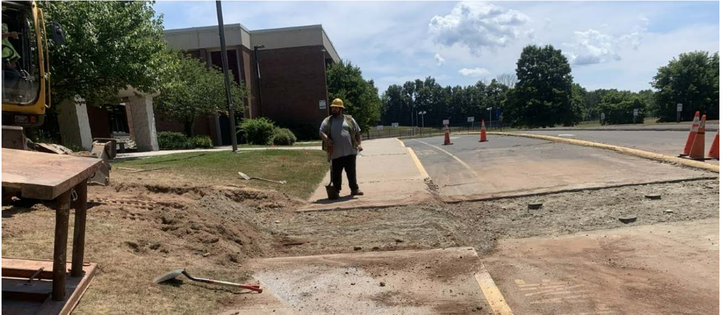
Picture 3: Ludlow Construction is grading the backfilled trench area at Coginchaug High School.
