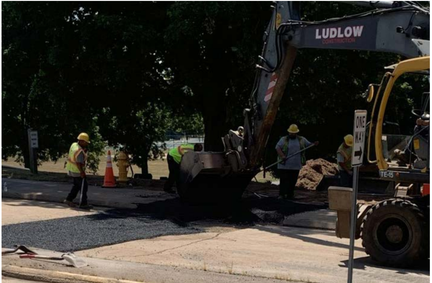
Picture 4: Ludlow Construction places asphalt on the previously excavated area at Coginchaug High School.
