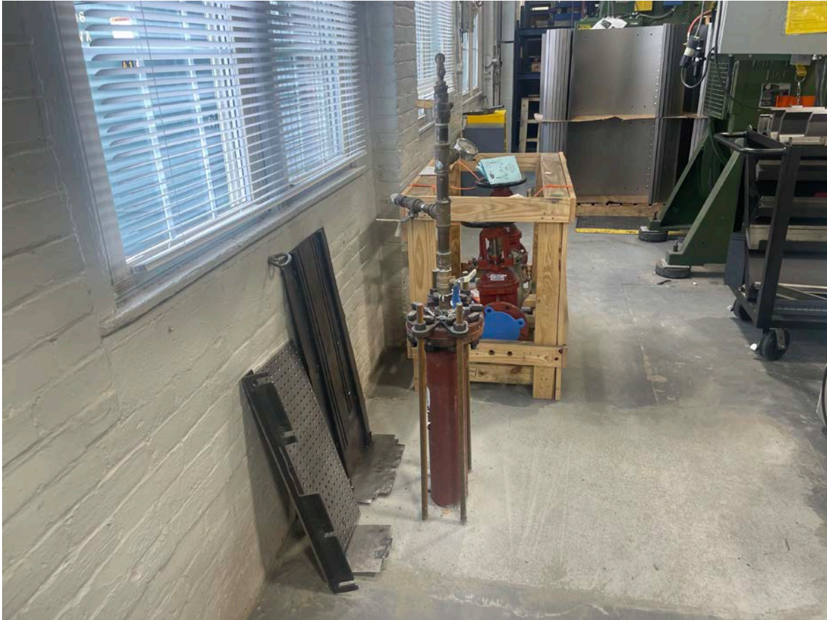
Picture 1: Water service line that Ludlow previously brought into the Durham Manufacturing facility through the west side of the building. View to the north.
