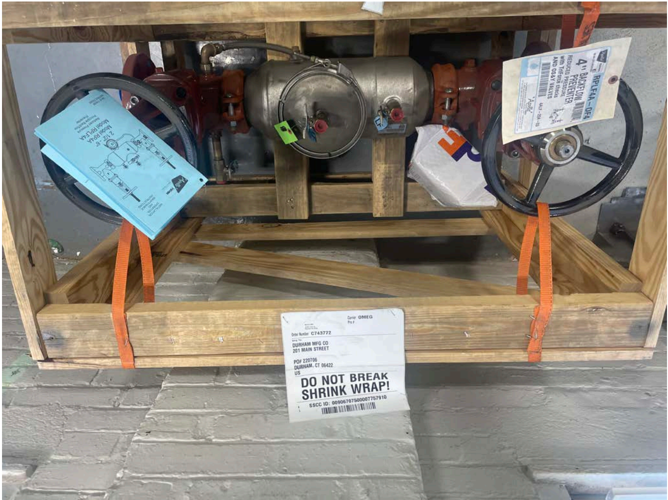
Picture 2: Backflow preventer that West State Mechanical is preparing to install on the water service that Ludlow brought into the Durham Manufacturing Facility.
