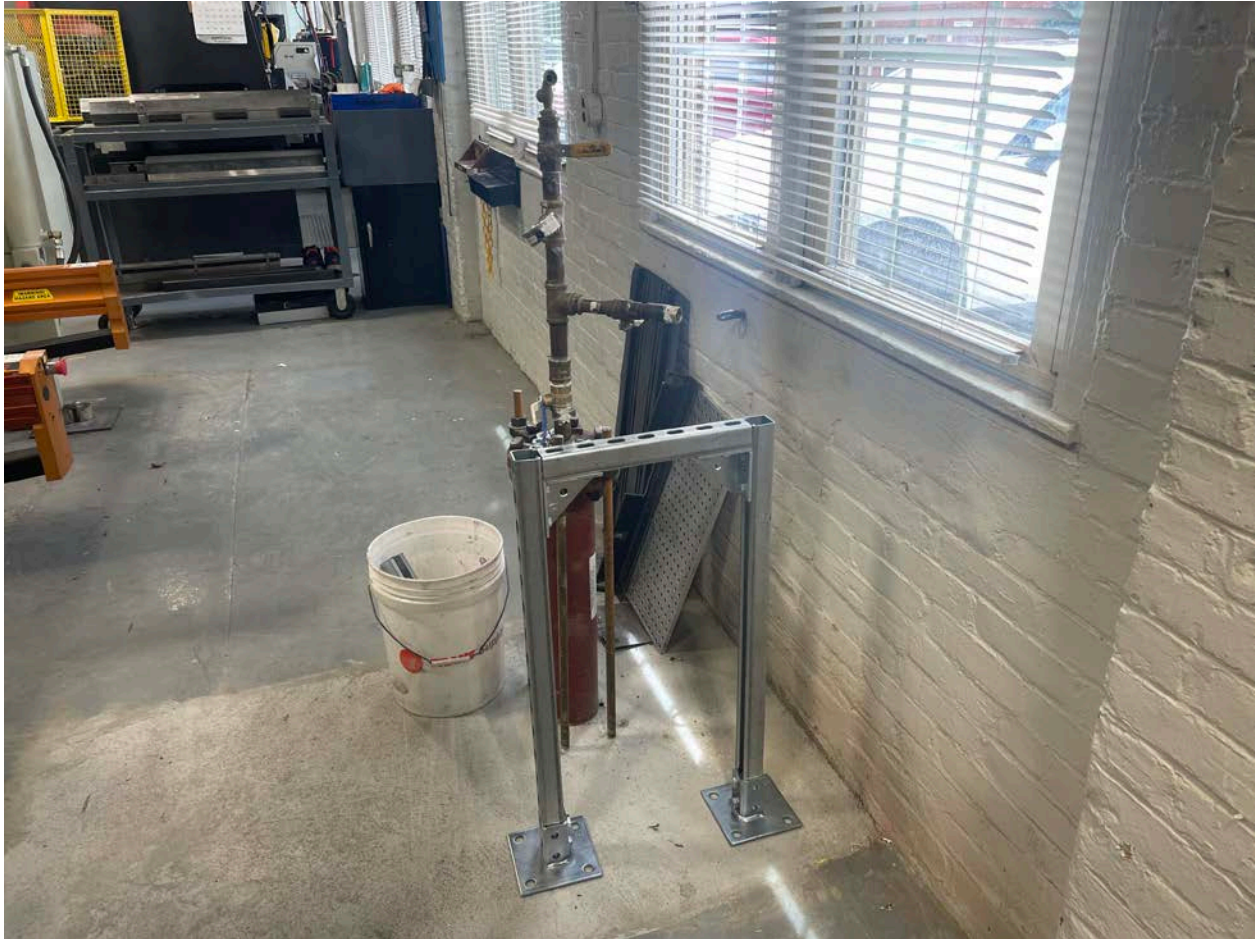
Picture 3: A portion of the stand that West State Mechanical installed on the north side of the water service that was brought into the Durham Manufacturing facility to support the backflow preventor they will be installing. View to the southwest.
