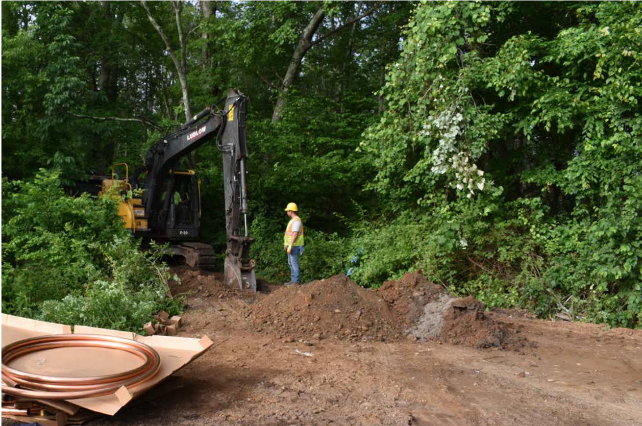
Photo 1: Ludlow crew continuing excavation of pipe trench along driveway at 114 Maiden Lane. View to the southwest.
