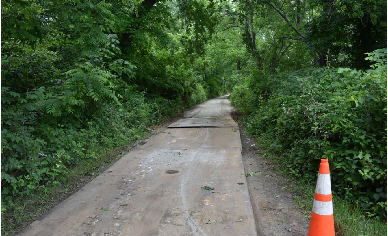
Photo 6: Steel plates covering open trench and driveway over brook culvert at 114 Maiden Lane at the end of the work day. View to the north.
