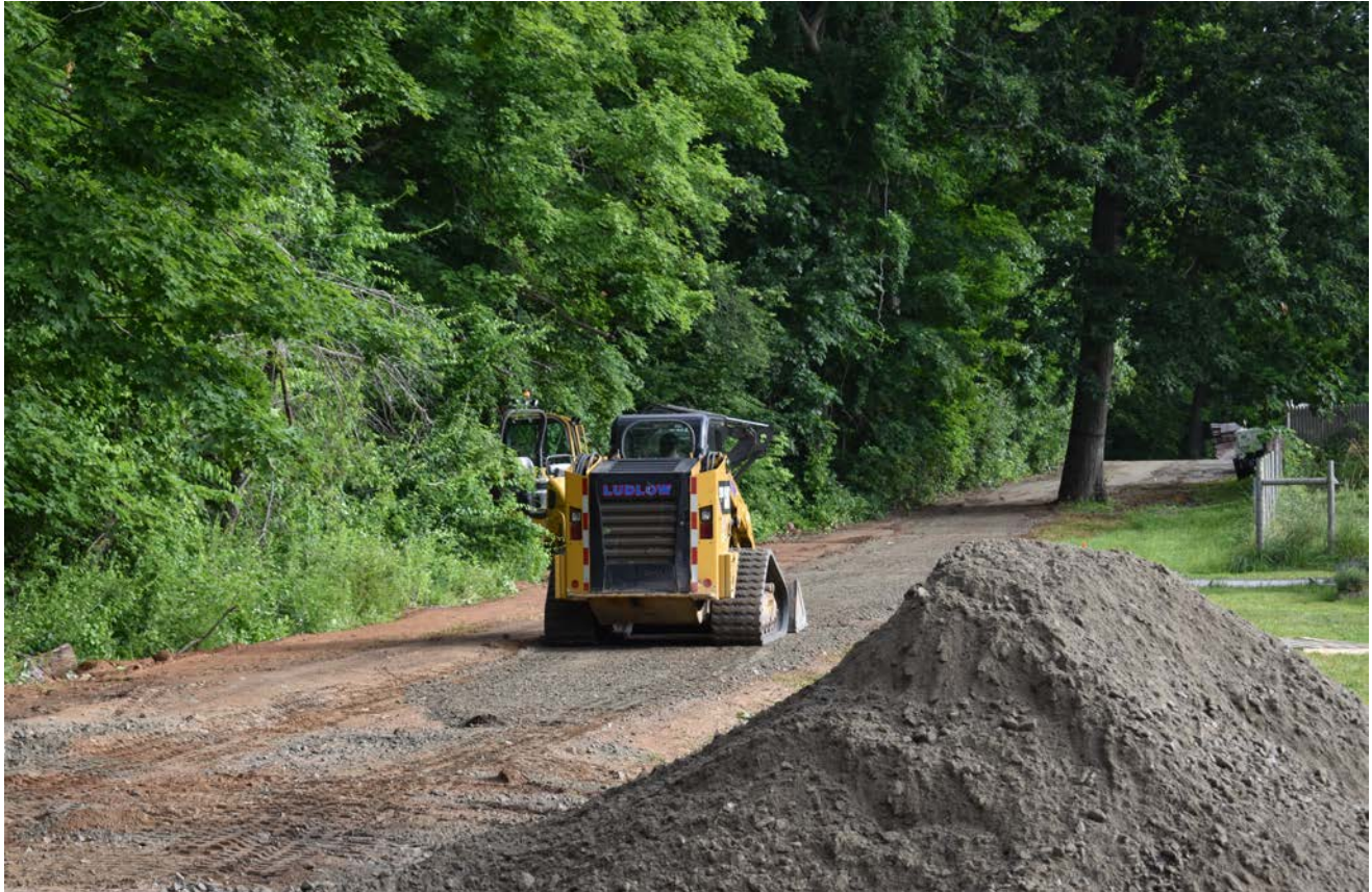
Photo 2: Ludlow skid steer operator top-dressing backfilled driveway at 114 Maiden Lane with sand. View to the northwest.
