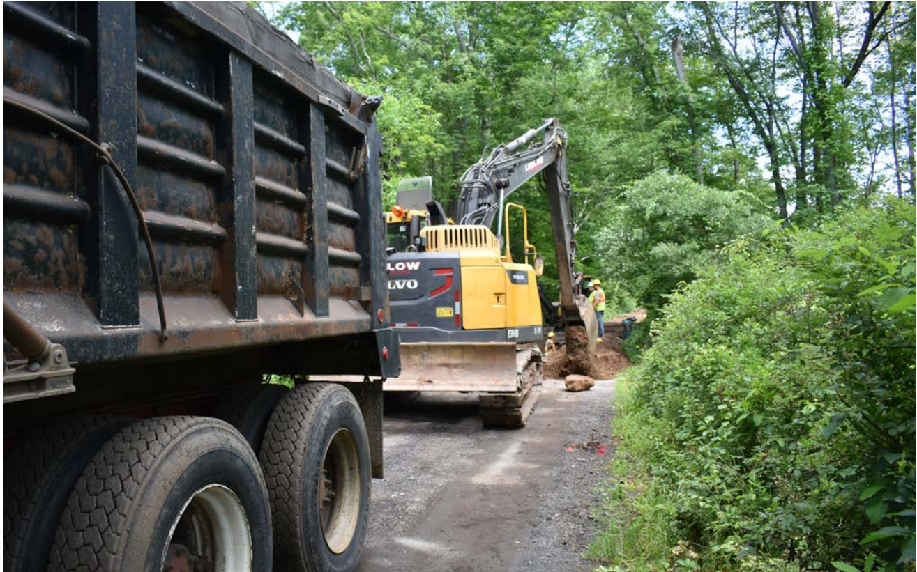
Photo 3: Water pipe trench excavation approaching brook culvert at 114 Maiden Lane. View to the north.
