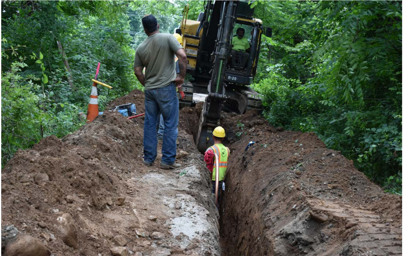
Photo 5: Ludlow extending pipe trench to brook culvert area at 114 Maiden Lane. View to the south.
