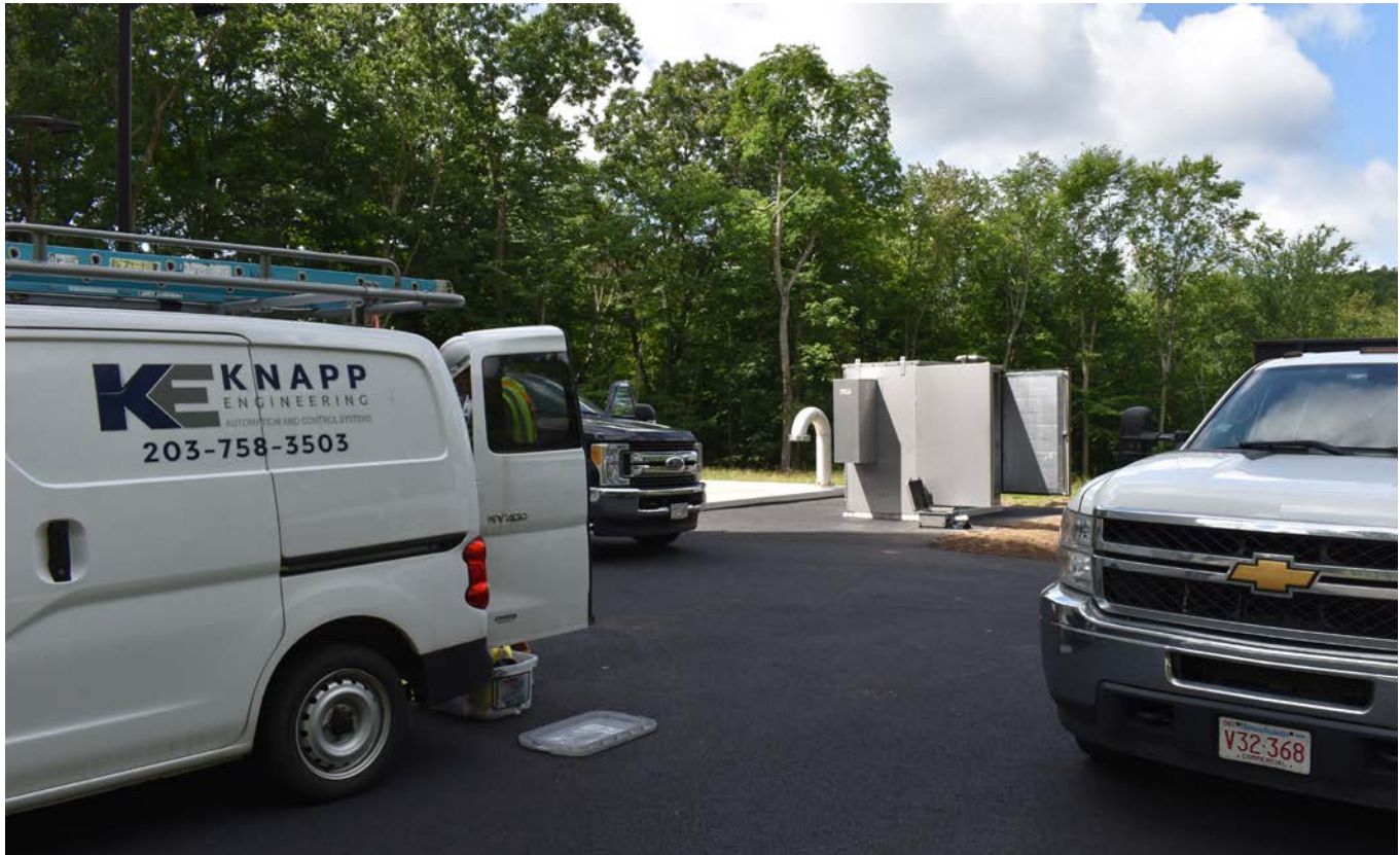
Photo 4: Knapp Engineering technicians preparing to adjust the control system antenna at the water tank site off Talcott Ridge Drive. View to the southwest.
