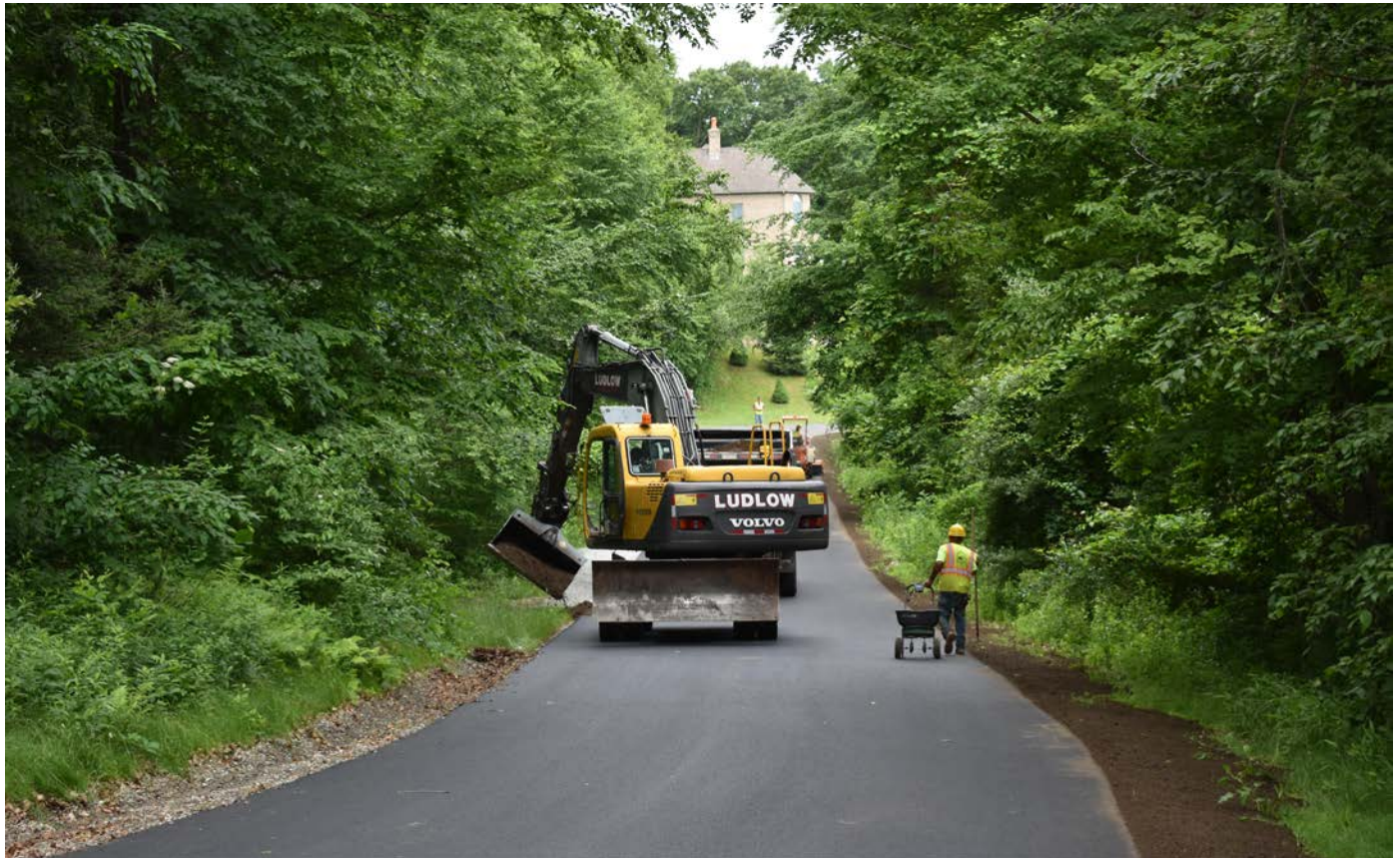
Photo 4: Ludlow road crew placing loam and seed off the sides of Shared Access Driveway. View to the west.
