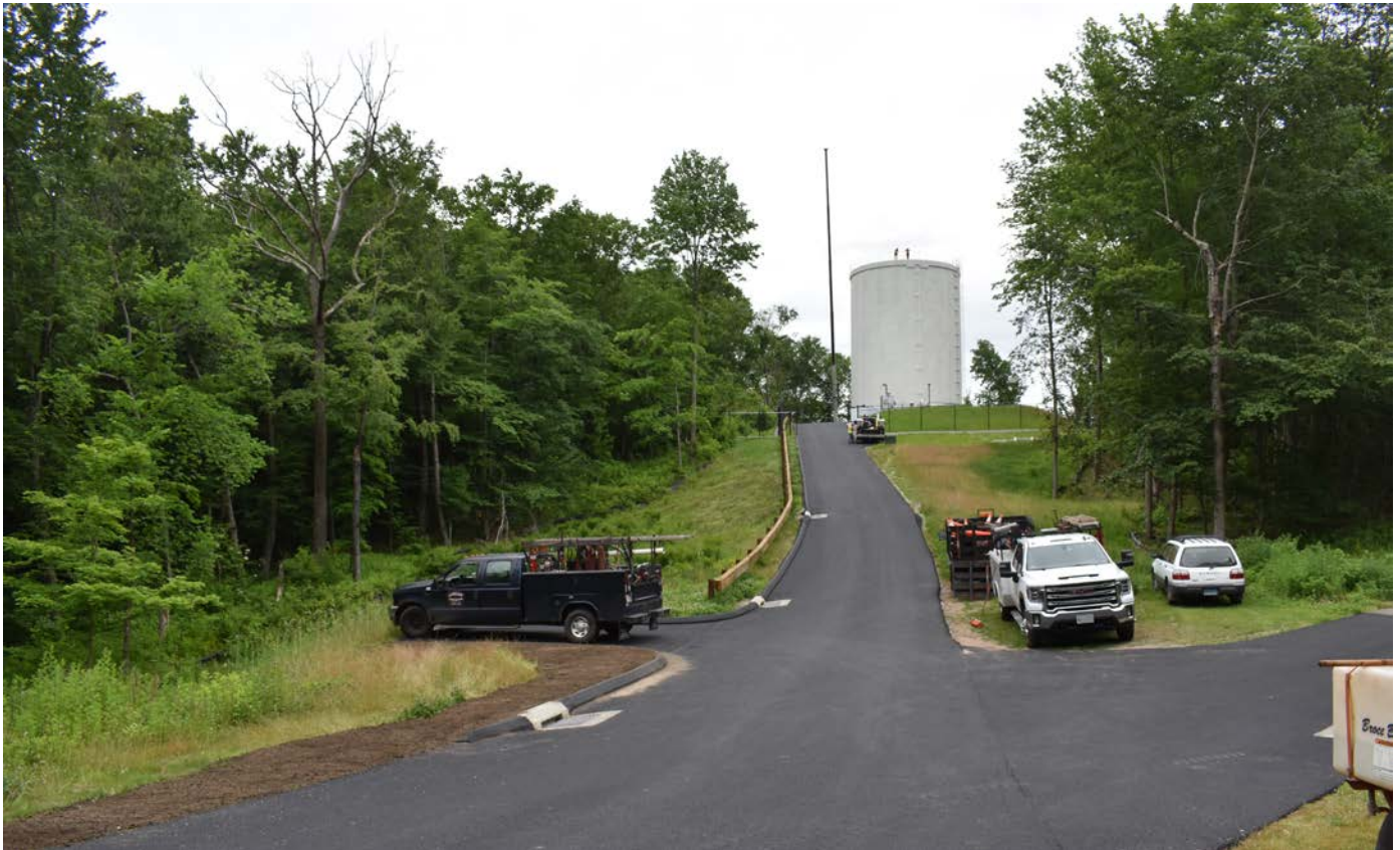
Photo 2: Tank access Driveway off Talcott Ridge Drive. Crane boom has been assembled adjacent to tank. View to the east.
