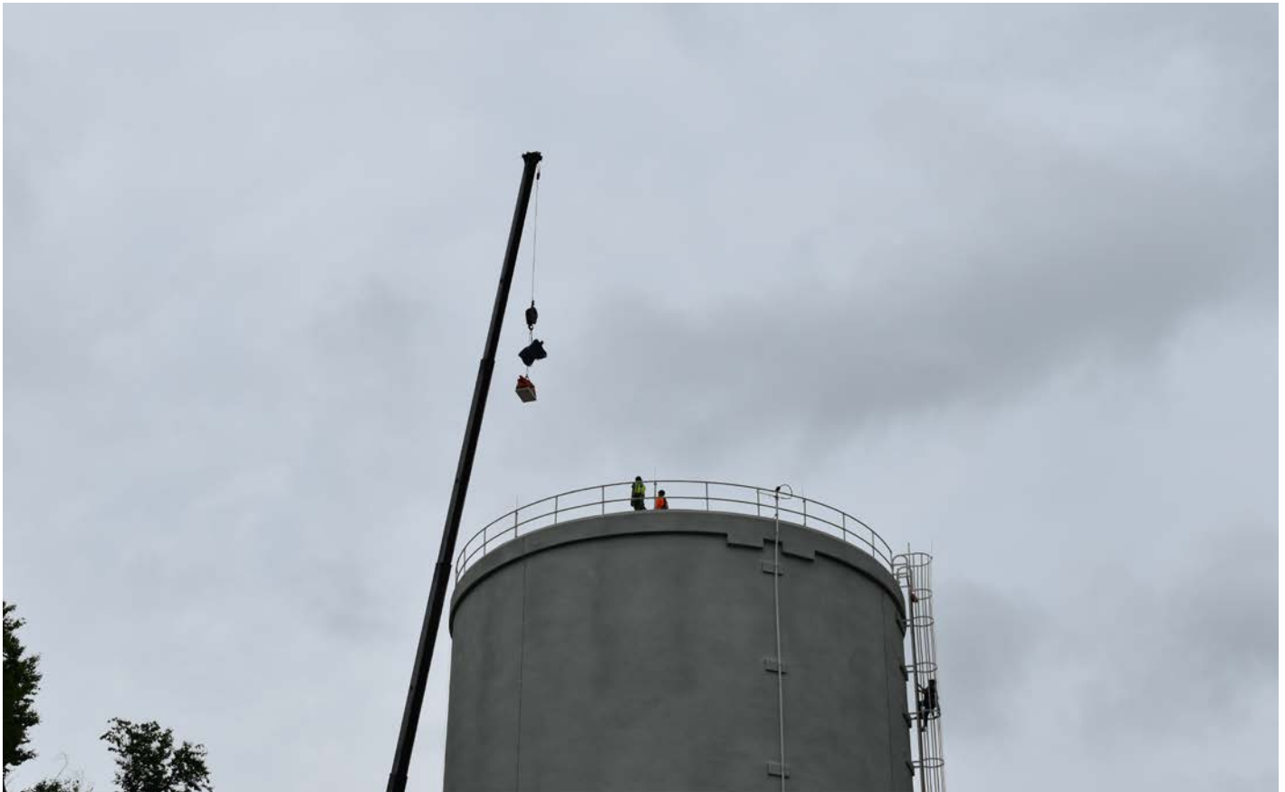
Photo 3: Equipment and supplies being delivered to workers on tank roof. View to the east.
