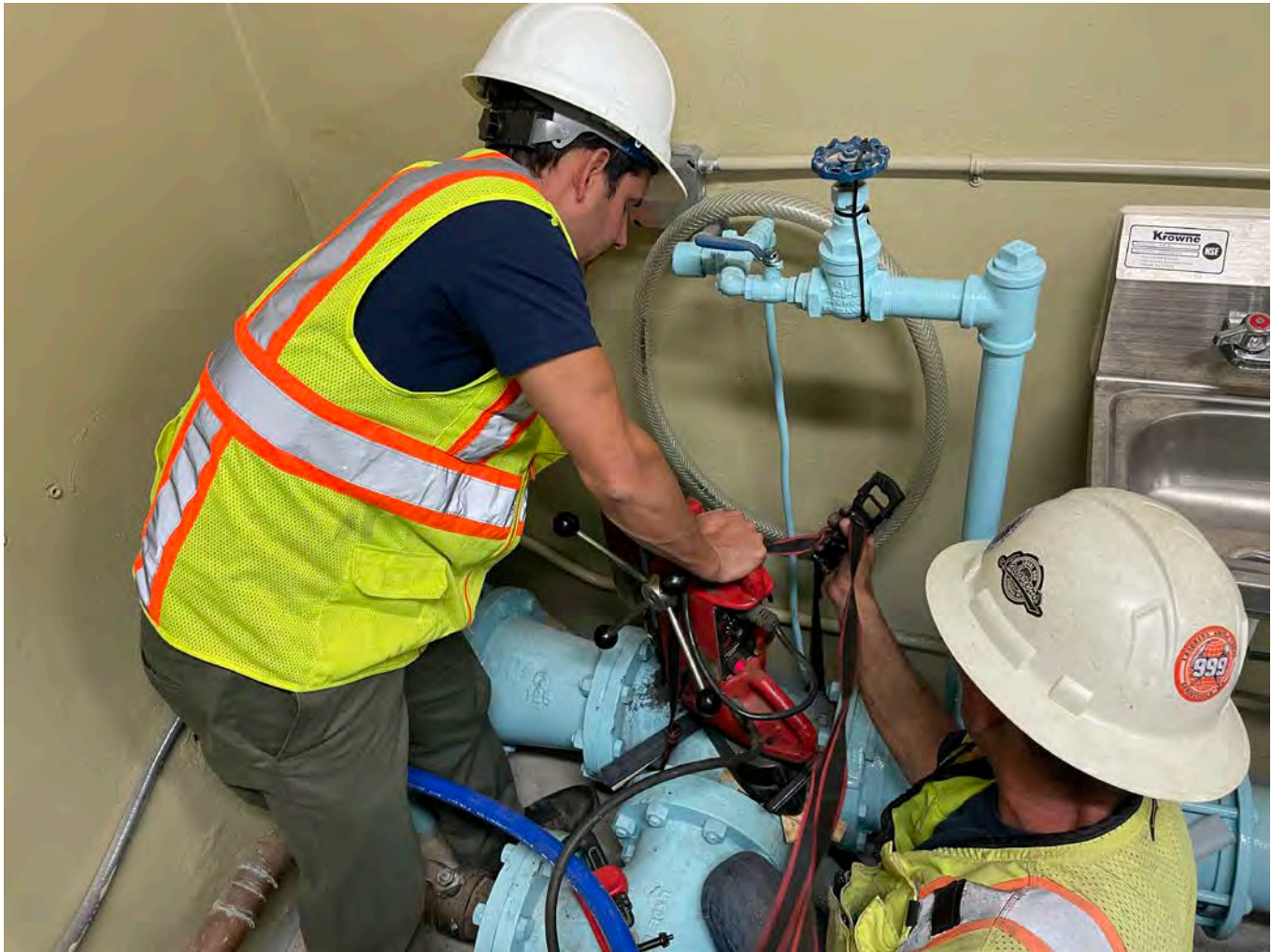
Picture 4: Ludlow setting up to tap a 6" DIP TEE located at the southwest corner of the Long Hill Pump Station in Middletown. The tap site will be used for chlorine injection.
