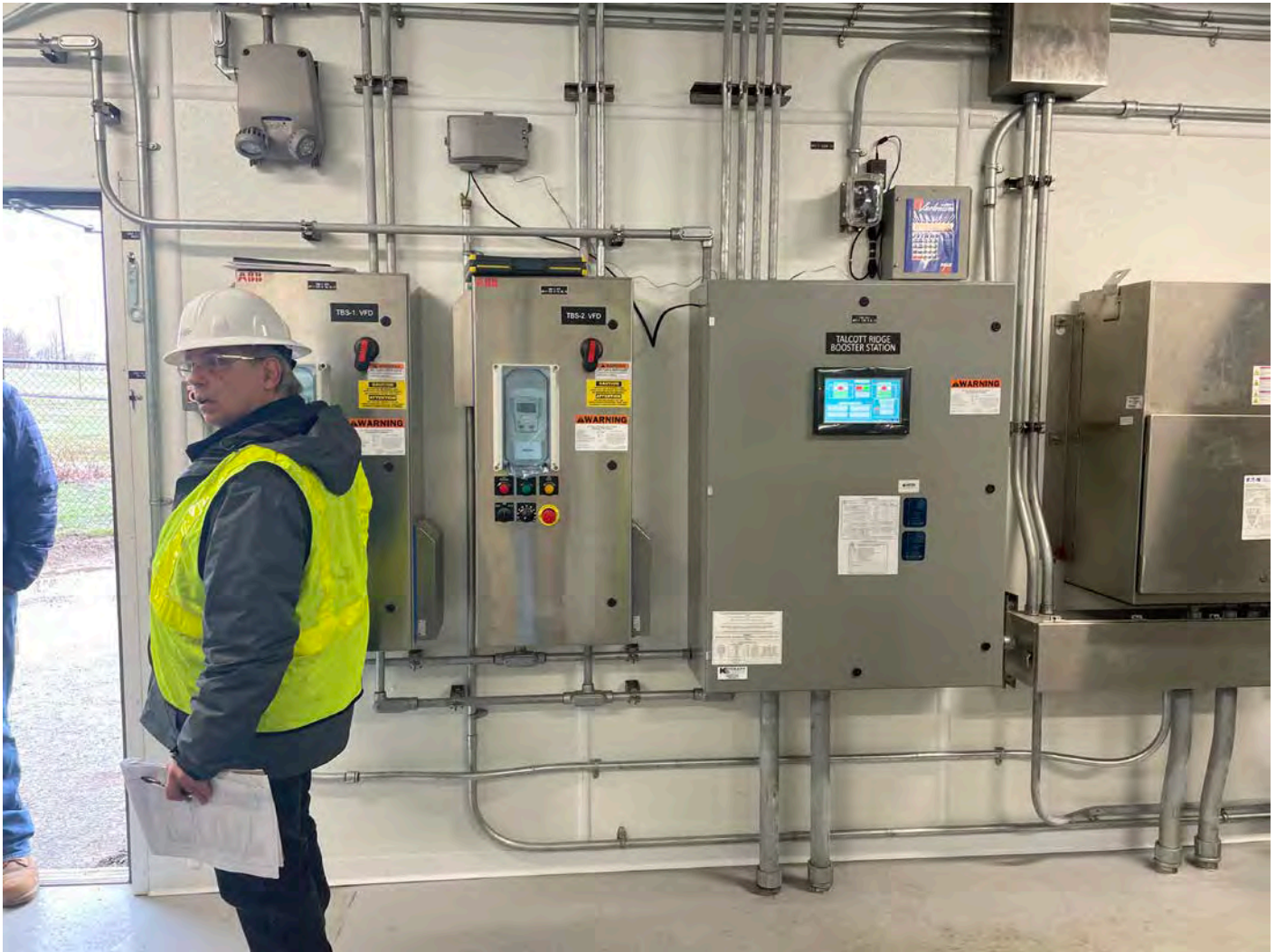
Picture 2: Variable frequency drives (left) and control panel (center) located on the north side of the booster station located on S. Main Street in Middletown. View to the north.
