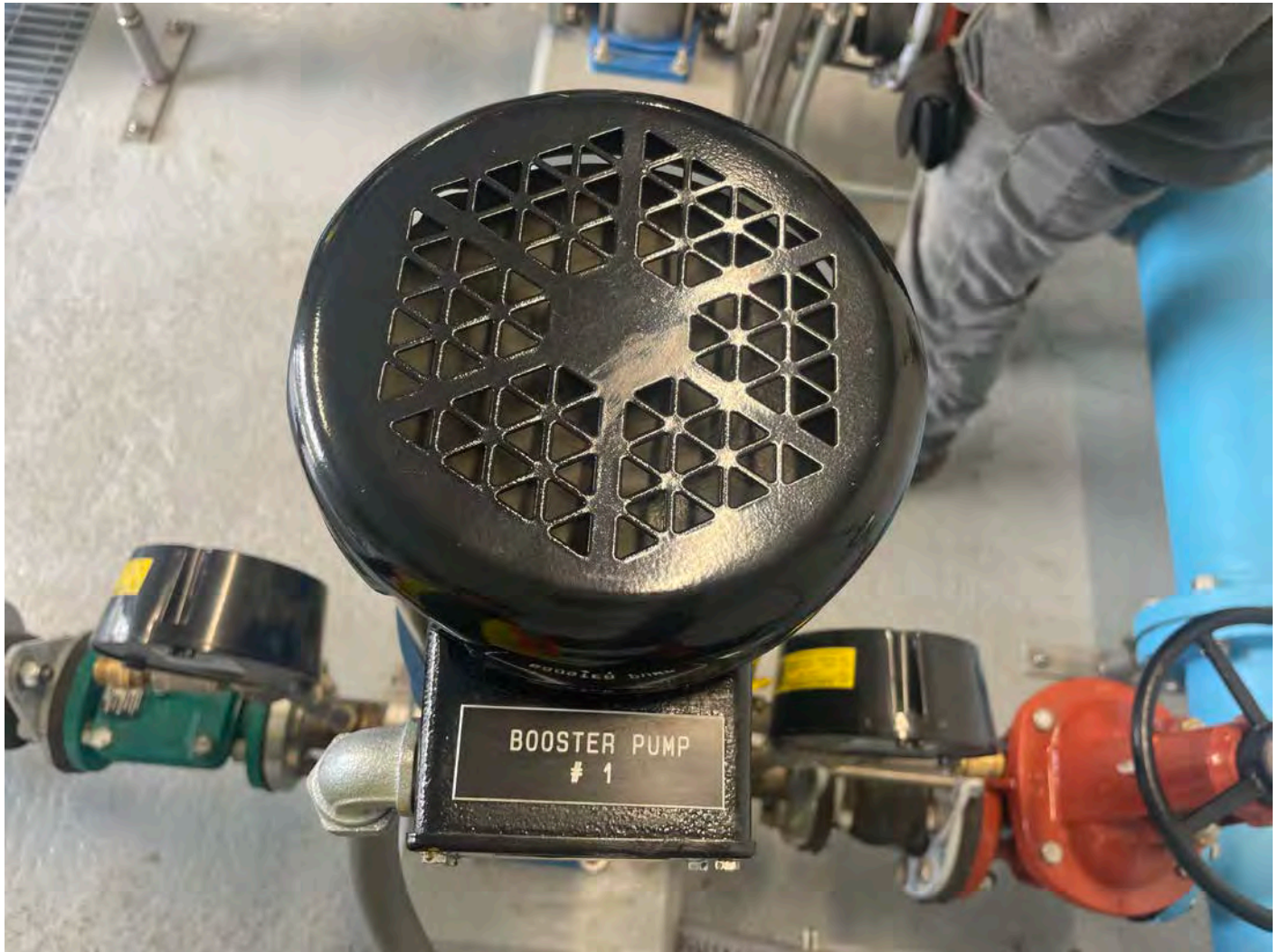
Picture 6: Booster Pump #1, which was spinning in the opposite direction due to some wiring issues. This problem was solved before the project team left the booster station for the day.
