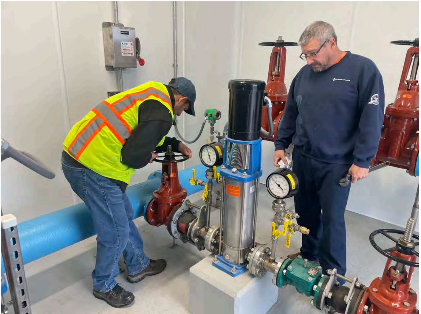
Picture 1: Ludlow opening water line valve inside of the booster station located on S. Main Street in Middletown. View to the southwest.
