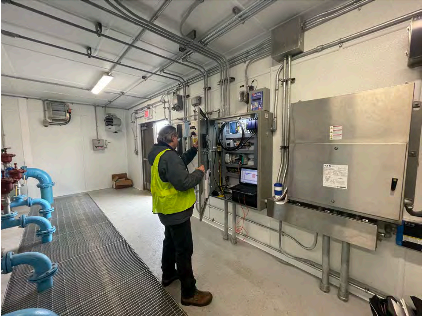
Picture 7: Knapp Engineering working on the control panel located on the north side of the booster station located on S. Main Street in Middletown. View to the northwest.
