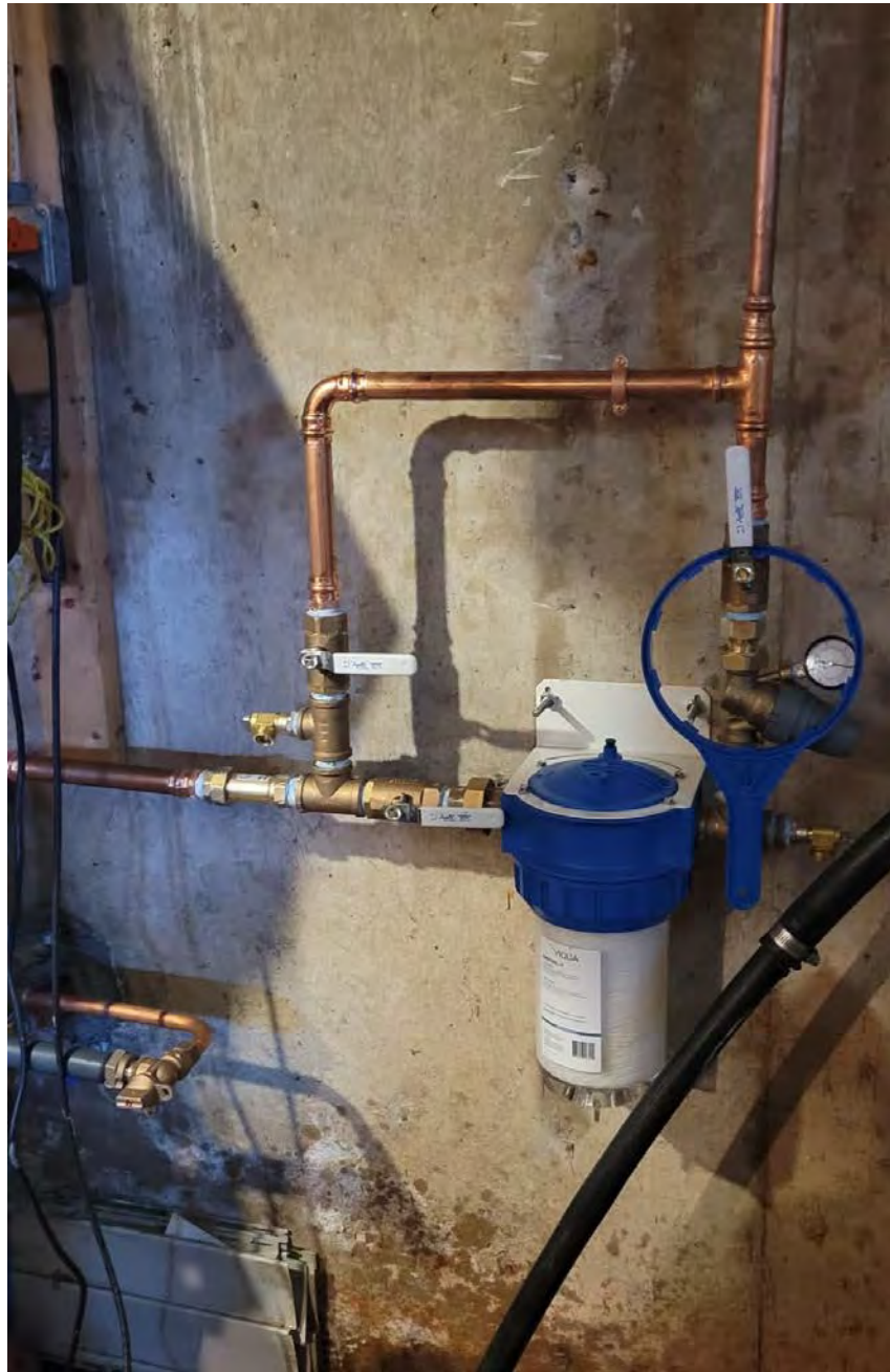
Picture 1: Final water system components that were installed at the 187 Maple Avenue, Durham, residence by Fazzino Plumbing.
