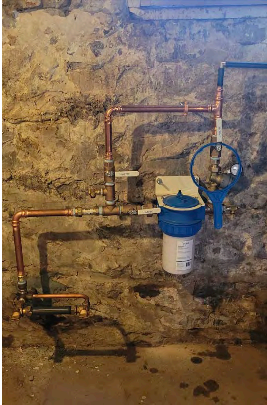
Picture 2: Final water system components that were installed at the 158 Maple Avenue, Durham, residence by Fazzino Plumbing.
