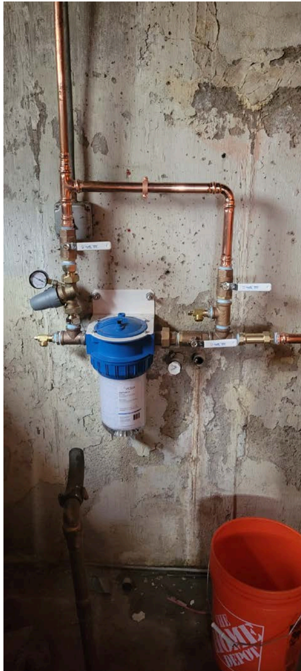
Picture 1: Final water system components that were installed at the 188 Maple Avenue, Durham, residence by Fazzino Plumbing.
