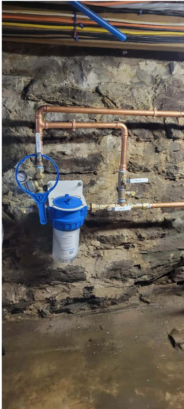
Picture 3: Final water system components installed at the 123 Maiden Lane, Durham, residence by Fazzino Plumbing.
