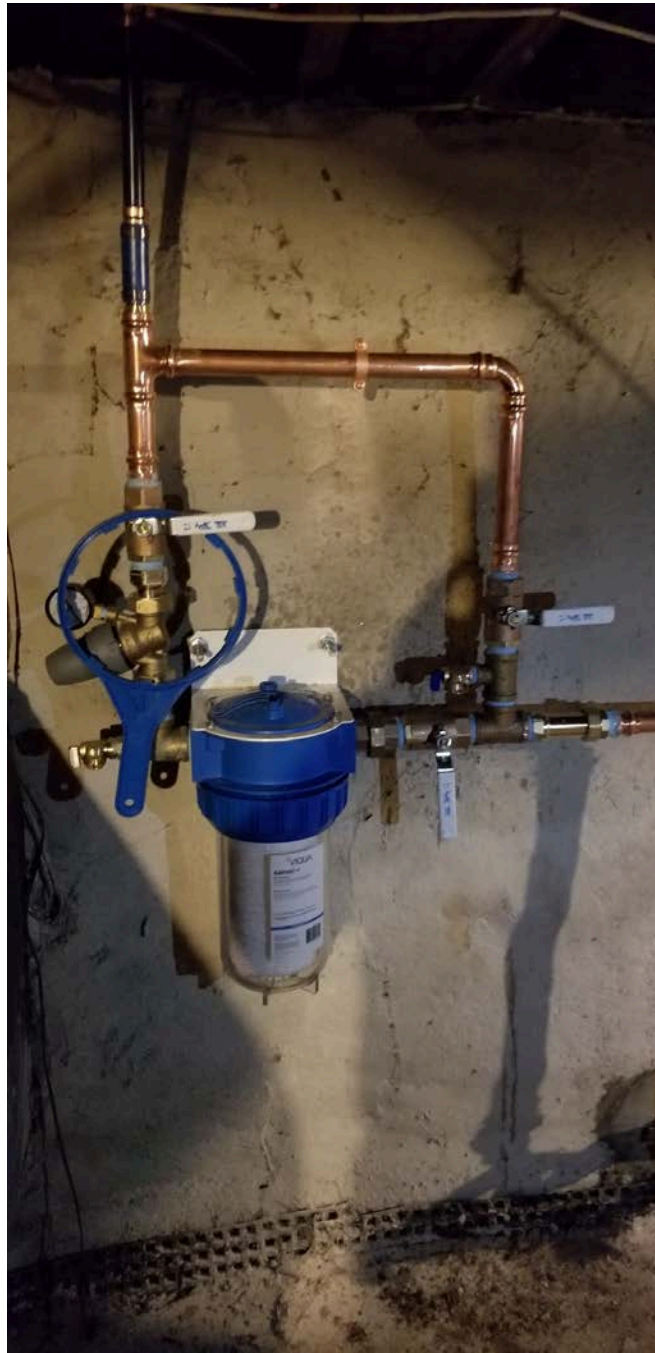
Picture 2: Final water system components that were installed at the 254 Maple Avenue, Durham, residence by Fazzino Plumbing.
