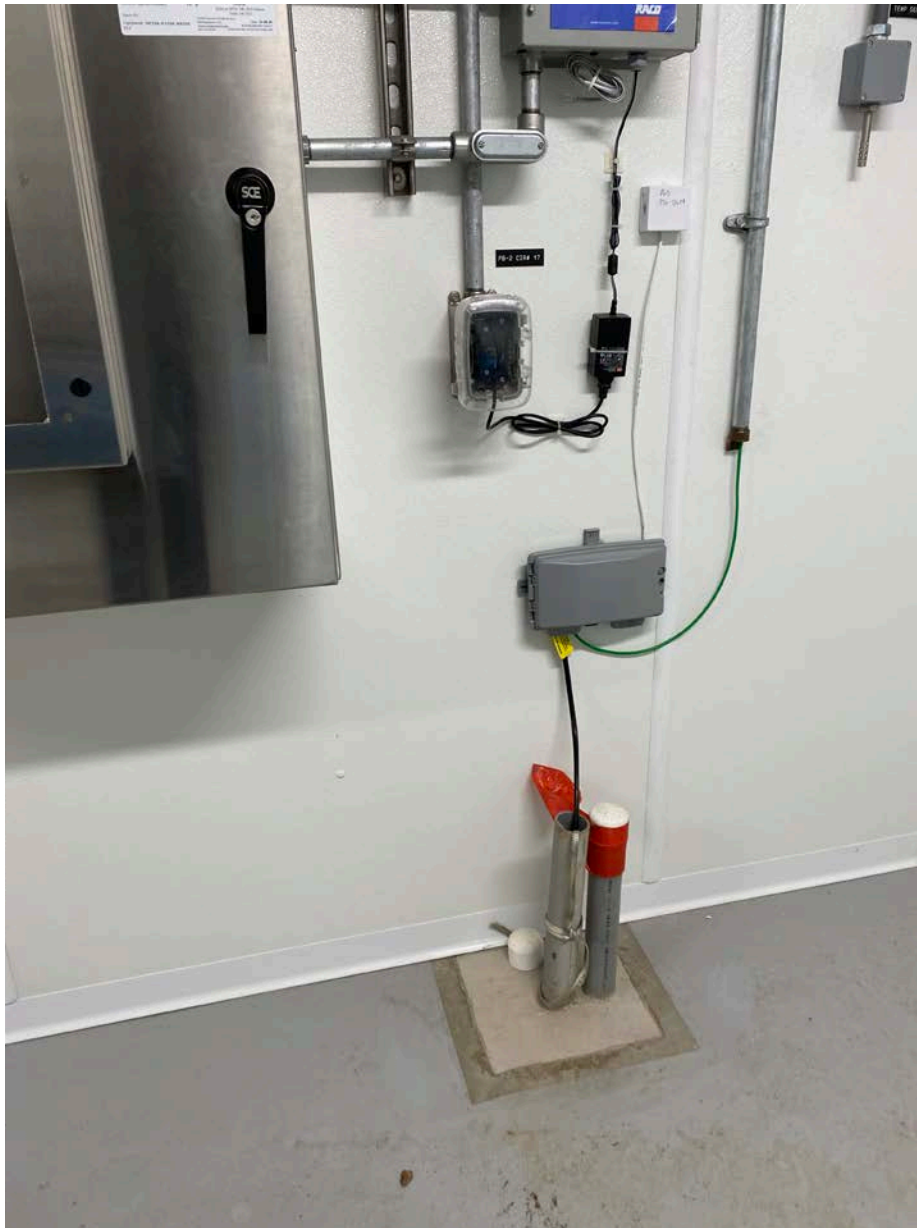
Picture 4: A & R Electric wires the telephone demarcation box to the ground bar in the Booster Station.
