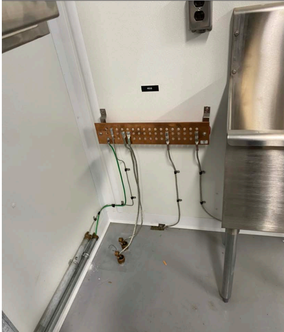
Picture 3: A & R Electric wires the telephone demarcation box to the ground bar in the Booster Station.
