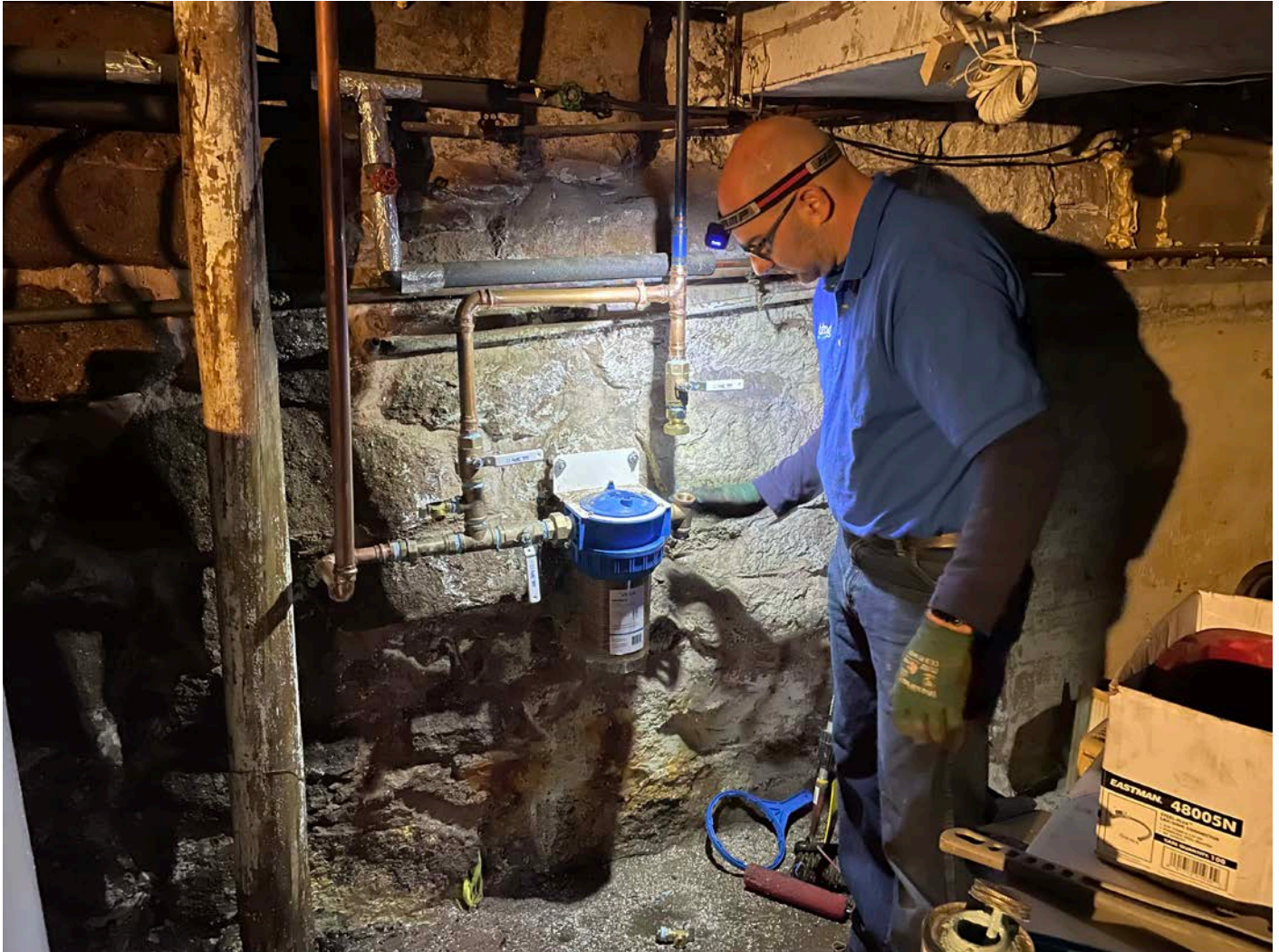
Picture 5: Fazzino Plumbing replacing brass tee fittings at the 312 Main Street, Durham, residence.
