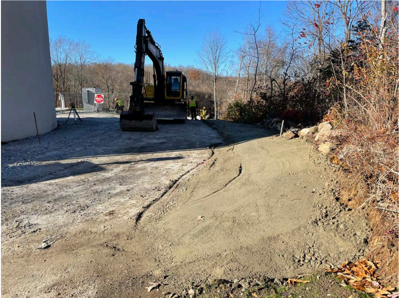
Picture 1: 1.25"-minus gravel that Ludlow has placed and compacted on the north side of the water tank located east of the Shared Access Driveway in Middletown. View to the west.
