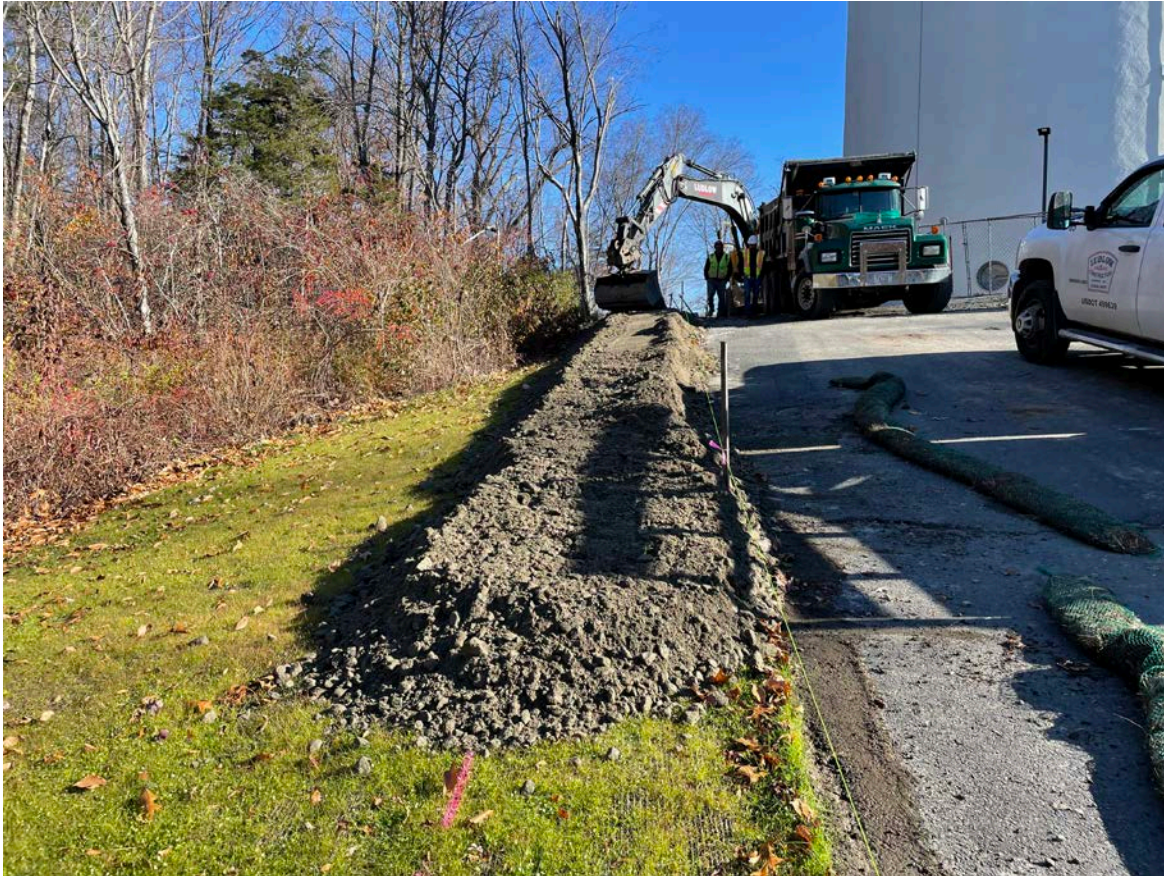
Picture 3: 1.25"-minus gravel that Ludlow has placed between Stations 10+50 and 11+75 on the north side of the Shared Access Driveway in Middletown. View to the east.
