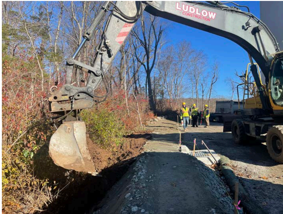
Picture 4: Ludlow placing loam over the 1.25"-minus gravel that they placed and compacted on the north side of the water tank and between Stations 10+50 and 11+75. View to the east.
