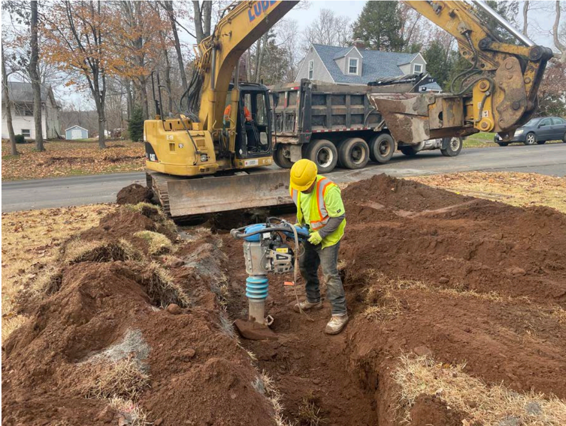
Picture 3: Ludlow compacting a 1' lift of native fill after having installed a 1" copper water line at the 235 Maple Avenue property. View to the west.
