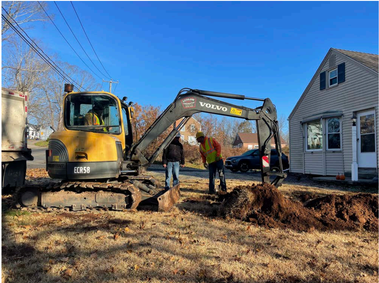
Picture 1: Ludlow excavating on the west side of the 235 Maple Avenue property for the installation of a 1” copper water service line. View to the northeast.
