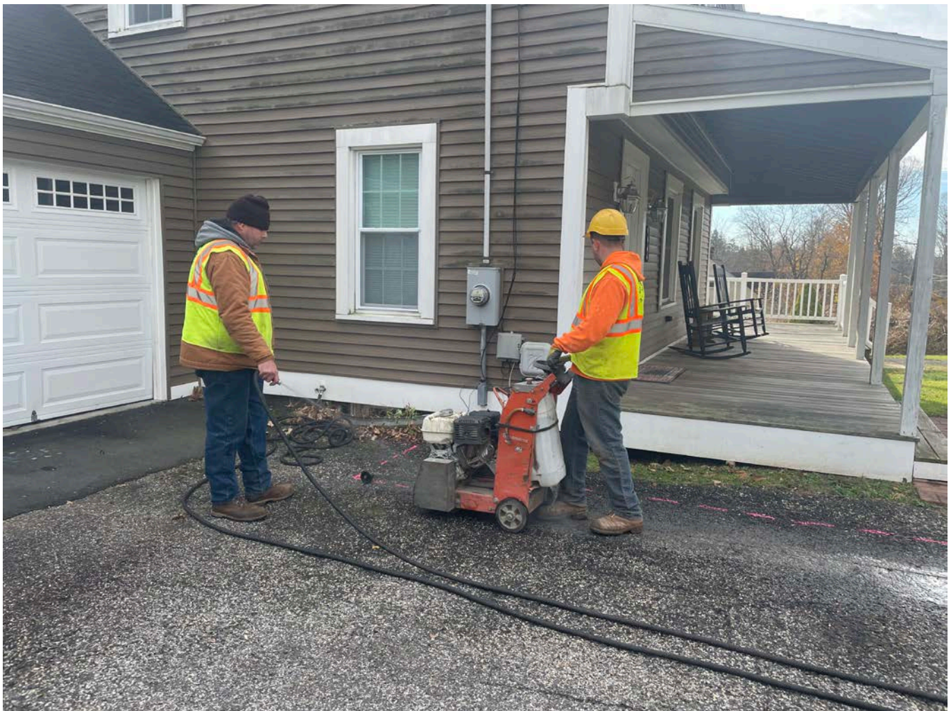
Picture 2: Ludlow saw cutting asphalt on the driveway of the 245 Maple Avenue property for the installation of a 1" copper water service line. View to the south.
