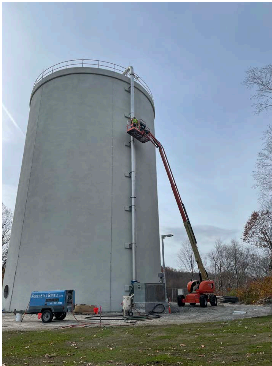
Picture 5: Keltic Painting in the process of painting the 12" air duct located on the northeast side of the water tank located east of the Shared Access Driveway in Middletown. View to the west.
