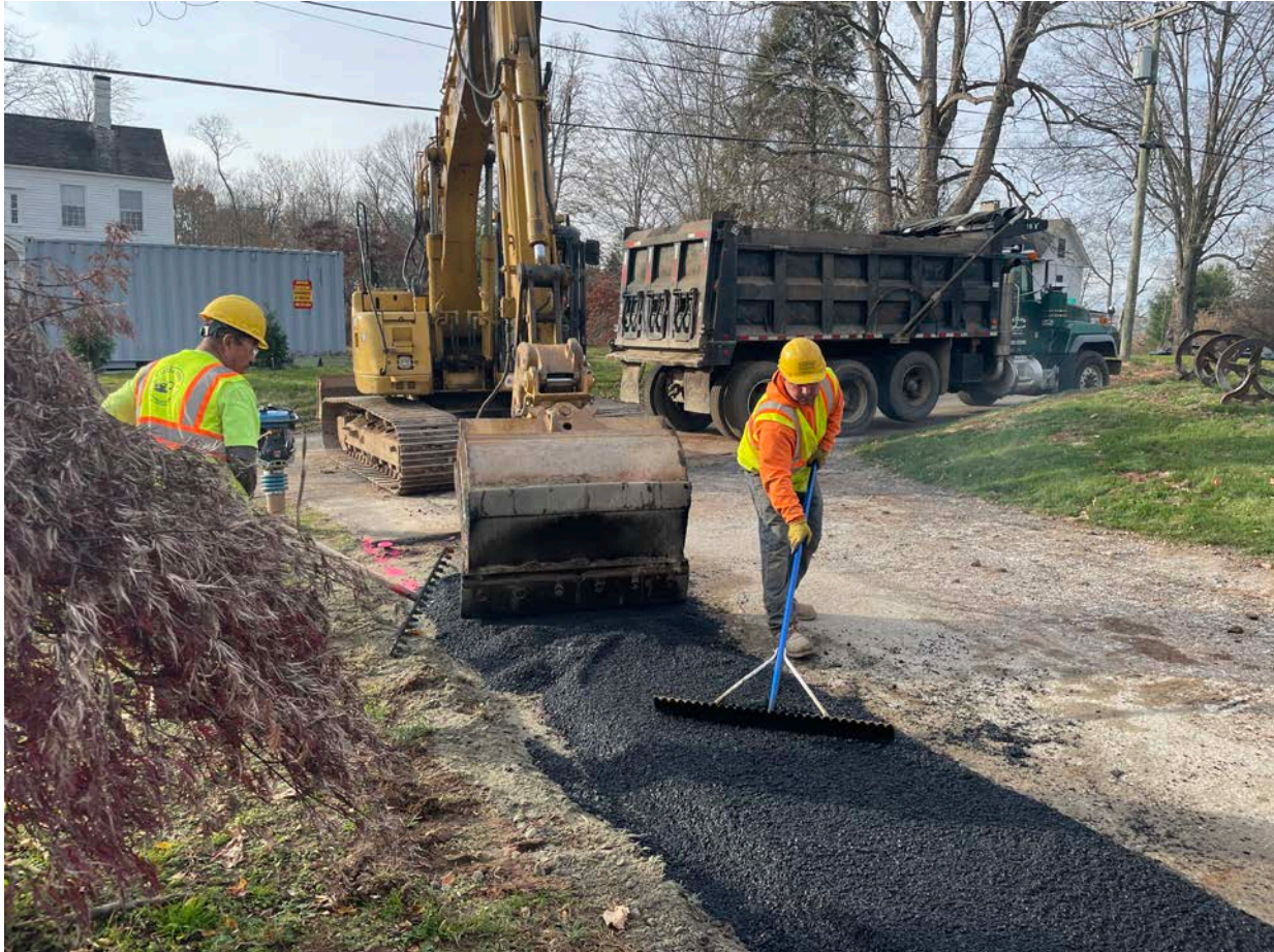
Picture 6: Ludlow placing asphalt over the trench footprint at the 245 Maple Avenue property. View to the west.
