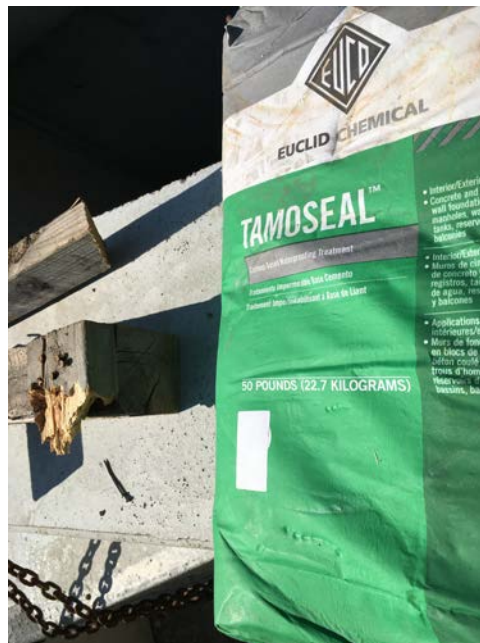
Picture 4: Tamoseal powder mixed with Arco (no pic - not yet on site so). First sealing coat for cap of tank.
