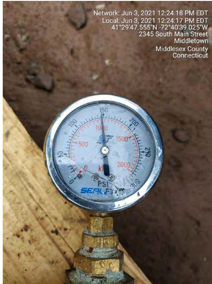
Picture 7: Final pressure of the pressure test that Ludlow performed today on the section of 16” DIP that Ludlow previously installed on the south side of the water meter vault footprint.
