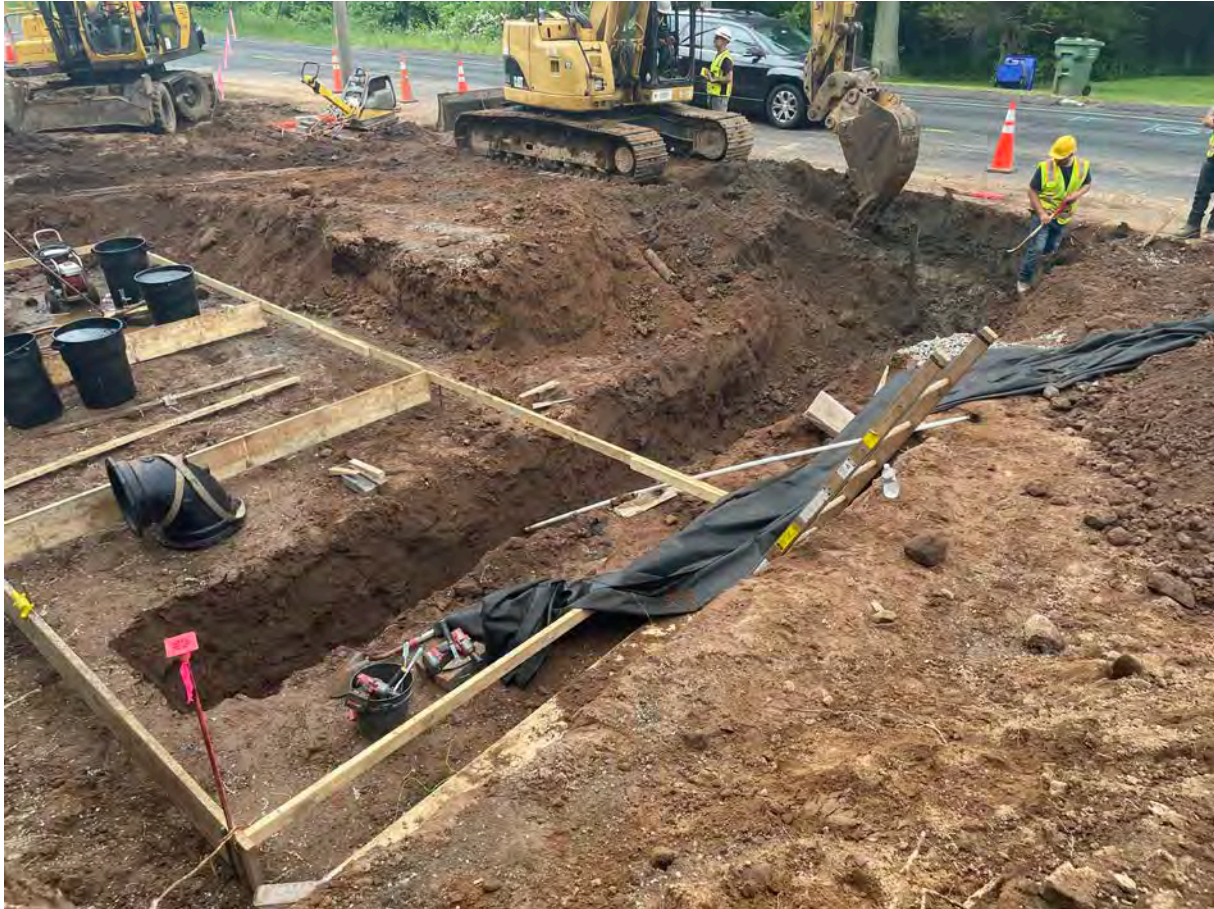
Picture 1: Ludlow excavating at and east of Station 801+00 for the installation of 16" DIP. View to the southwest.
