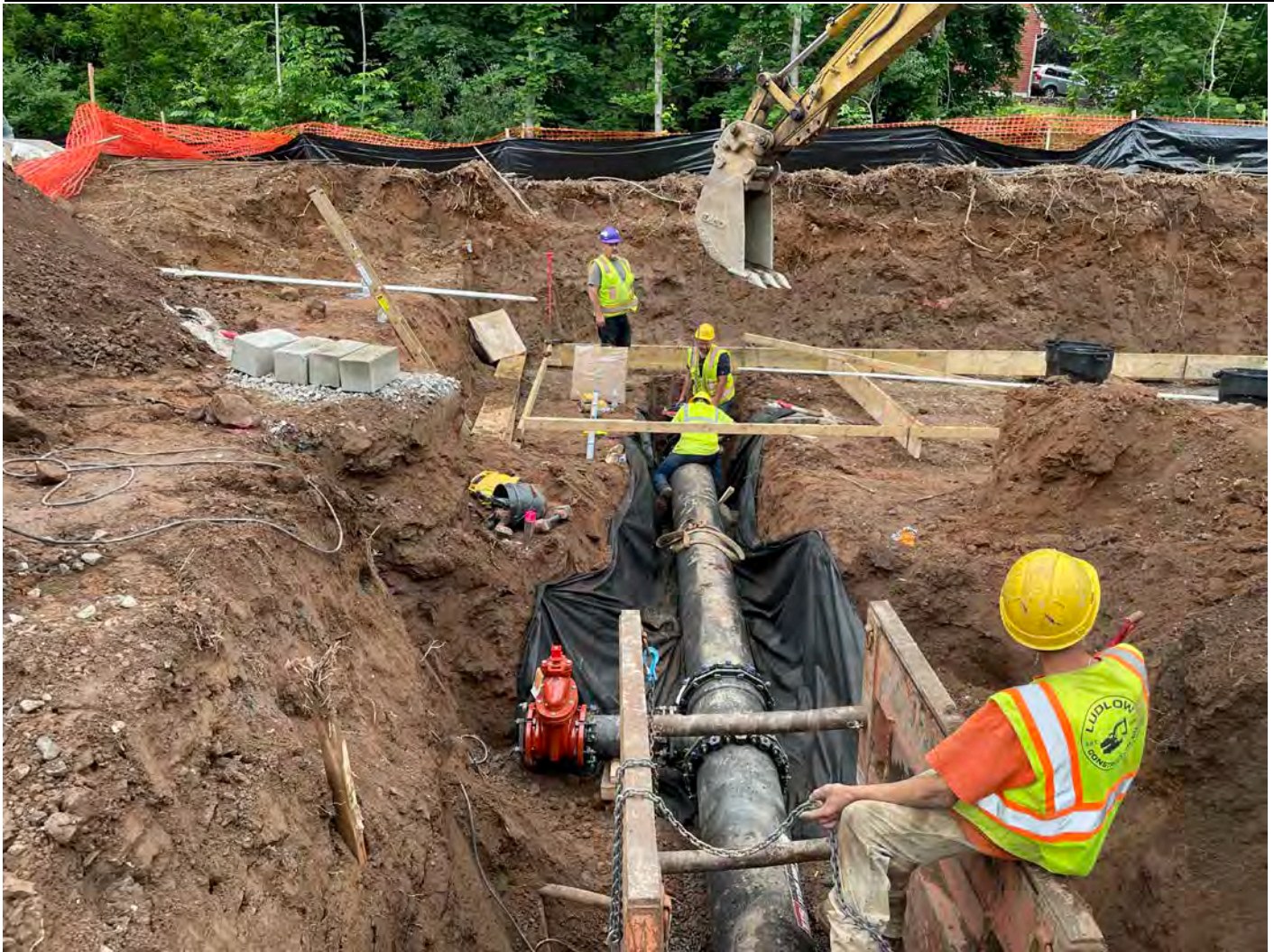
Picture 5: View of Ludlow installing 16" DIP east of Station 800+00 at the water meter vault work zone located at ~Station 124+80. View to the east.
