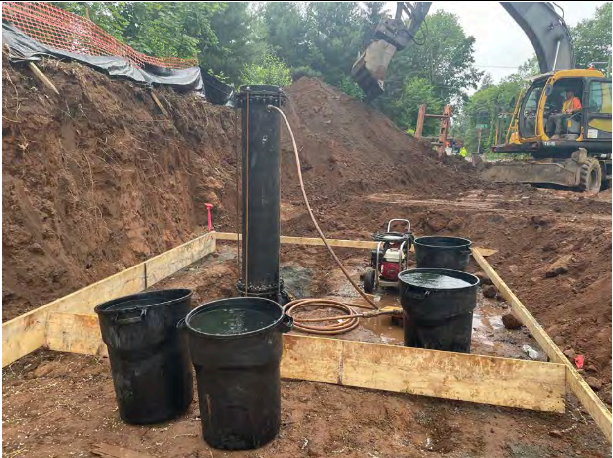
Picture 2: 16" Ludlow conducting a pressure test on the 16" DIP they previously installed on the south side of the water meter vault footprint. View to the south.
