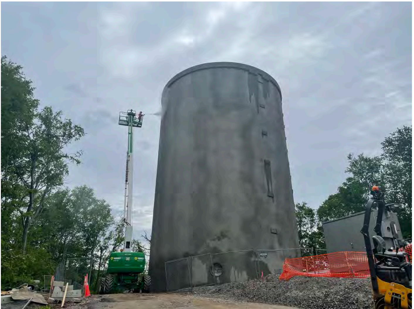
Picture 3: DN Tanks pressure washing the exterior of the water tank located east of the Shared Access Driveway in Middletown as they prepare to place the final coating on the tank. View to the east.
