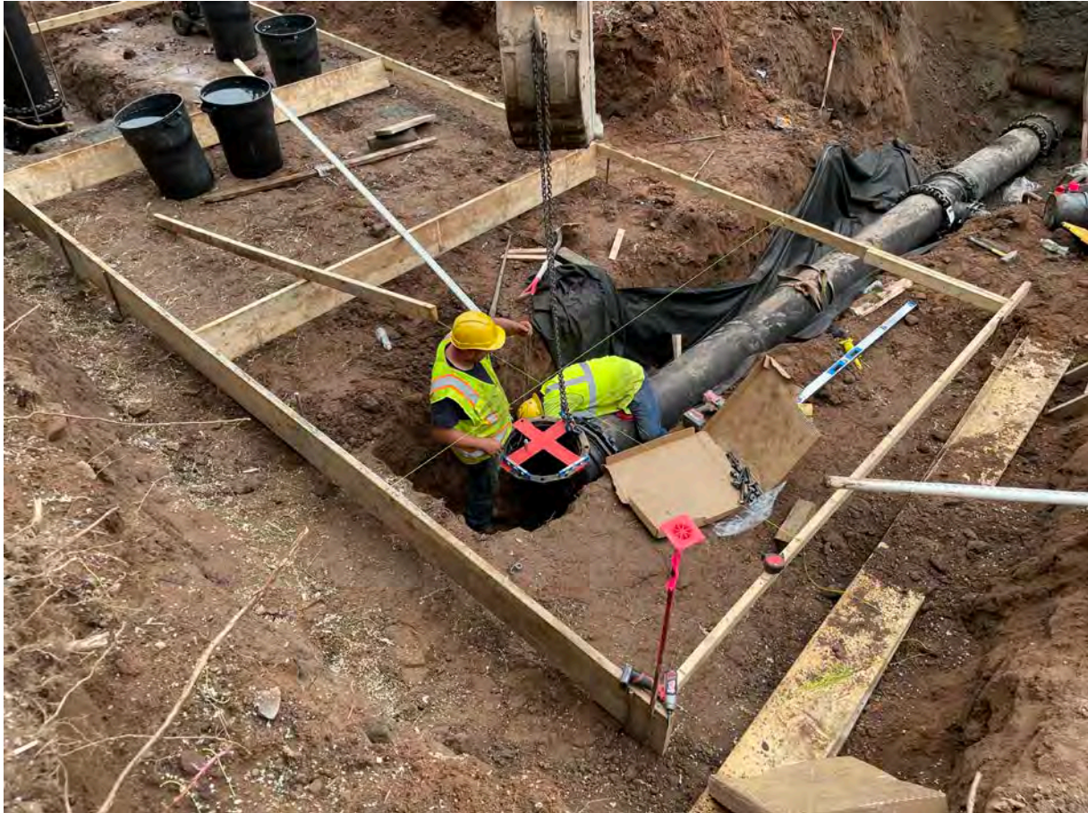
Picture 6: Ludlow installing a 16" DIP 90° bend at the northeast corner of the water meter vault footprint located at ~Station 124+80. View to the southwest.
