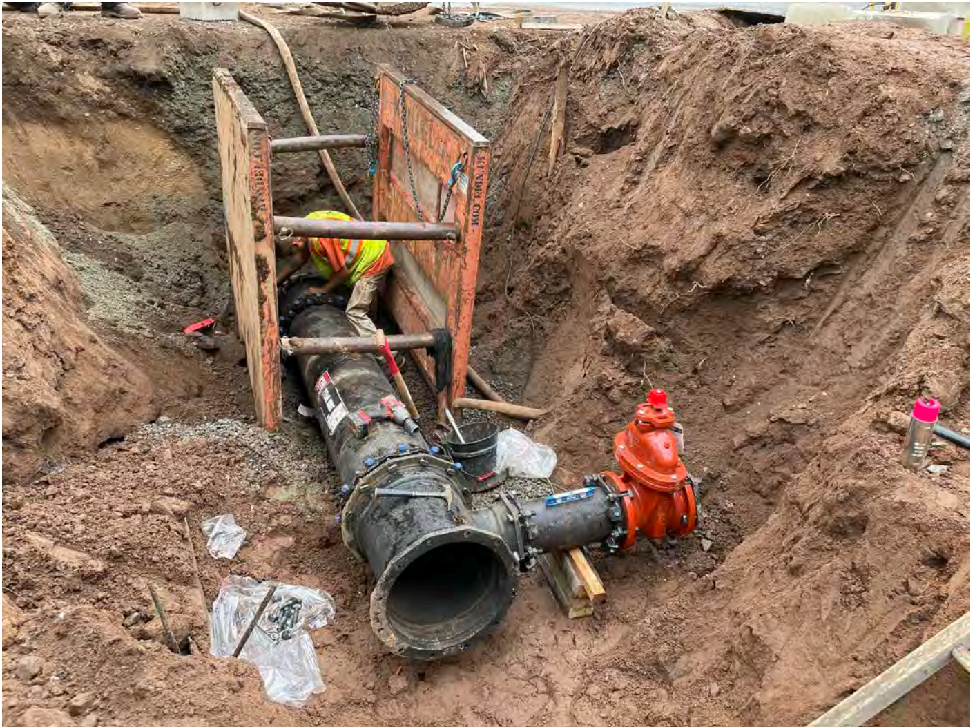
Picture 4: Ludlow installing 16" DIP with a 16x16x8 M.J. C.L.D.I. TEE and an M.J. 8" gate valve. View to the west.
