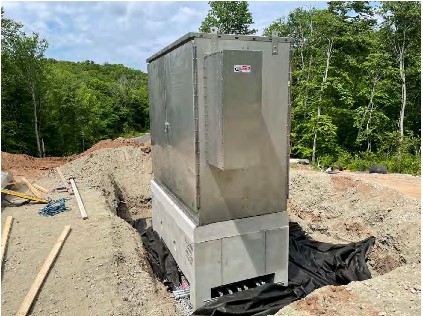
Picture 3: The electrical enclosure that Ludlow just placed on the north side of the altitude vault. View to the west.
