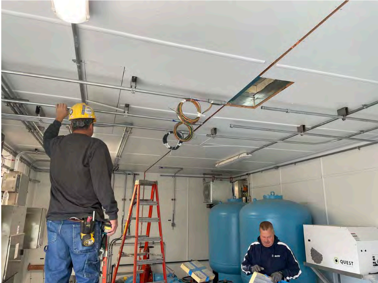
Picture 1: United Concrete installing wiring and wiring conduits on the inside of the booster station located at Station 750+63 in Middletown. View to the east.
