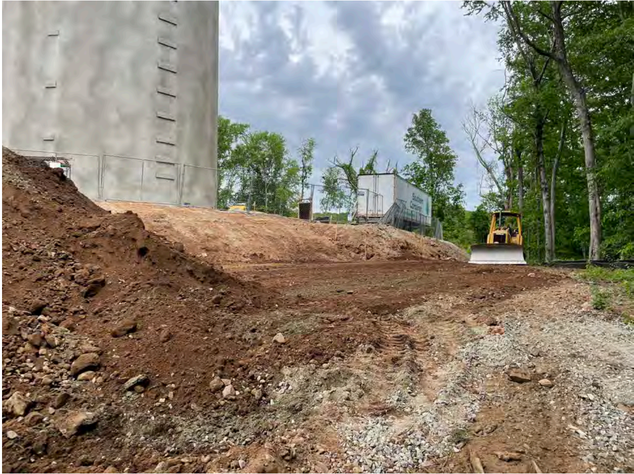
Picture 8: Ludlow grading fill at the toe of slope on the southwest side of the water tank work zone located east of the Shared Access Driveway in Middletown. View to the east.
