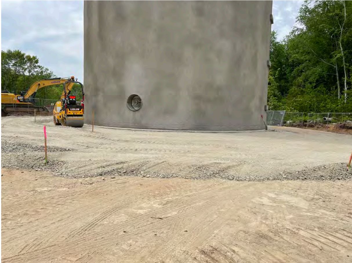
Picture 6: Ludlow compacting fill in the southeast side of the base of the water tank located east of the Shared Access Driveway in Middletown. View to the west.
