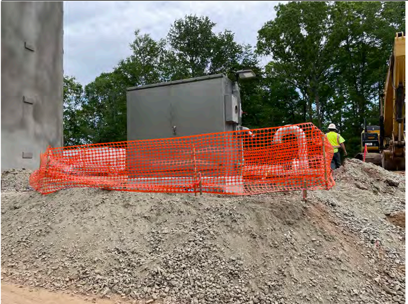
Picture 5: The electrical enclosure that Ludlow just placed on the north side of the altitude valve vault, with snow fence placed around it for security. View to the south.
