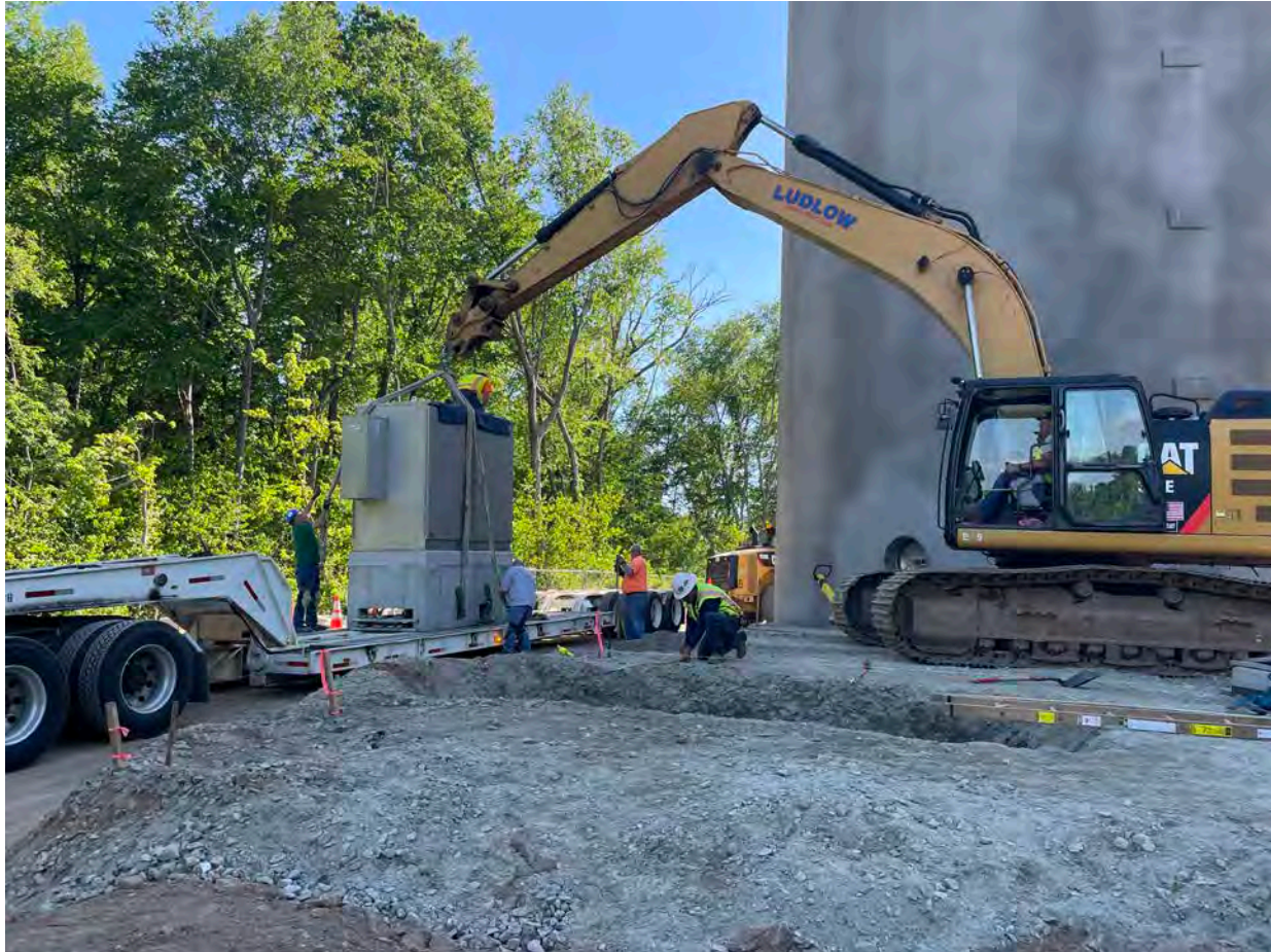
Picture 2: Ludlow preparing to lift the electrical enclosure into place on the north side of the altitude valve vault. View to the northeast.
