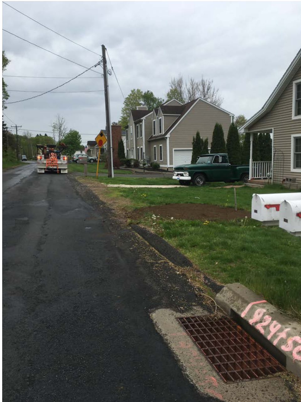
Picture 4: View to south. Ludlow restores water service trenches in response to complaints from homeowners at 166 Maple St. (foreground) and 172 Maple Street (in background).
