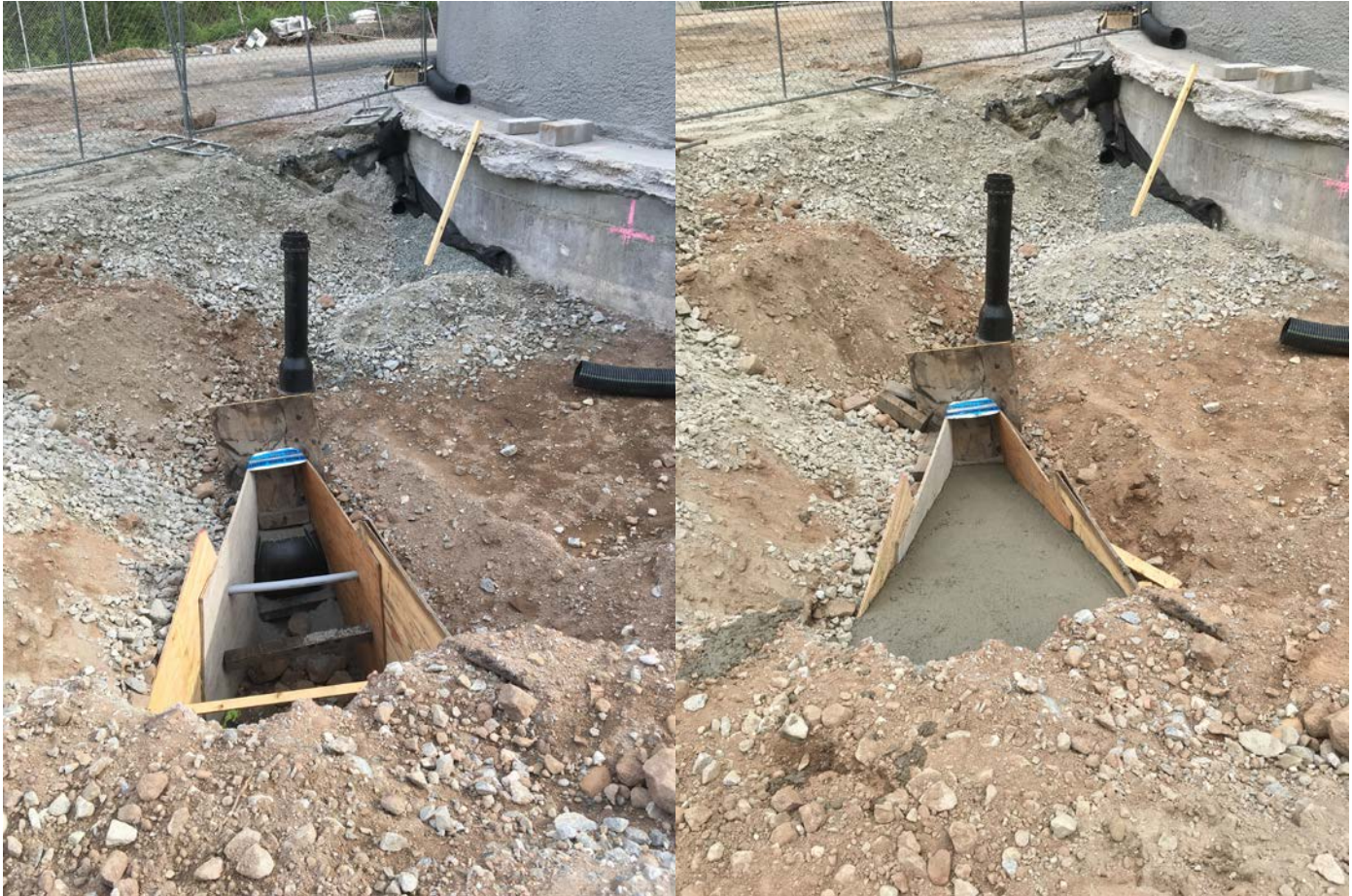
Picture 2: Thrust block form and pre and post concrete placement. Tank driveway is to the top left of the photo.
