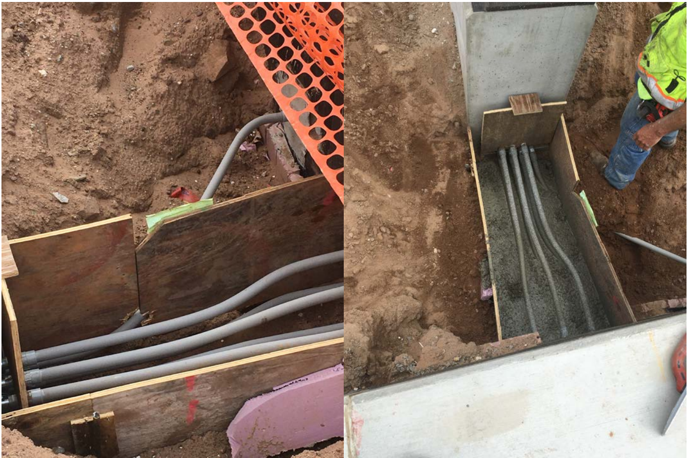
Picture 3: View of the form at the PRV vault near Routes 17 & 147. Note that Ludlow ran short of concrete and will need to complete the pour next week. The line not inside the form is the grounding line.
