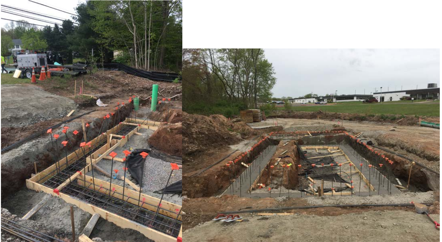
Picture 1: View of the booster station footprint before and after concrete footing is placed. Ludlow placed the concrete and positioned the rebar within the concrete to the proper configuration for the foundation walls of the booster station located at Station 750+63 South Main Street in Middletown. Views are to south and to the west.
