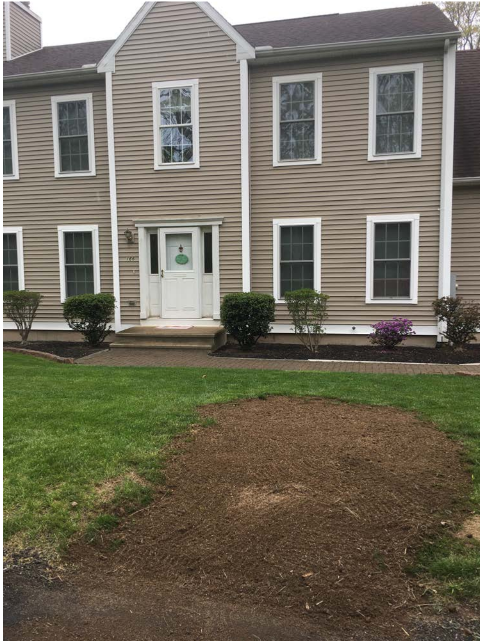
Picture 5: View to west of 172 Maple Street lawn repair. Water service trench settling was not acceptable to homeowner.
