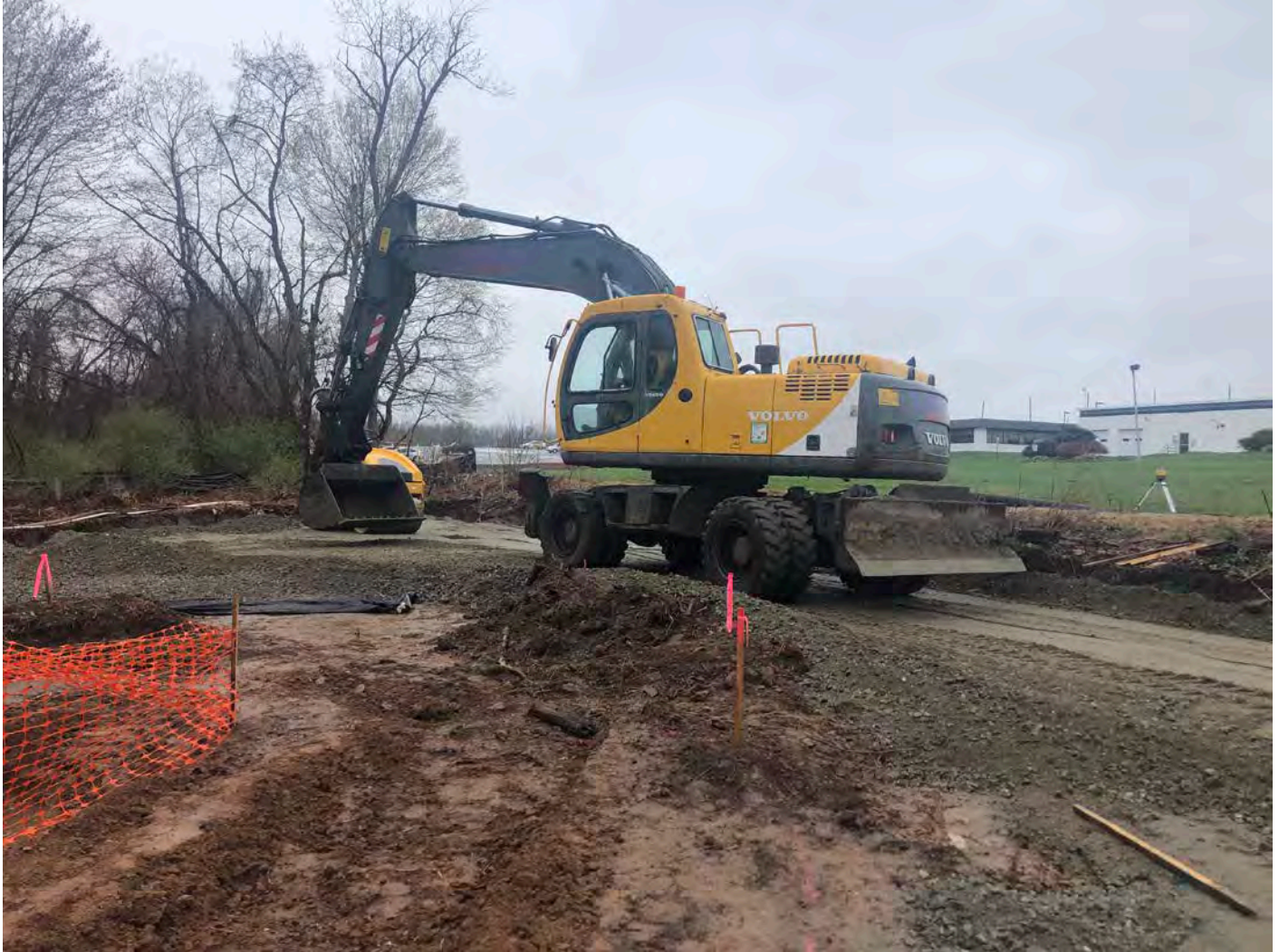
Picture 5: Ludlow grading 1.25” gravel as they construct the bituminous concrete driveway at the booster station located at Station 750+63 in Middletown. View to the west.
