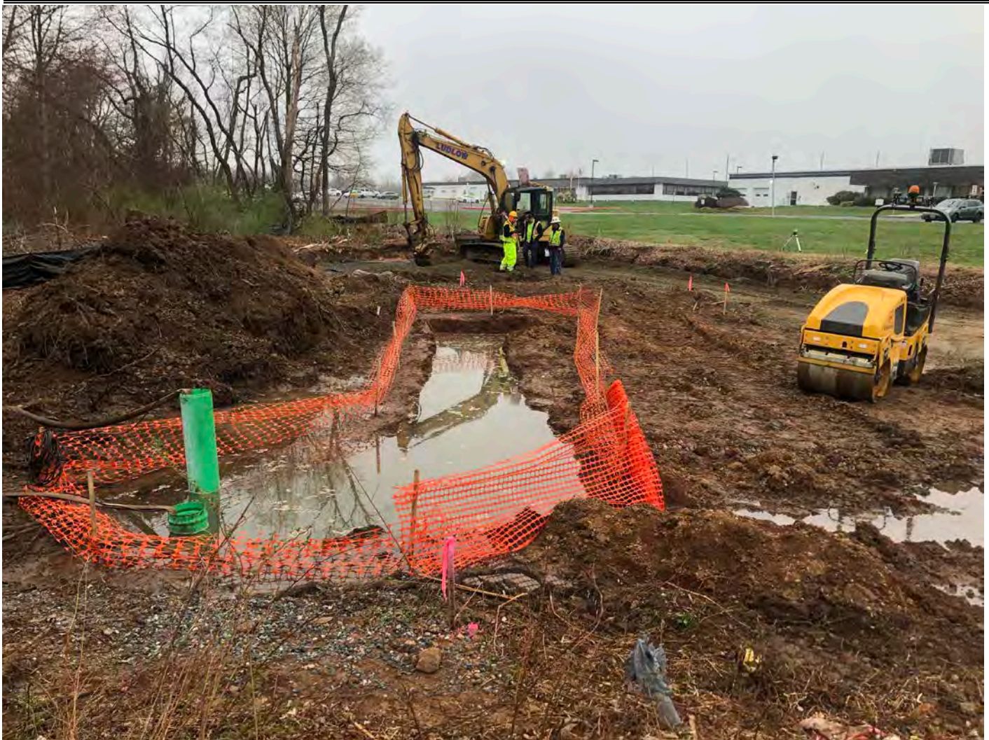
Picture 2: View of the booster station work zone located at Station 750+63 in Middletown. View to the west.
