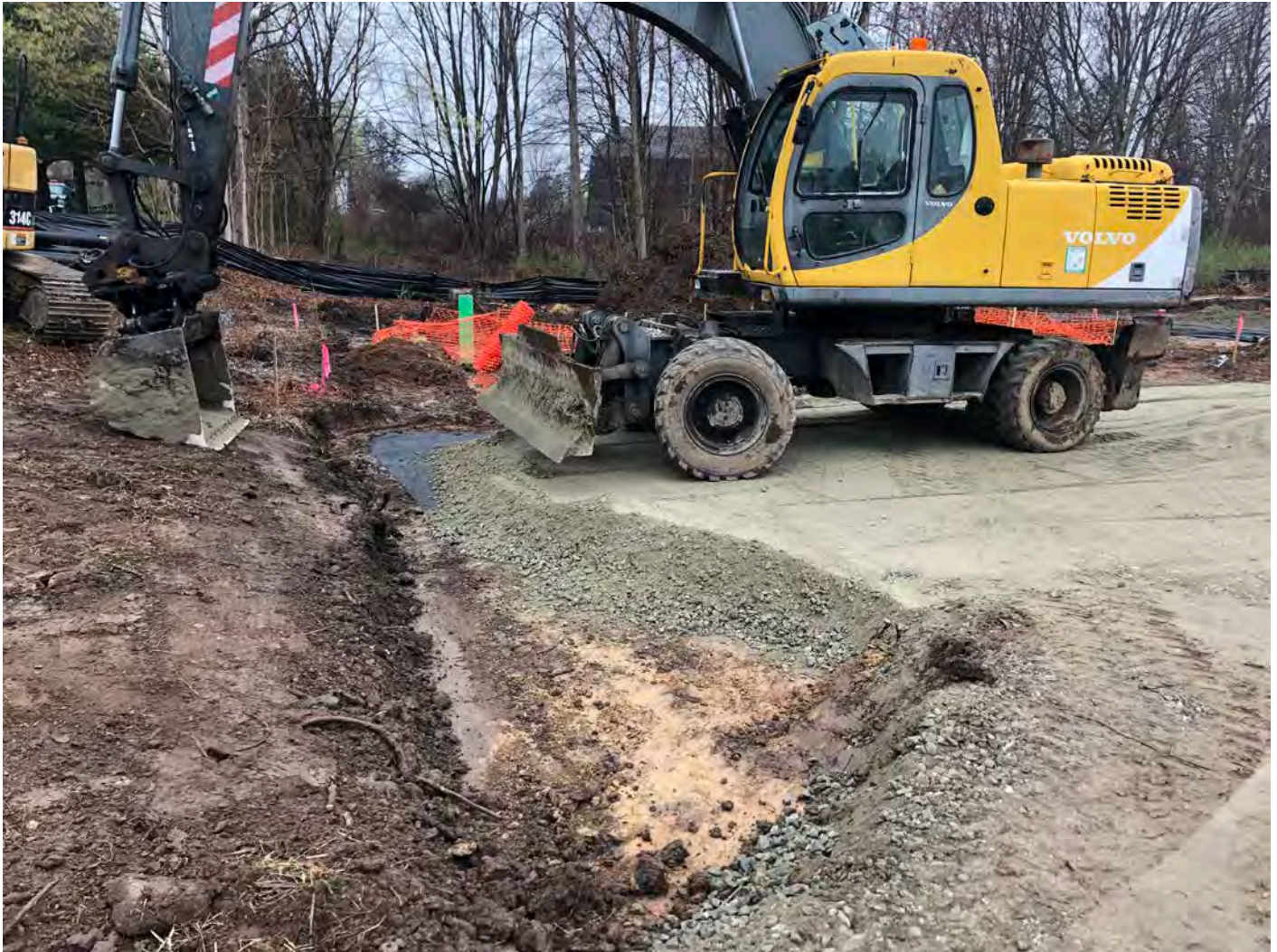
Picture 3: Ludlow placing 1.25” gravel on top of geofabric as they construct the bituminous concrete driveway at the booster station located at Station 750+63 in Middletown. View to the south.
