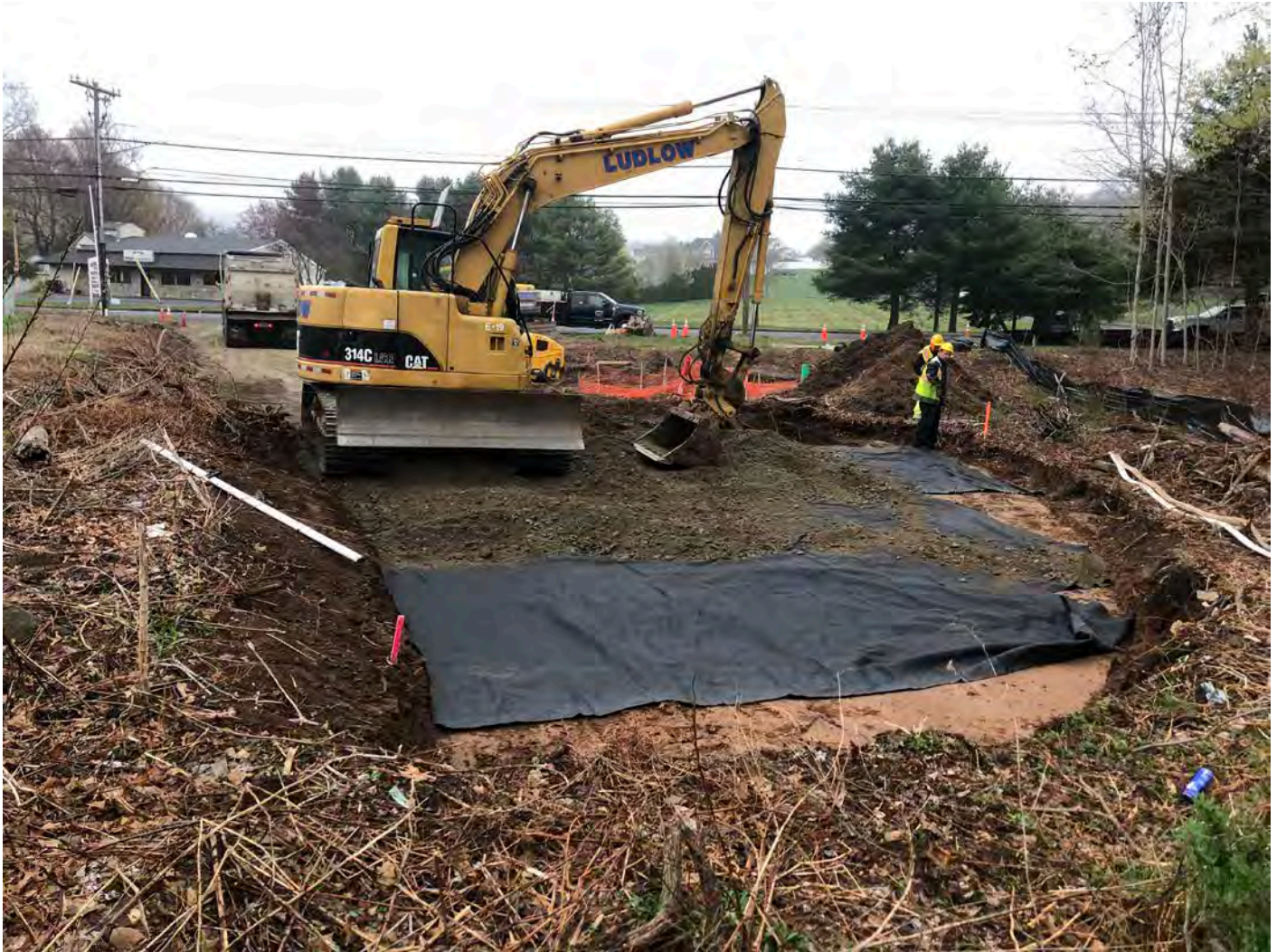
Picture 1: Ludlow placing 1.25" gravel on top of geofabric as they construct the bituminous concrete driveway at the booster station located at Station 750+63 in Middletown. View to the southeast.
