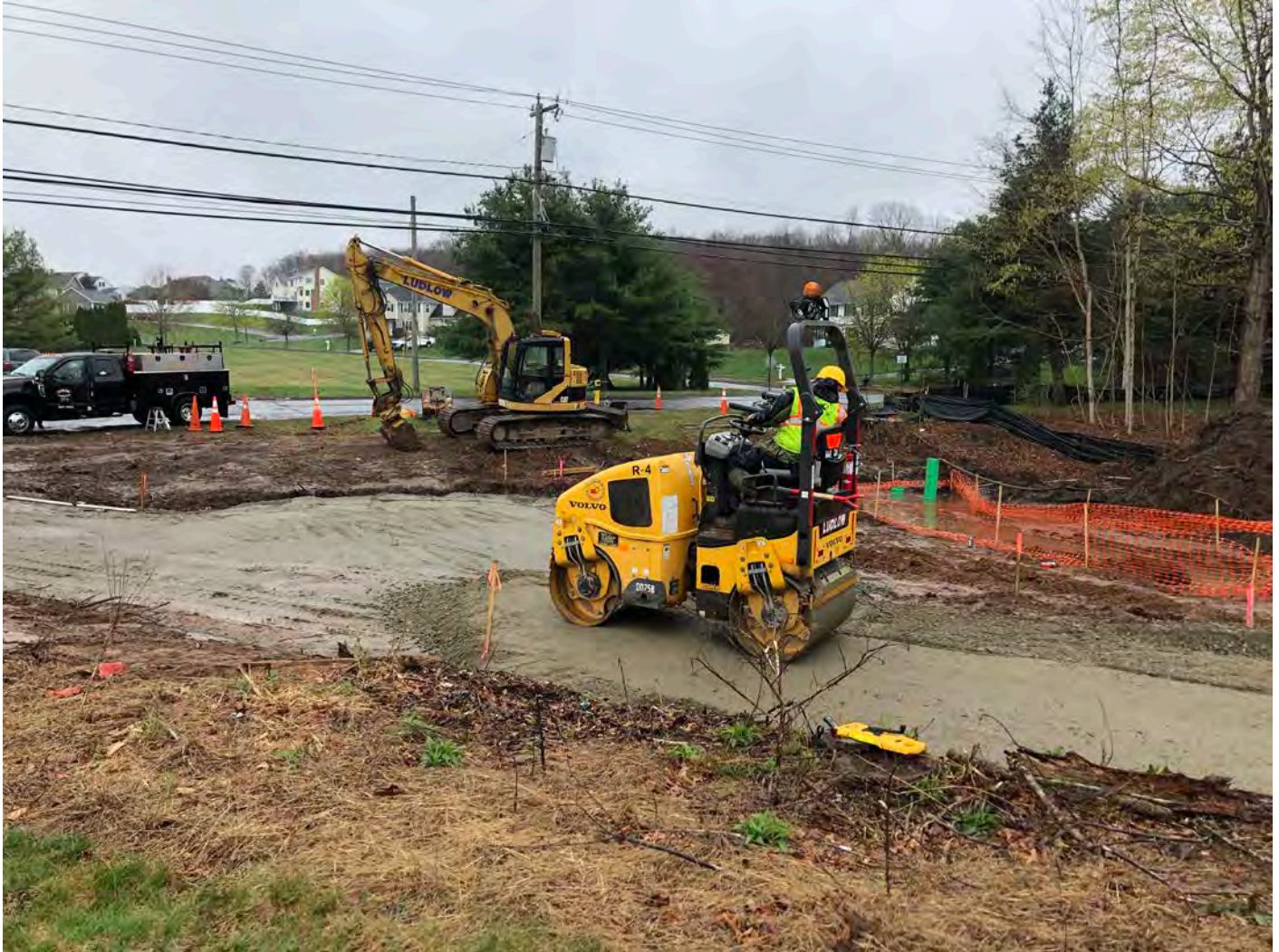
Picture 4: Ludlow compacting 1.25" gravel as they construct the bituminous concrete driveway at the booster station located at Station 750+63 in Middletown. View to the southeast.
