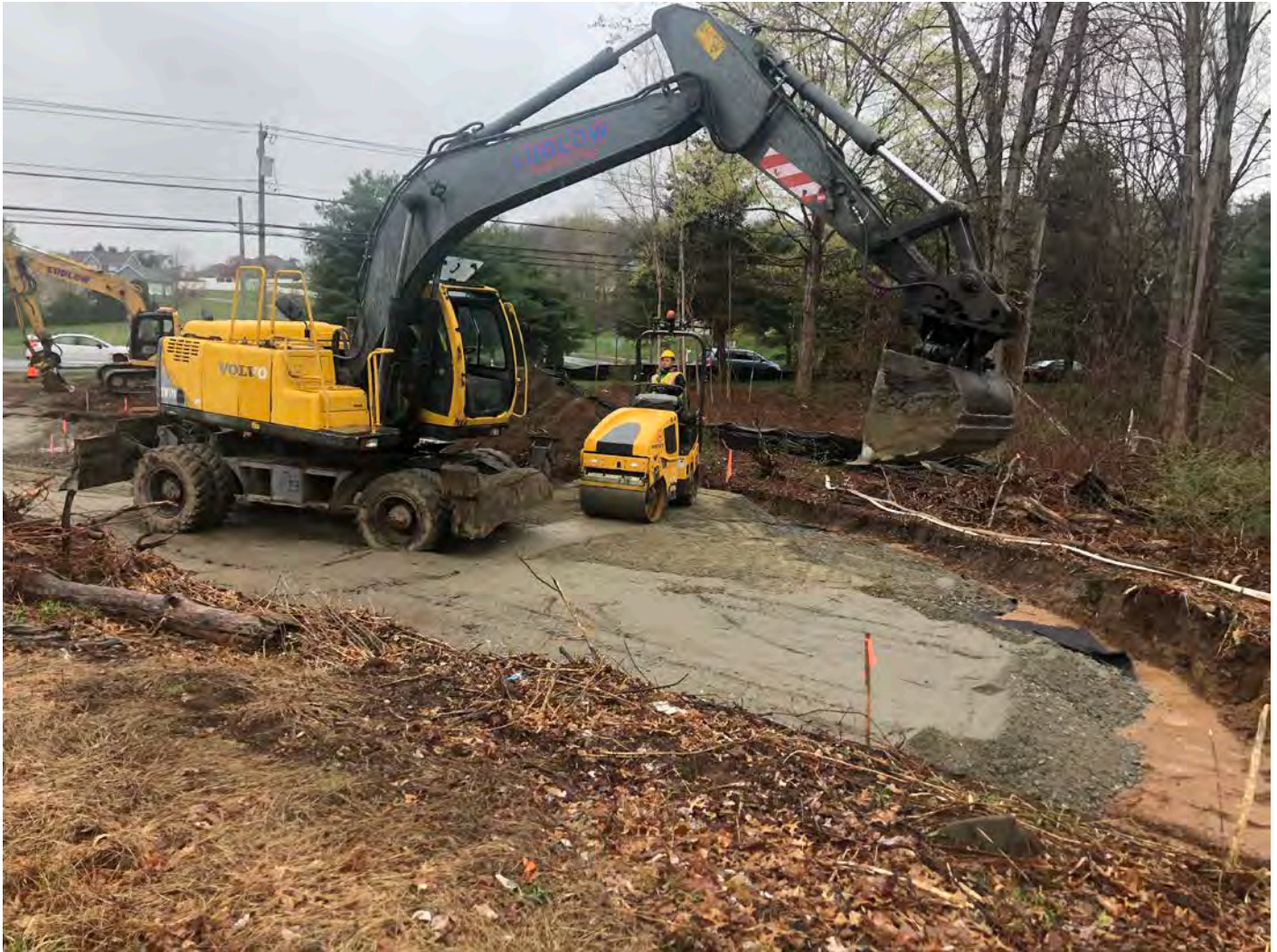
Picture 6: Ludlow grading 1.25" gravel as they construct the bituminous concrete driveway at the booster station located at Station 750+63 in Middletown. View to the southeast.
