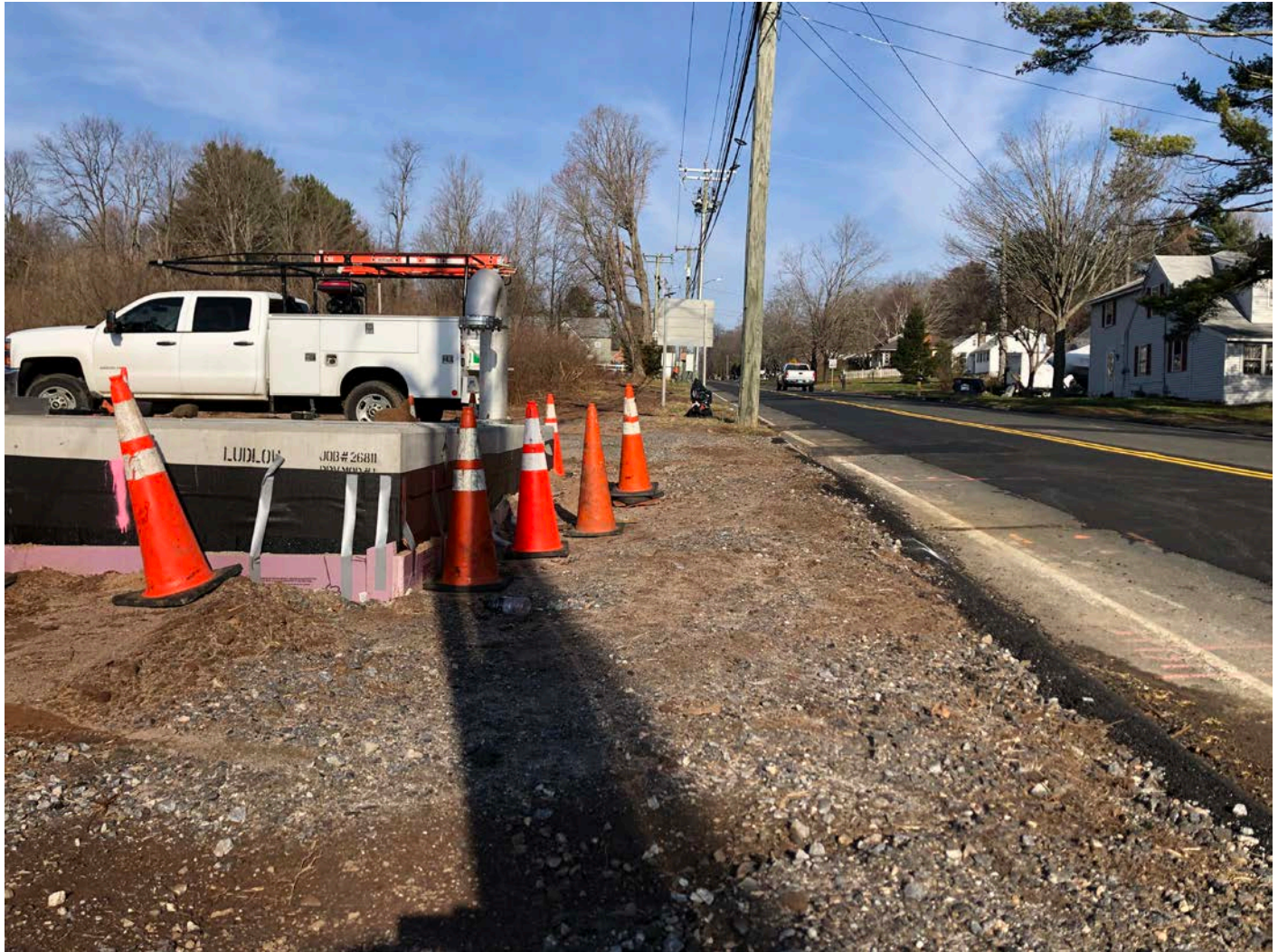
Picture 4: View of the PRV vault located west of Station 161+30 on Main Street, Durham. View to the north.
