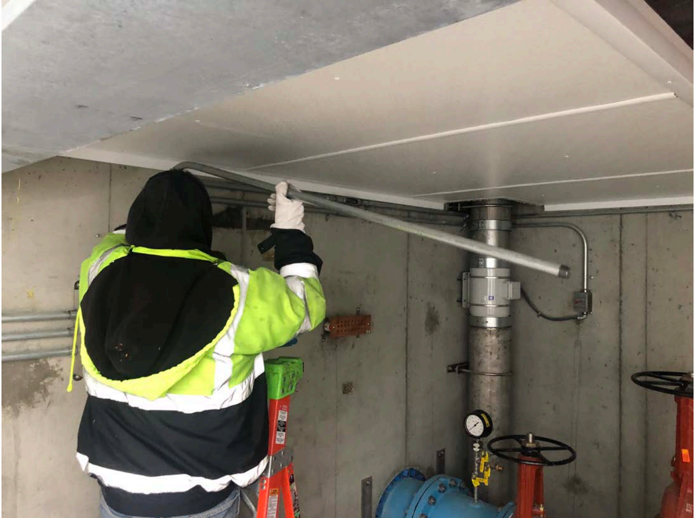
Picture 2: United Concrete installing metal conduit inside of the PRV vault. View to the northeast.
