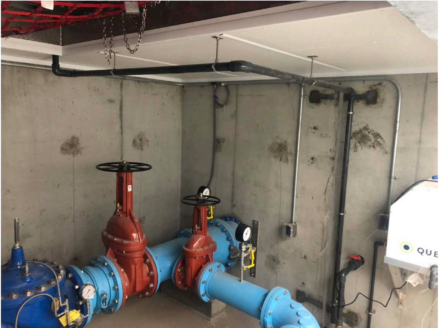
Picture 1: The interior of the PRV vault located at Station 161+30. 2" PVC pipe has been installed, connecting a PVC stub that drains water from the drain channel that surrounds the edge of the eastern vault hatch to the sump located on the southern vault wall. View to the southeast.
