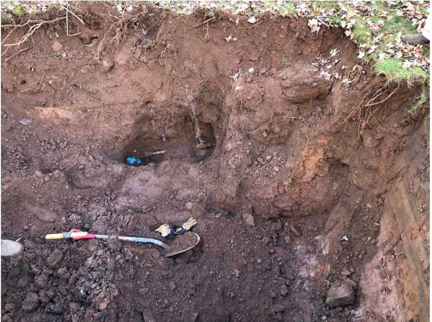
Picture 5: Ludlow uncovered an existing curb stop and service line going into the residence at 120 Main Street, Durham today. Once the existing service line was identified by Ludlow within the residence, Ludlow backfilled the excavation without installing an additional curb stop.
