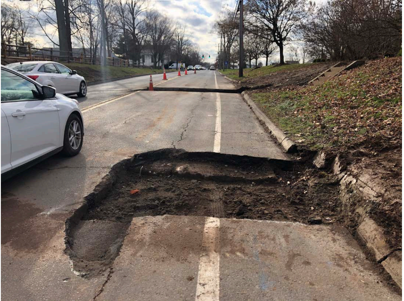
Picture 6: Curb stop overcuts that Ludlow excavated for permanent paving activities today. Curb stop overcut for 120 Main Street in the foreground; curb stop overcut for 119 Main Street, Durham in the background. View to the south.
