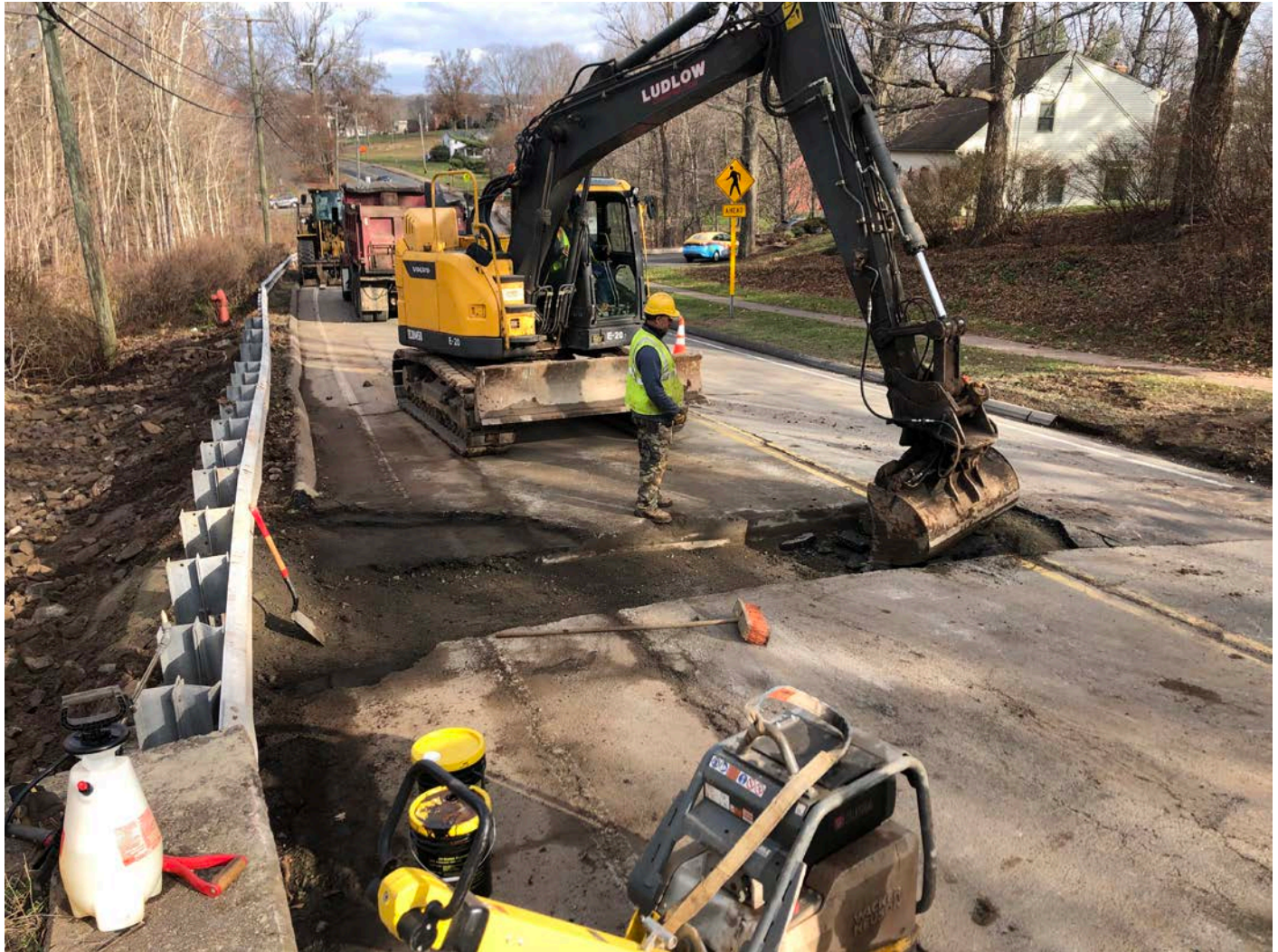
Picture 7: Ludlow excavating curb stop overcut on the southbound lane of Main Street for the curb stop at 127 Main Street, Durham. View to the northeast.
