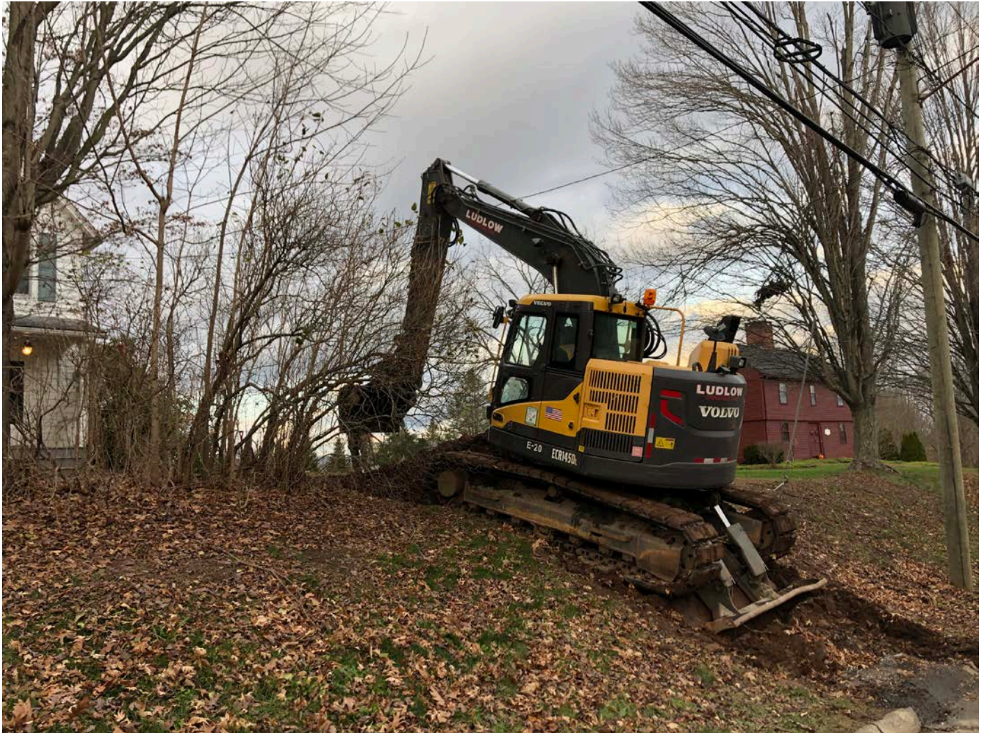
Picture 3: Ludlow excavating for the installation of a 1" curb stop at 120 Main Street, Durham. View to the northwest.
