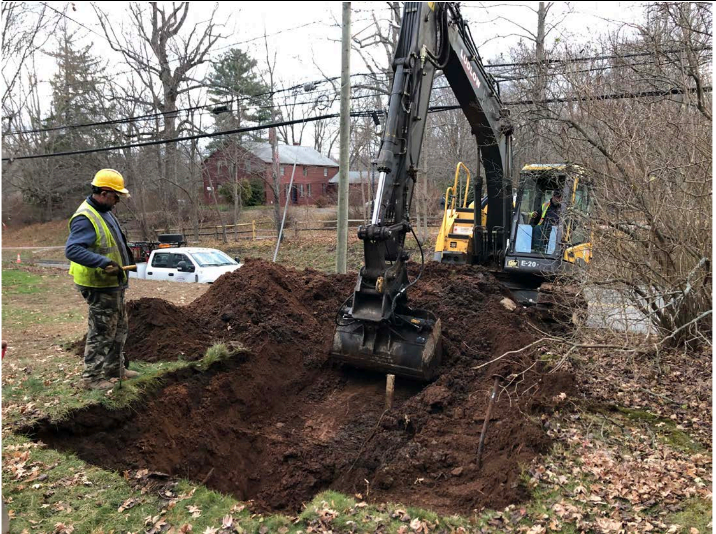
Picture 4: Ludlow excavating for the installation of a 1" curb stop at 120 Main Street, Durham. View to the northeast.
