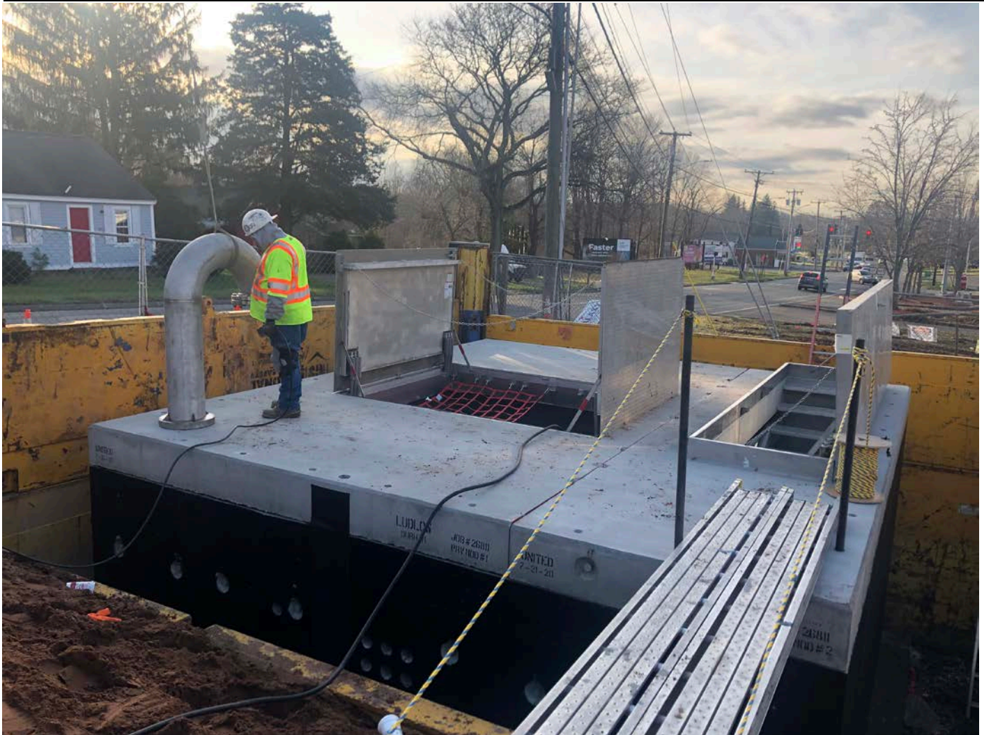
Picture 2: United Concrete installing vent pipe on the northeast corner of the PRV vault roof at Station 161+30 to the west of Main Street, Durham. View to the south.
