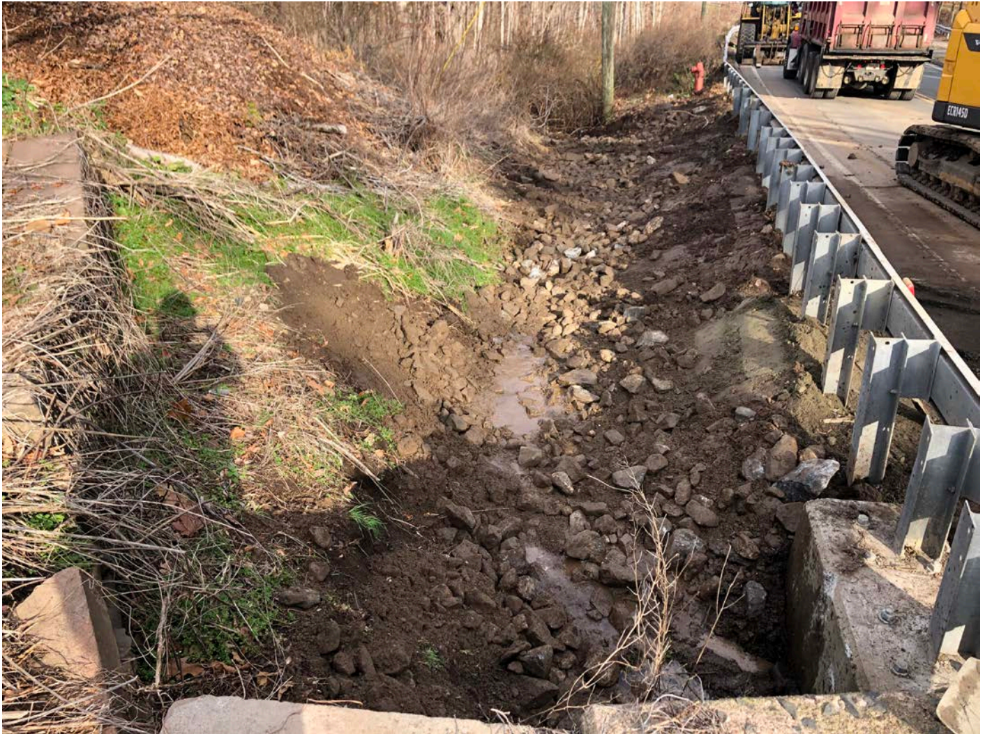
Picture 8: Ludlow placing riprap on top of the cover they placed over the copper service line that was installed yesterday for the curb stop at 127 Main Street, Durham. View to the north.
