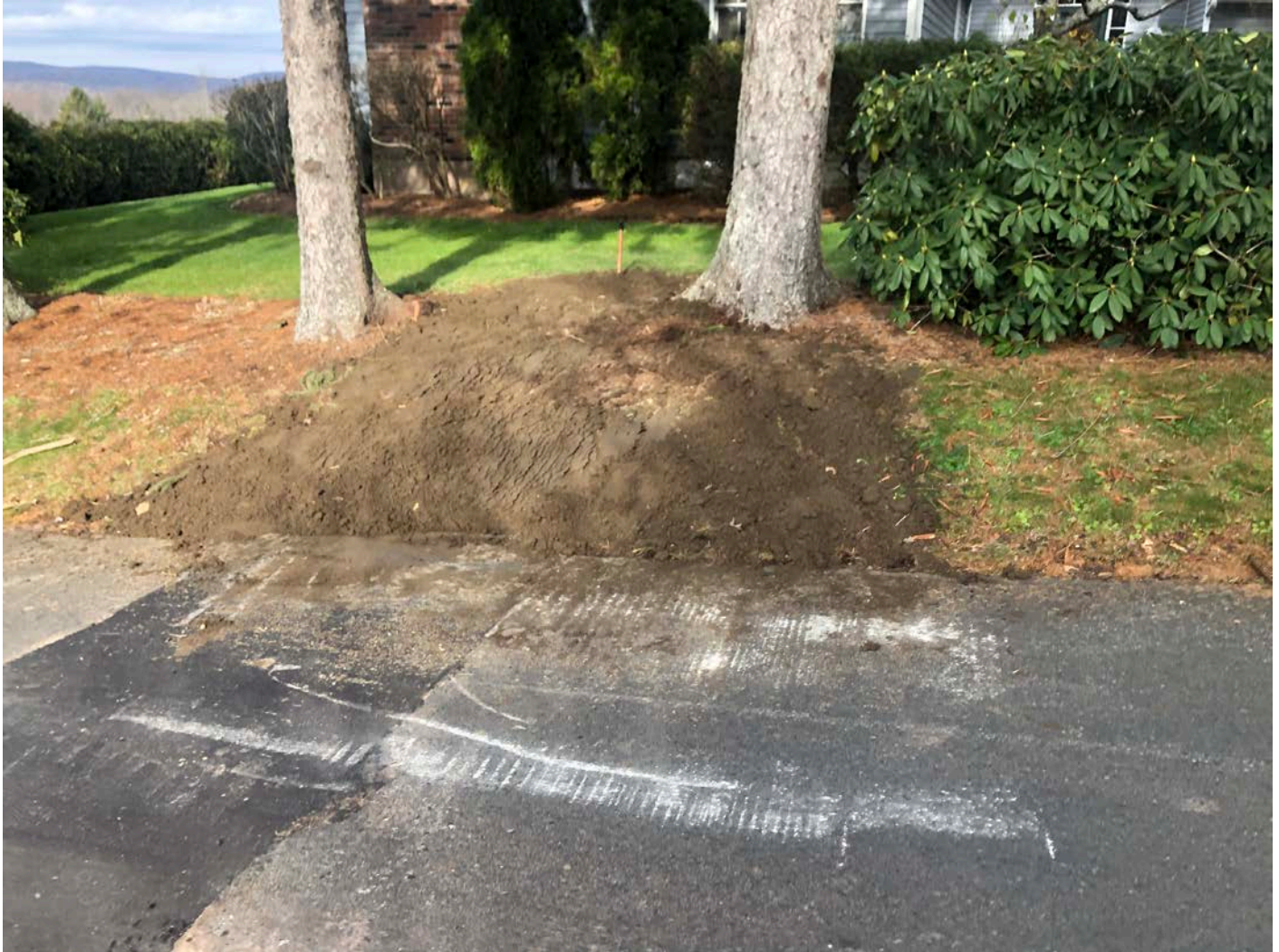
Picture 9: Loam placed over the area of lawn that was disturbed when Ludlow installed a curb stop at 29 Maple Avenue, Durham. View to the north.
