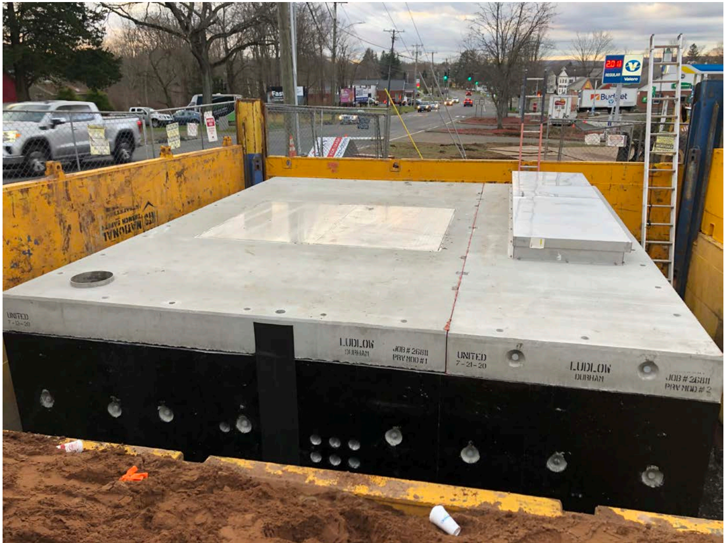
Picture 1: PRV vault with roof sections in place at Station 161+30 to the west of Main Street, Durham. View to the south.
