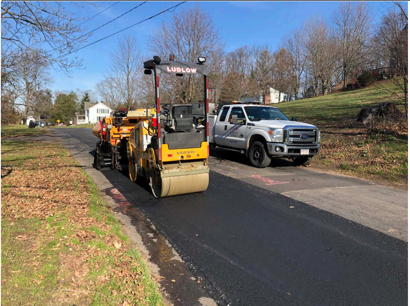
Picture 4: Ludlow compacting shim coat of asphalt that they placed over temporary trench pavement on the southbound lane of Maple Avenue, Durham at Station 912+50. View to the northeast.
