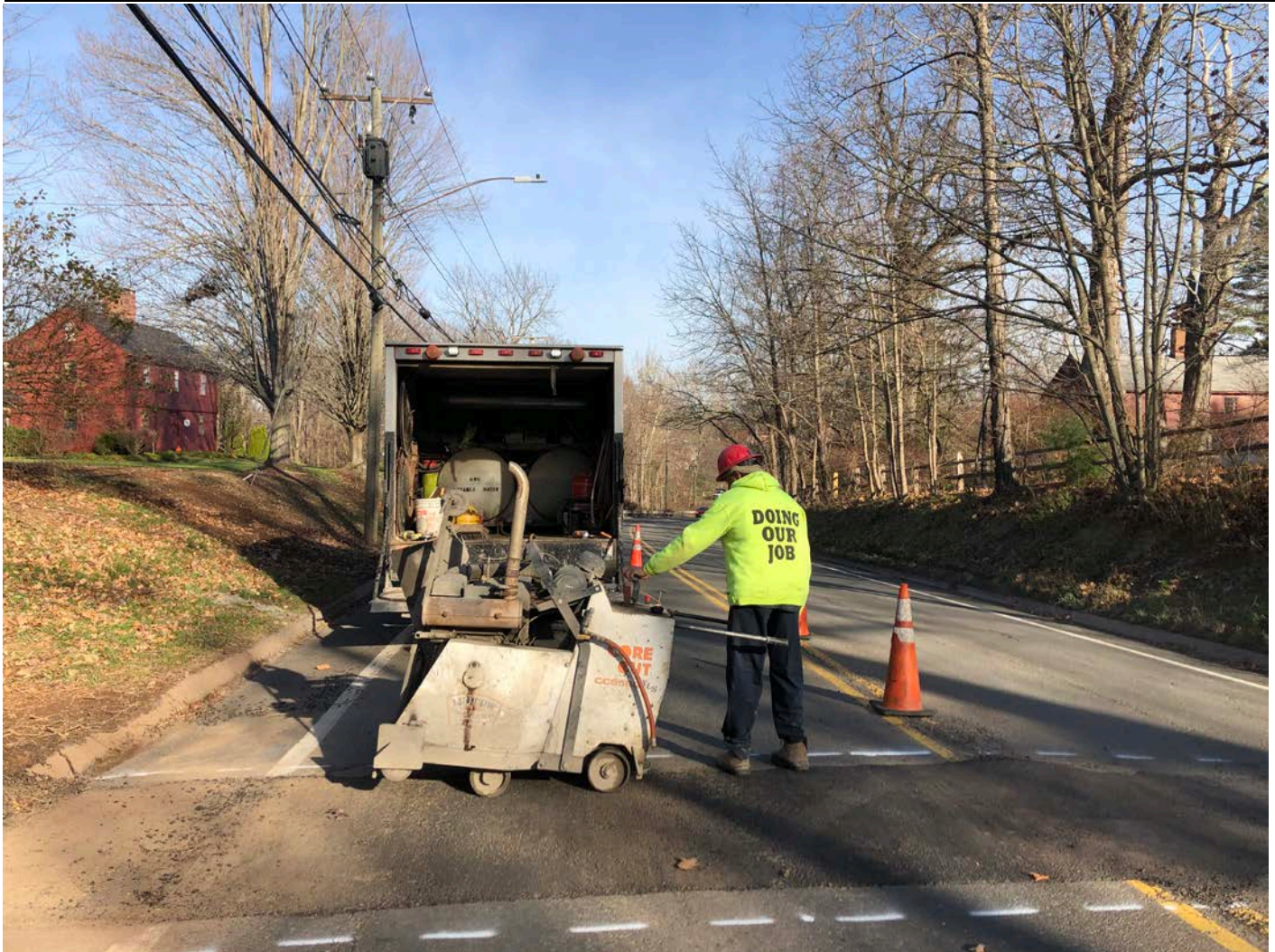
Picture 2: Ludlow saw cutting a curb stop overcut on the southbound lane of Main Street, Durham between 120 and 119 Main Street. View to the north.
