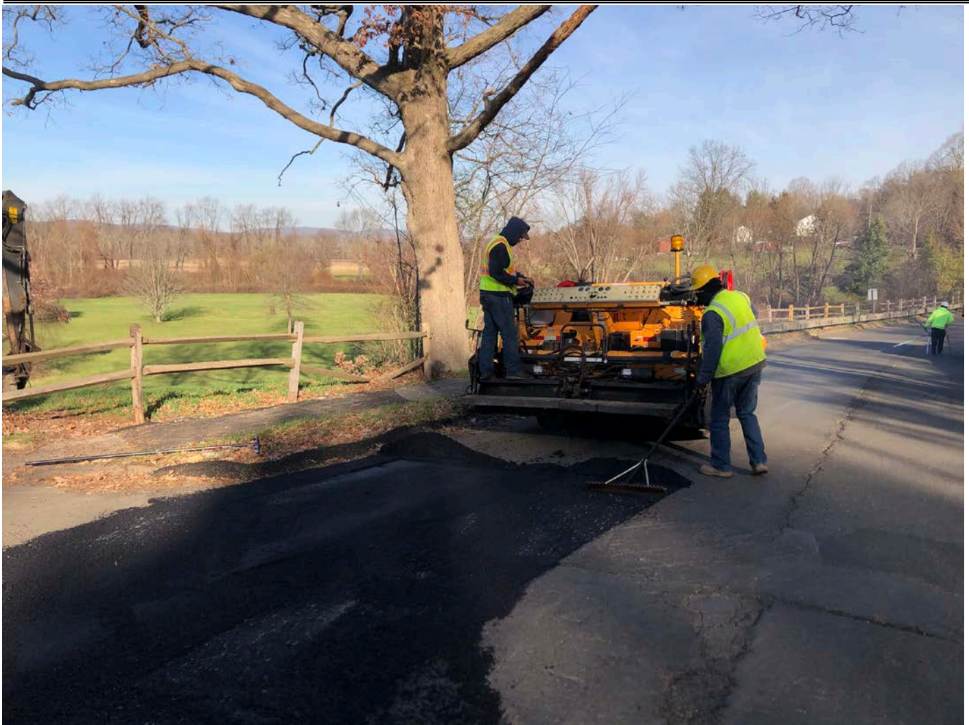
Picture 3: Ludlow shim coating over temporary water line trench pavement on Maple Avenue, Durham at Station 901+50. View to the north.
