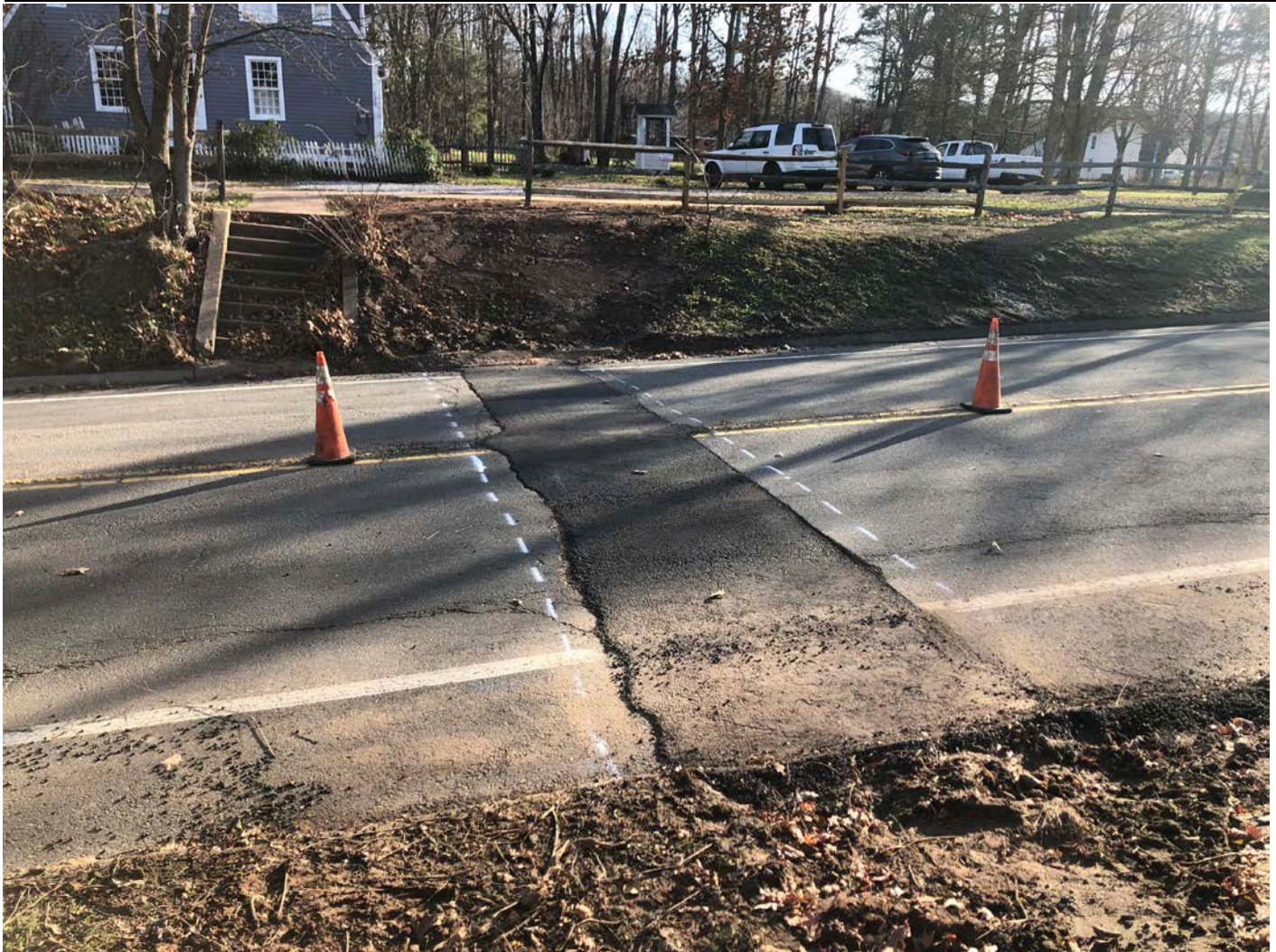
Picture 1: Cut lines marked out on the curb stop overcut for 119 Main Street, Durham that Ludlow cut today. View to the east.
