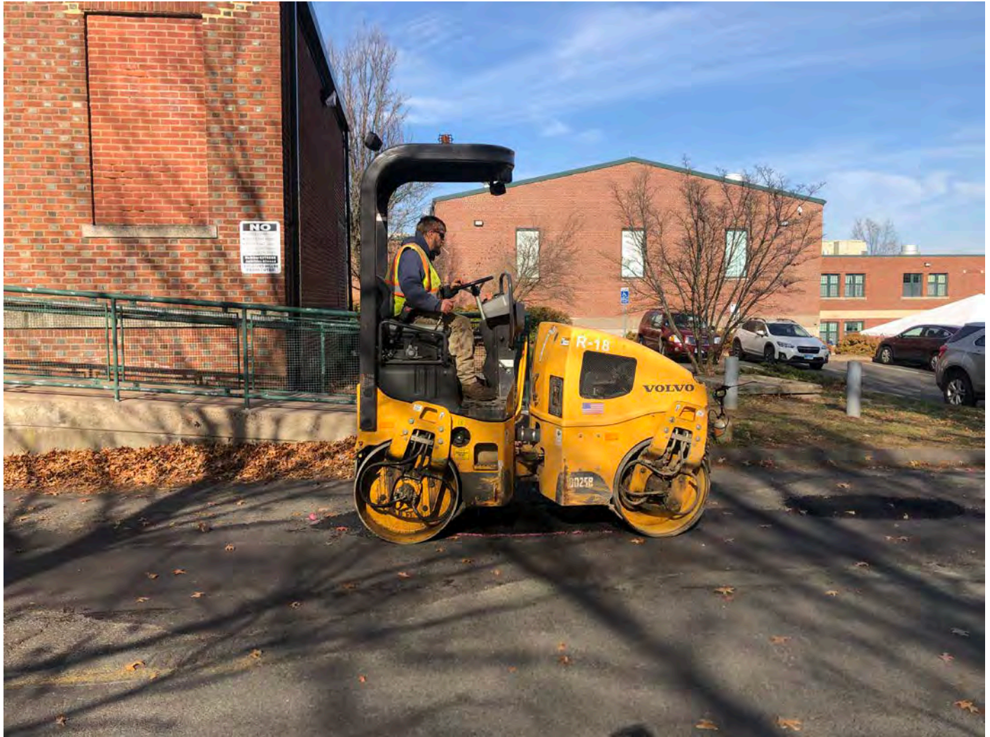
Picture 6: Ludlow compacting asphalt that they have placed to fill depressions on Pickett Lane, Durham at Station 504+00. View to the north.
