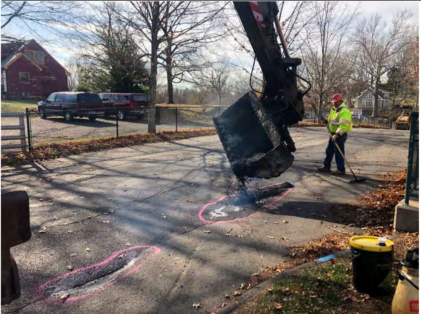
Picture 5: Ludlow patching potholes and depressions on Pickett Lane, Durham at Station 504+00. View to the northeast.
