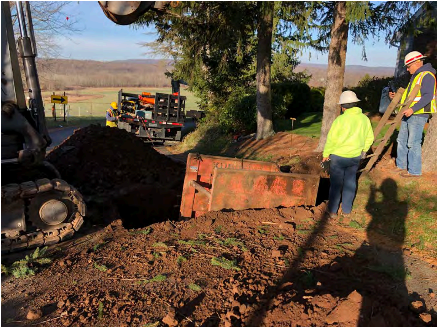
Picture 1: Ludlow excavating at 29 Maple Avenue, Durham for the installation of the installation of a curb stop. View to the west.
