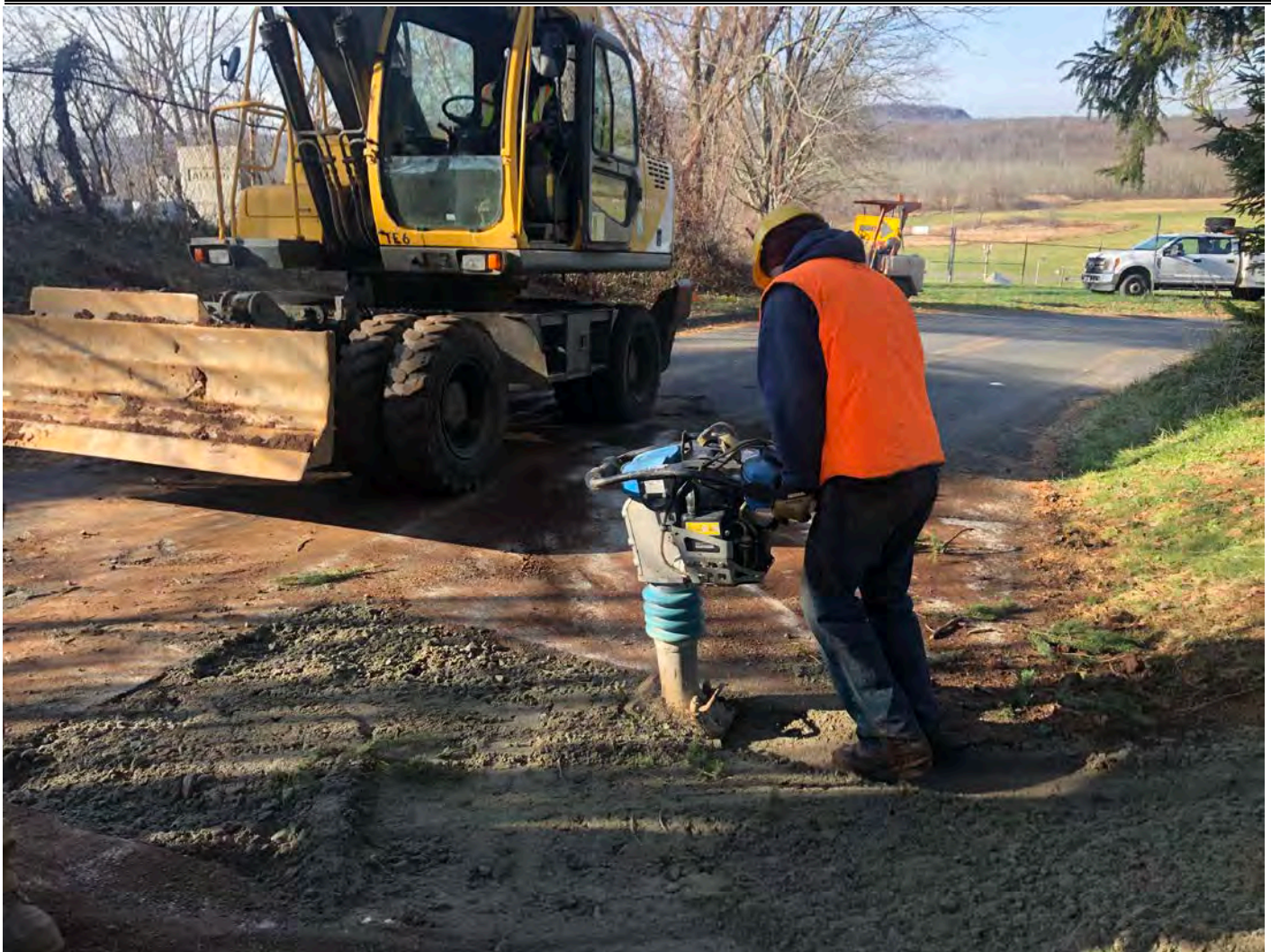
Picture 3: Ludlow compacting backfill in the trench that was excavated for the installation of a corporation stop and a curb stop for 29 Maple Avenue, Durham. View to the west.
