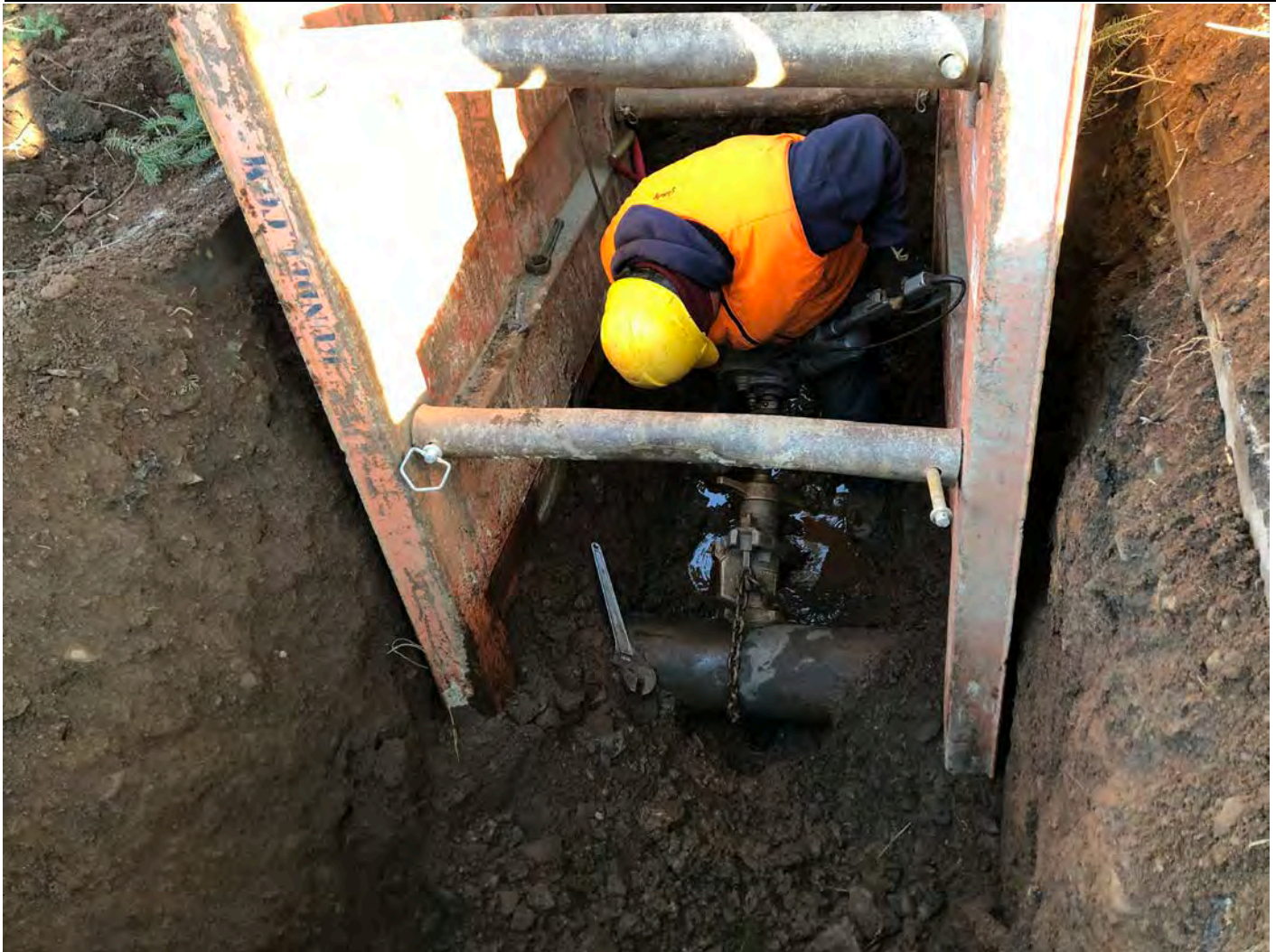
Picture 2: Ludlow tapping the existing Town water line for the installation of a corporation stop and a curb stop for 29 Maple Avenue, Durham. View to the west.
