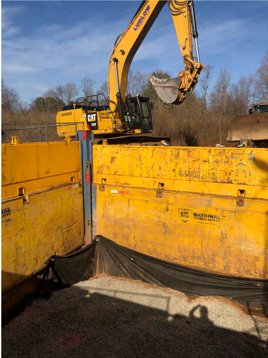
Picture 4: View of the PRV vault located to the west of Main Street, Durham at Station 161+30. Ludlow has placed and fine-graded 3/4" gravel at the bottom of the excavation today. View to the northwest.
