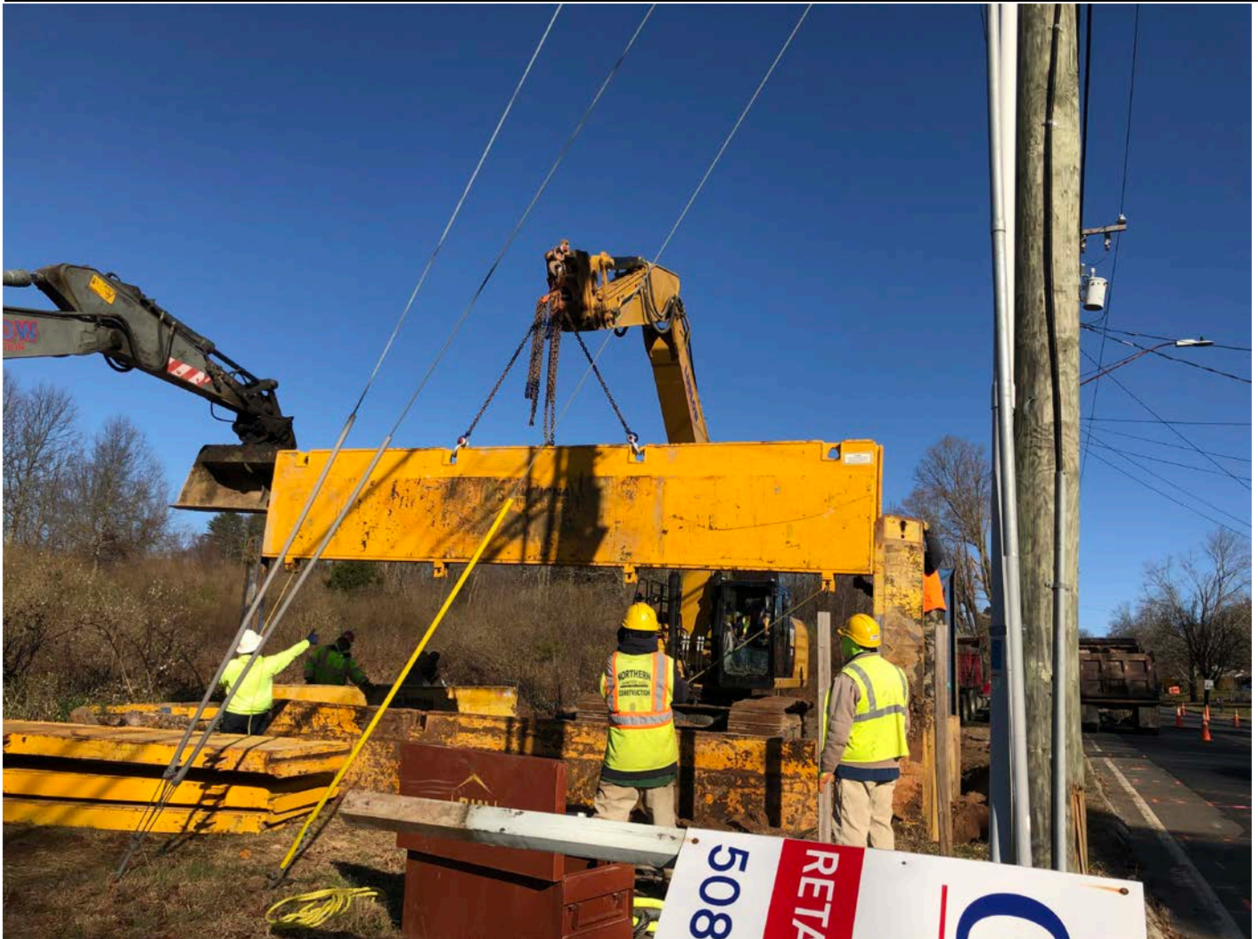
Picture 2: Ludlow placing the second sheeting panel on the south side of the Pressure Reducing Valve Vault on Main Street.
