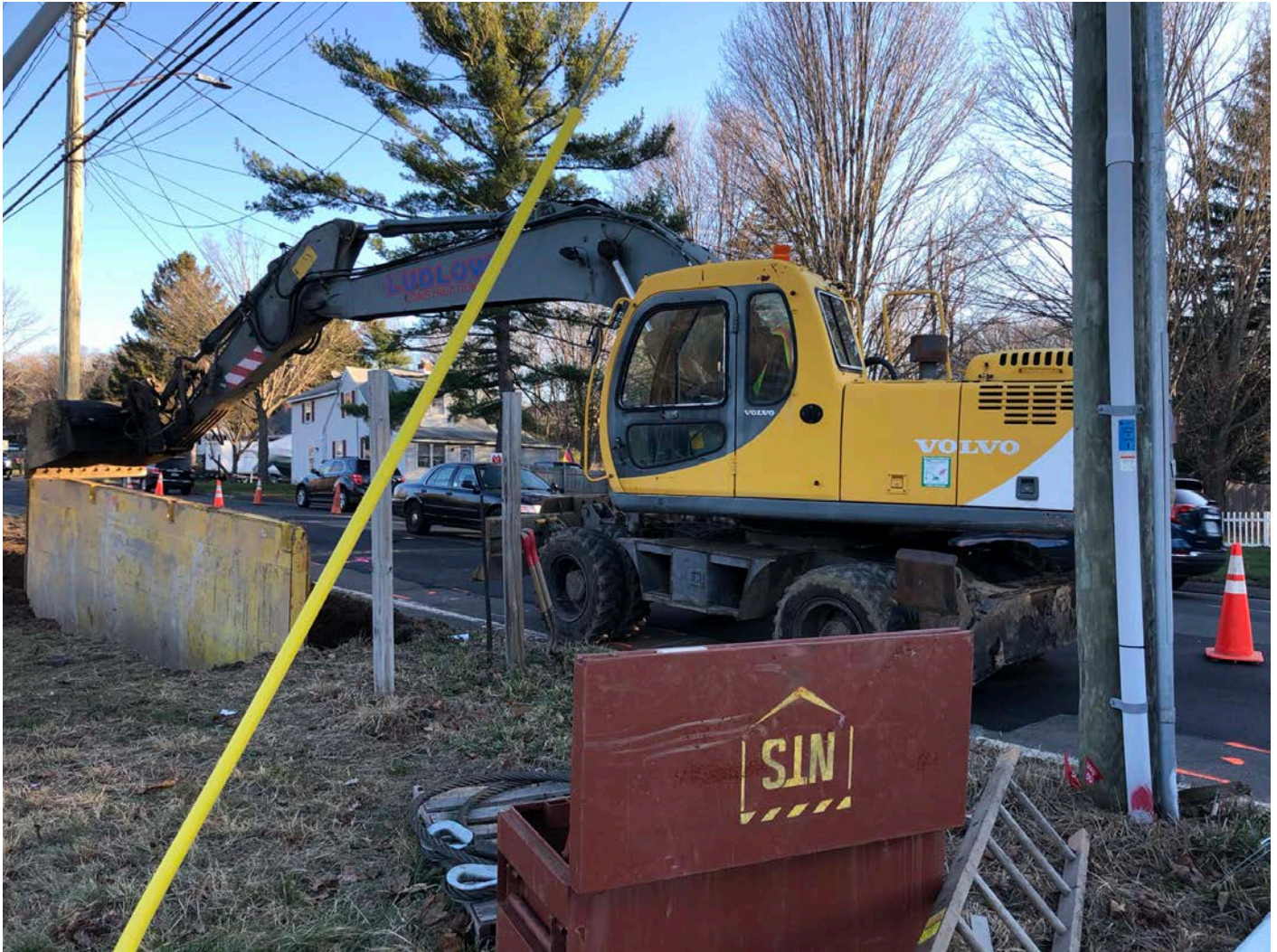
Picture 1: Ludlow excavating the west side of the Pressure Reducing Valve Vault site just north of 384 Main Street.
