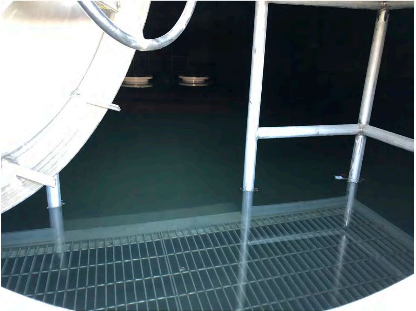
Picture 1: Water level in the water tank located to the east of the Shared Access Driveway, Middletown at 0746 hours this morning, prior to Ludlow adding additional water.
