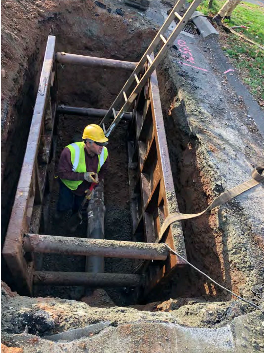
Picture 5: Ludlow in the process of installing a gate valve on the southbound lane of Maple Avenue, Durham at Station 925+55. View to the south.
