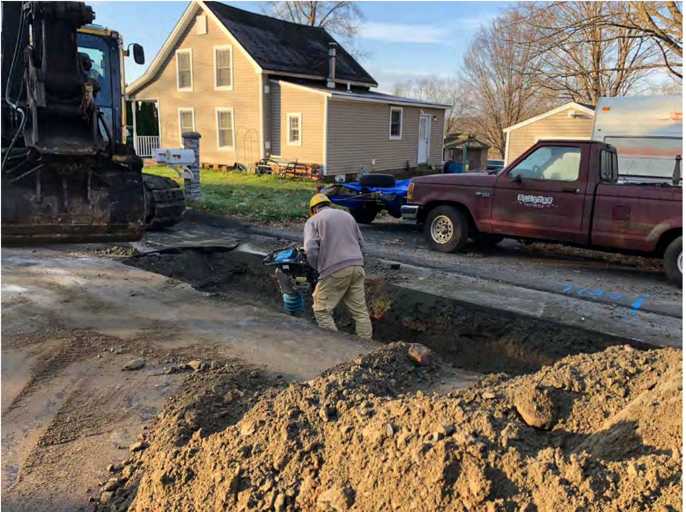
Picture 2: Ludlow compacting soil in test pit they excavated at Station 924+70 as the searched for the source of a leak on the 8" DIP water line on Maple Avenue, Durham. View to the southwest.
