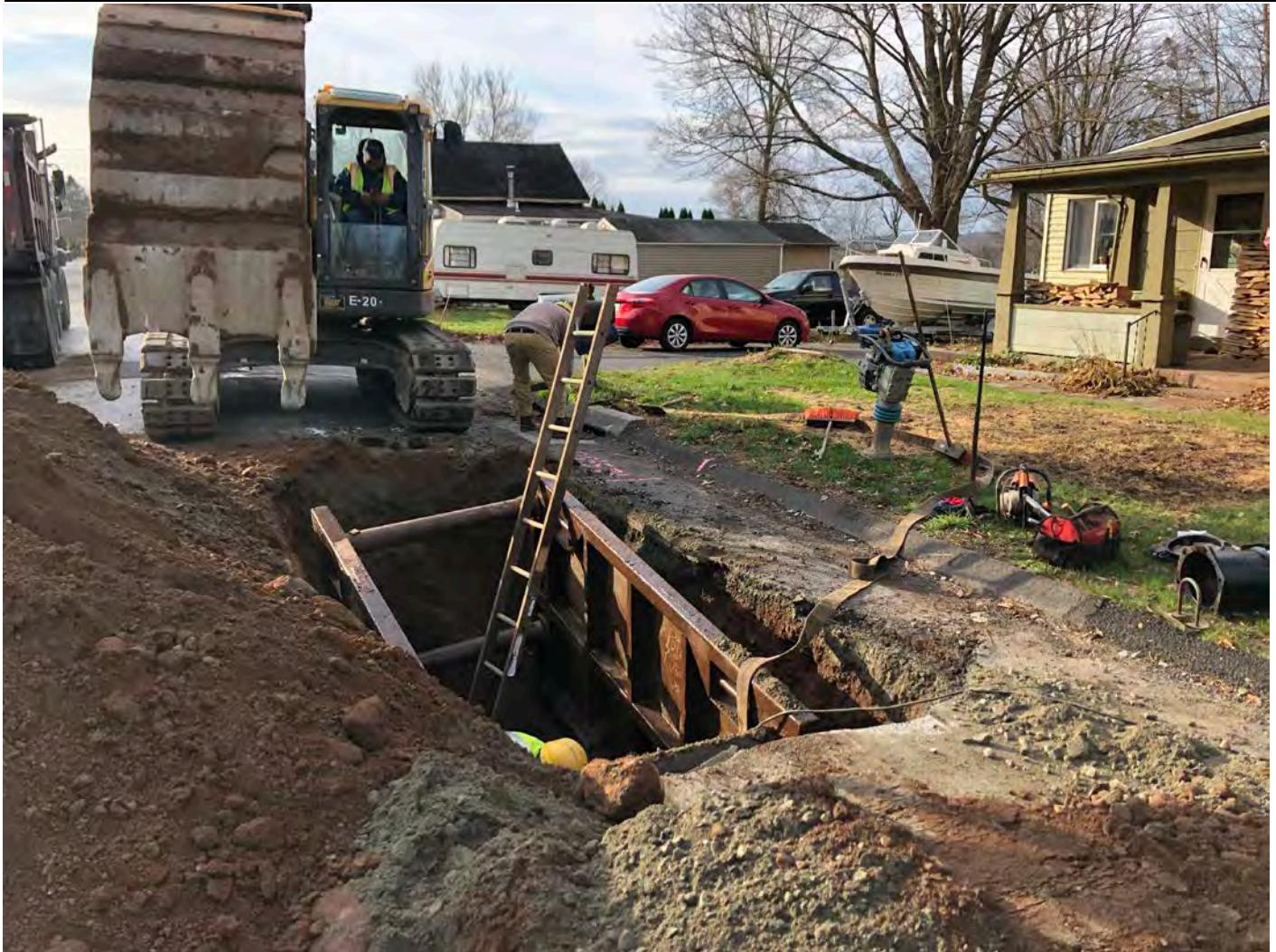
Picture 4: Ludlow in the process of installing a gate valve on the southbound lane of Maple Avenue, Durham at Station 925+55. View to the southwest.
