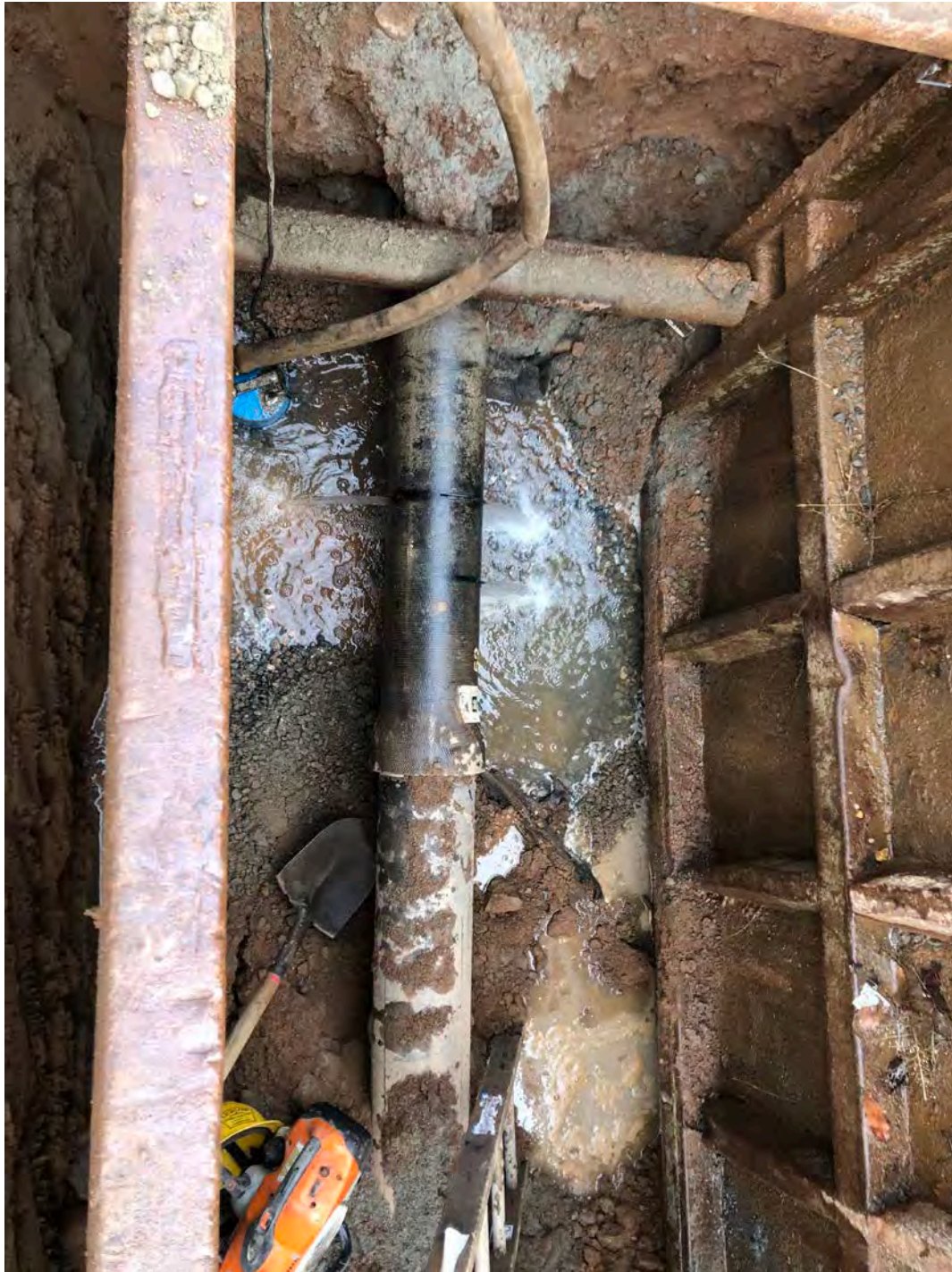
Picture 6: Water exiting the 8”DIP water line on the southbound lane of Maple Avenue, Durham at Station 925+55 where Ludlow cut slits in the pipe.
