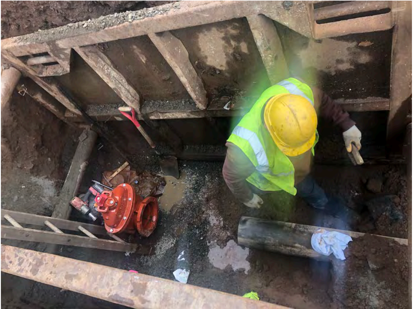
Picture 7: Ludlow in the process of installing a gate valve on the southbound lane of Maple Avenue, Durham at Station 925+55. View to the east.
