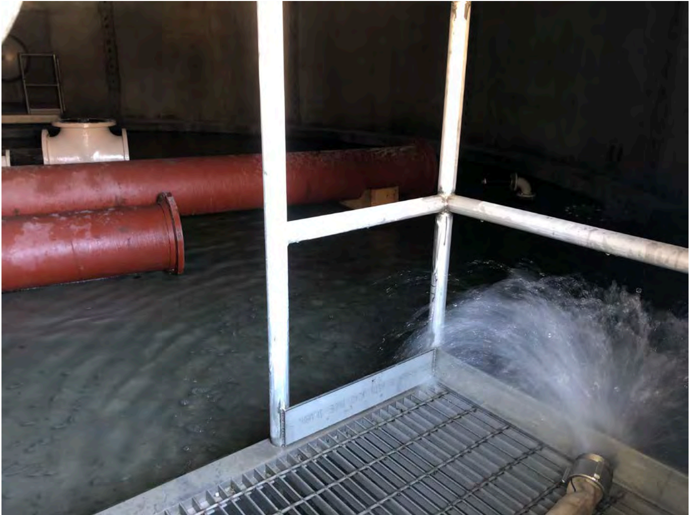
Picture 2: Water being placed into the water tank located to the east of the Shared Access Driveway, Middletown. The water level was brought up to just below the bottom of the manway hatch. View to the southeast.
