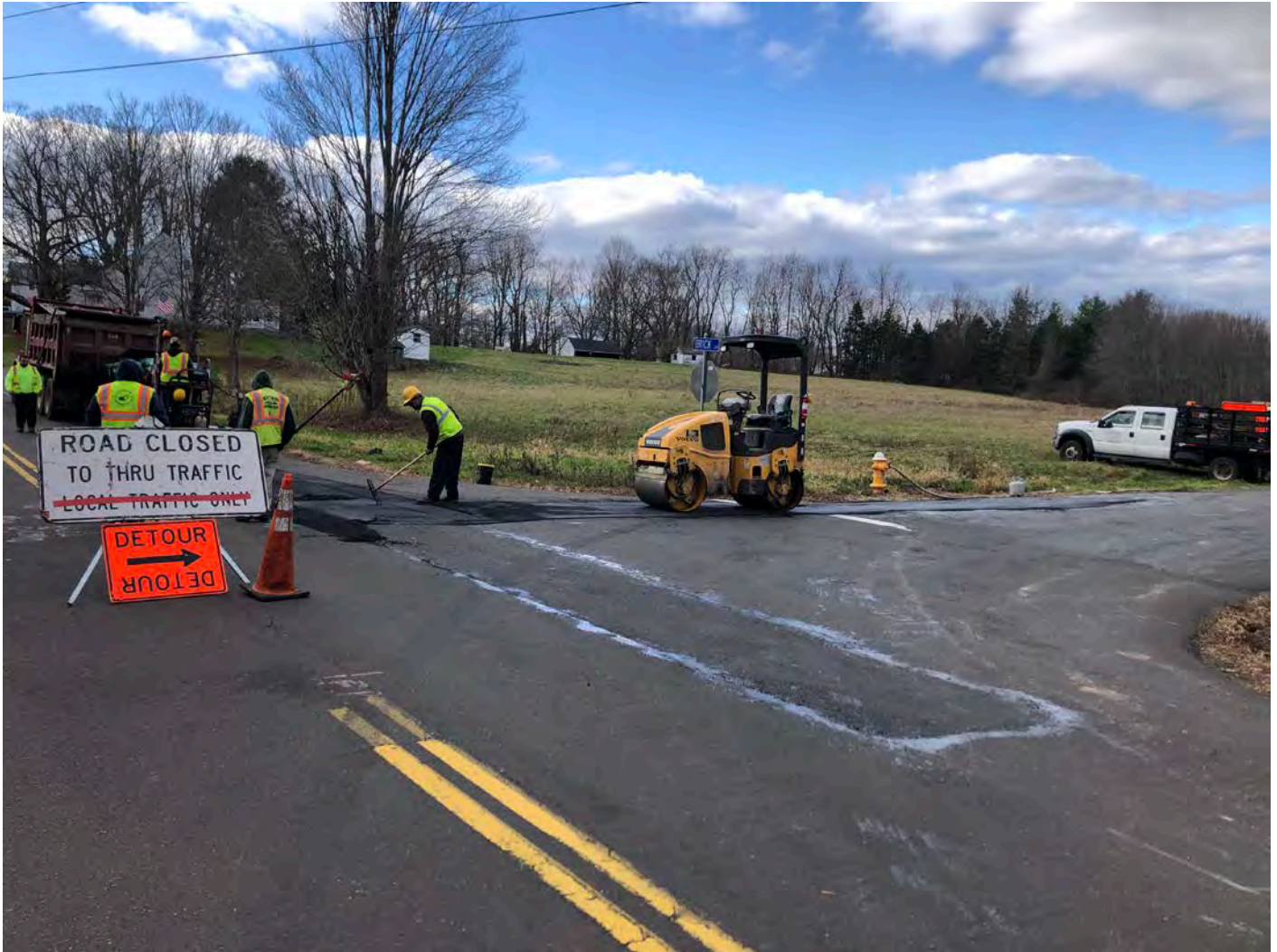
Picture 5: Ludlow shim coating over temporary trench pavement at the intersection of Brick Lane and Maiden Lane, Durham. View to the northwest.
