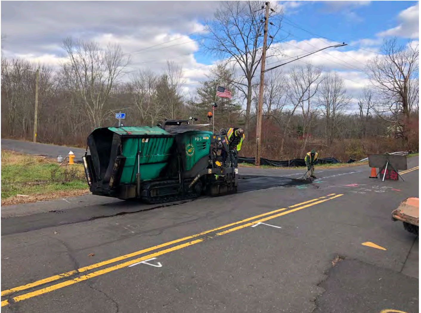
Picture 4: Ludlow shim coating over temporary trench pavement at the intersection of Brick Lane and Maiden Lane, Durham. View to the northeast.
