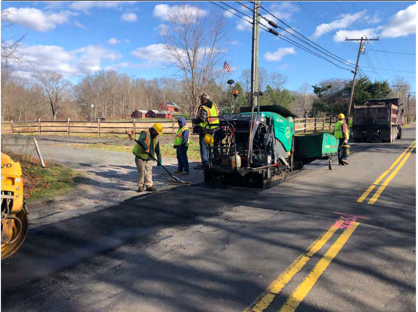
Picture 3: Ludlow shim coating over temporary trench pavement on Maiden Lane, Durham. View to the northeast.
