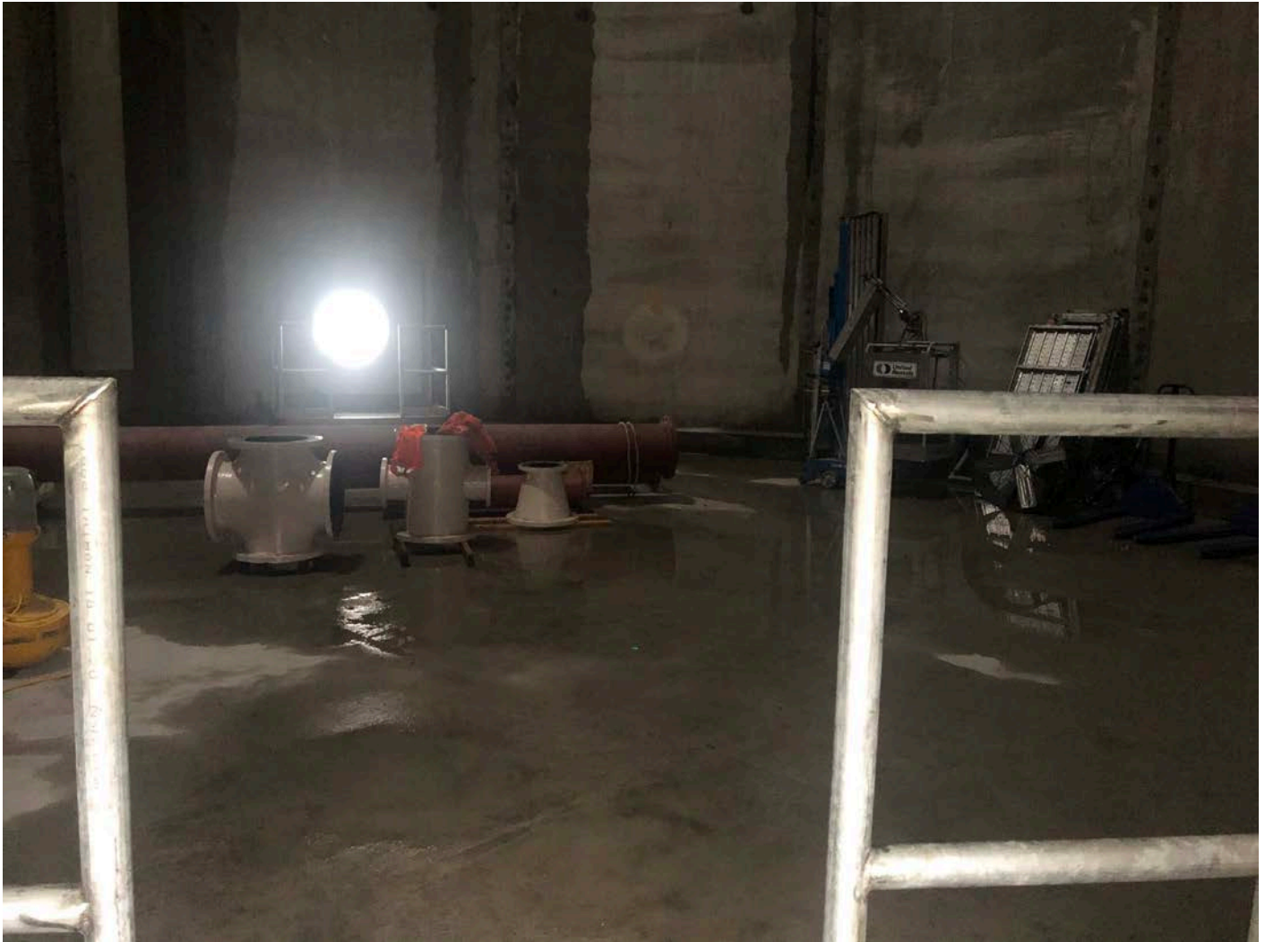
Picture 2: Current view of water tank interior. Water tank work zone located to the east of the Shared Access Driveway, Middletown
