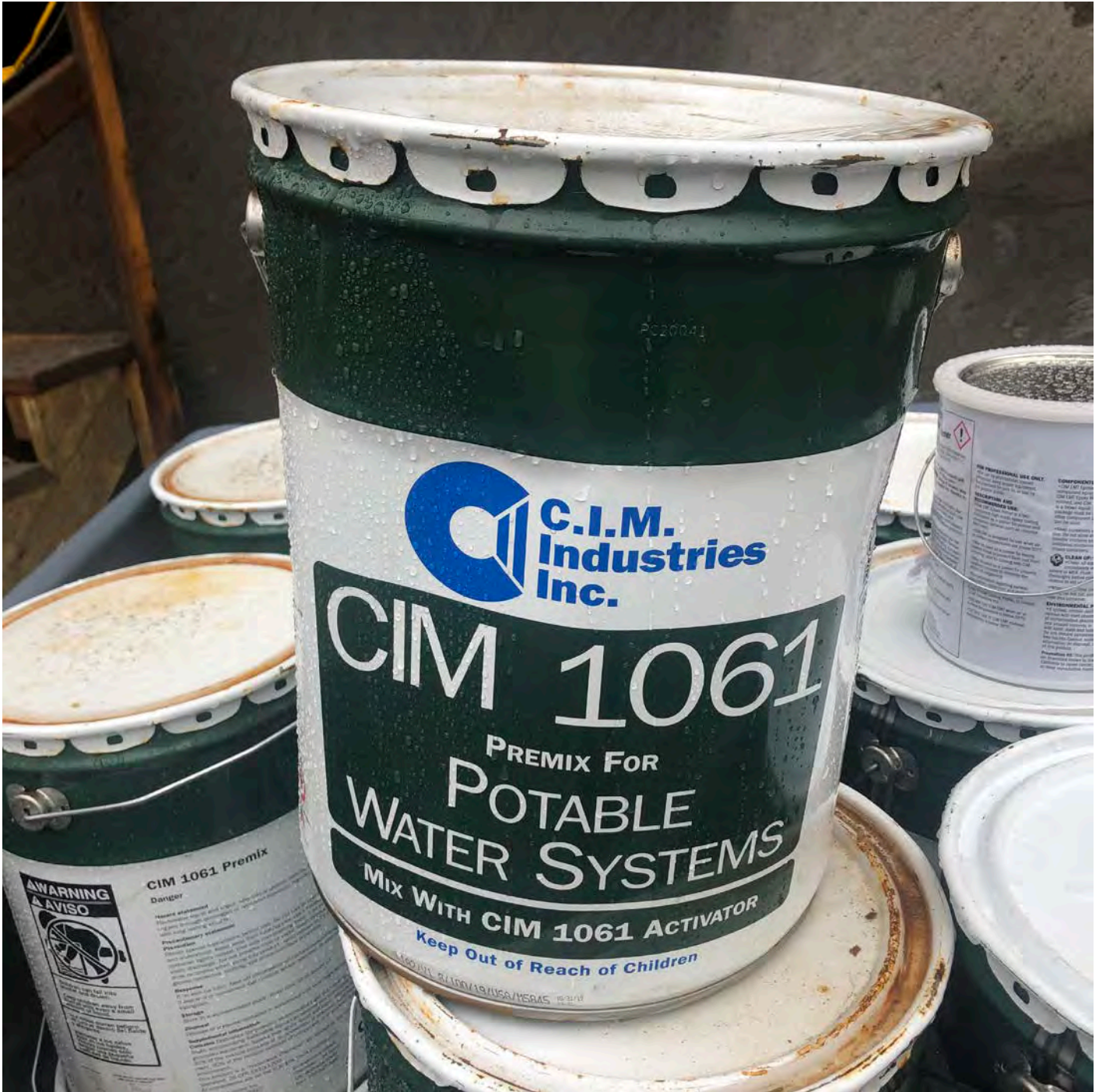
Picture 3: Part one of the two-part coating that will be applied to the interior of the water tank. Water tank work zone located to the east of the Shared Access Driveway, Middletown.
