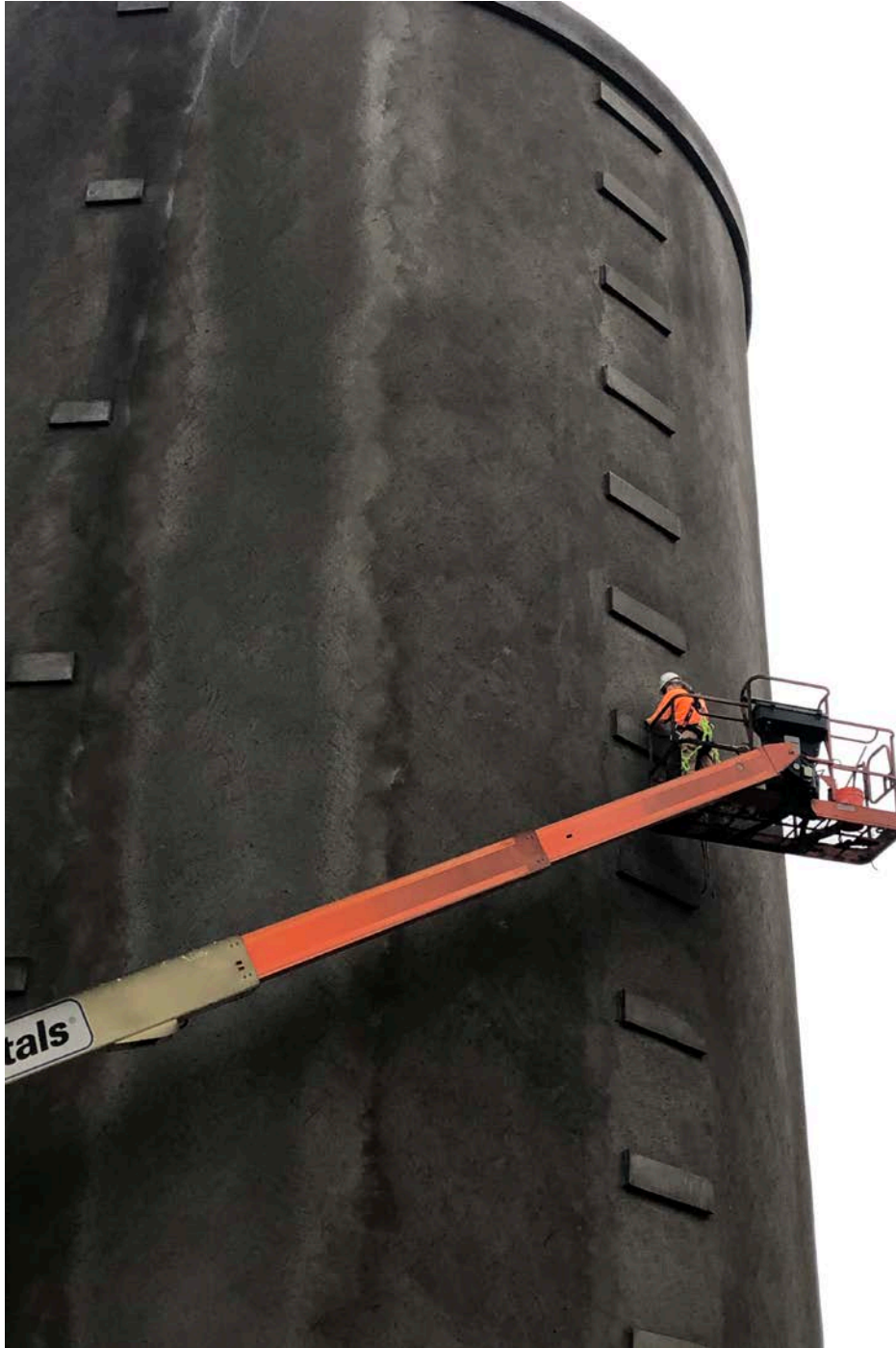
Picture 1: DN Tanks cleaning up shotcrete on the ladder supports on the water tank exterior. Water tank work zone, east of the Shared Access Driveway, Middletown. View to the northeast.
