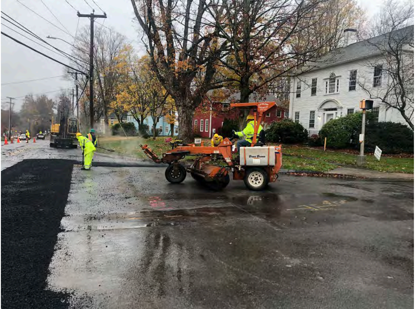
Picture 6: Ludlow cleaning up work zone between Stations 195+30 to 195+85 as part of permanent paving activities on the southbound lane of Main Street, Durham. View to the south.
