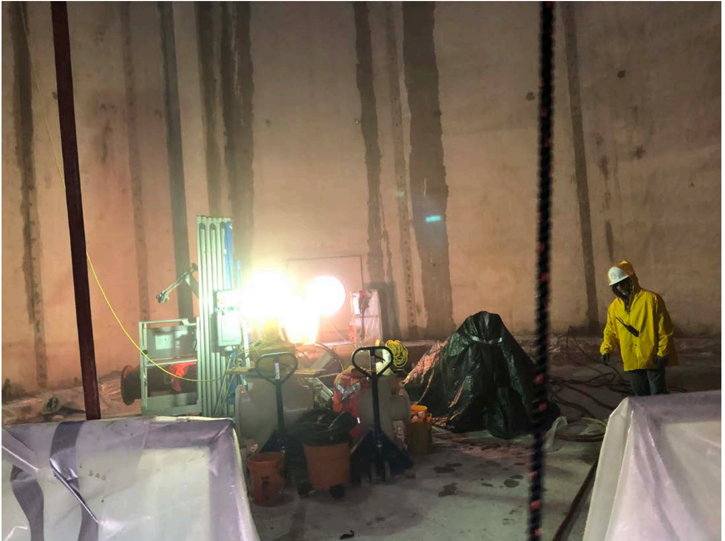
Picture 7: Current view of water tank interior. Water tank work zone located to the east of the Shared Access Driveway, Middletown.
