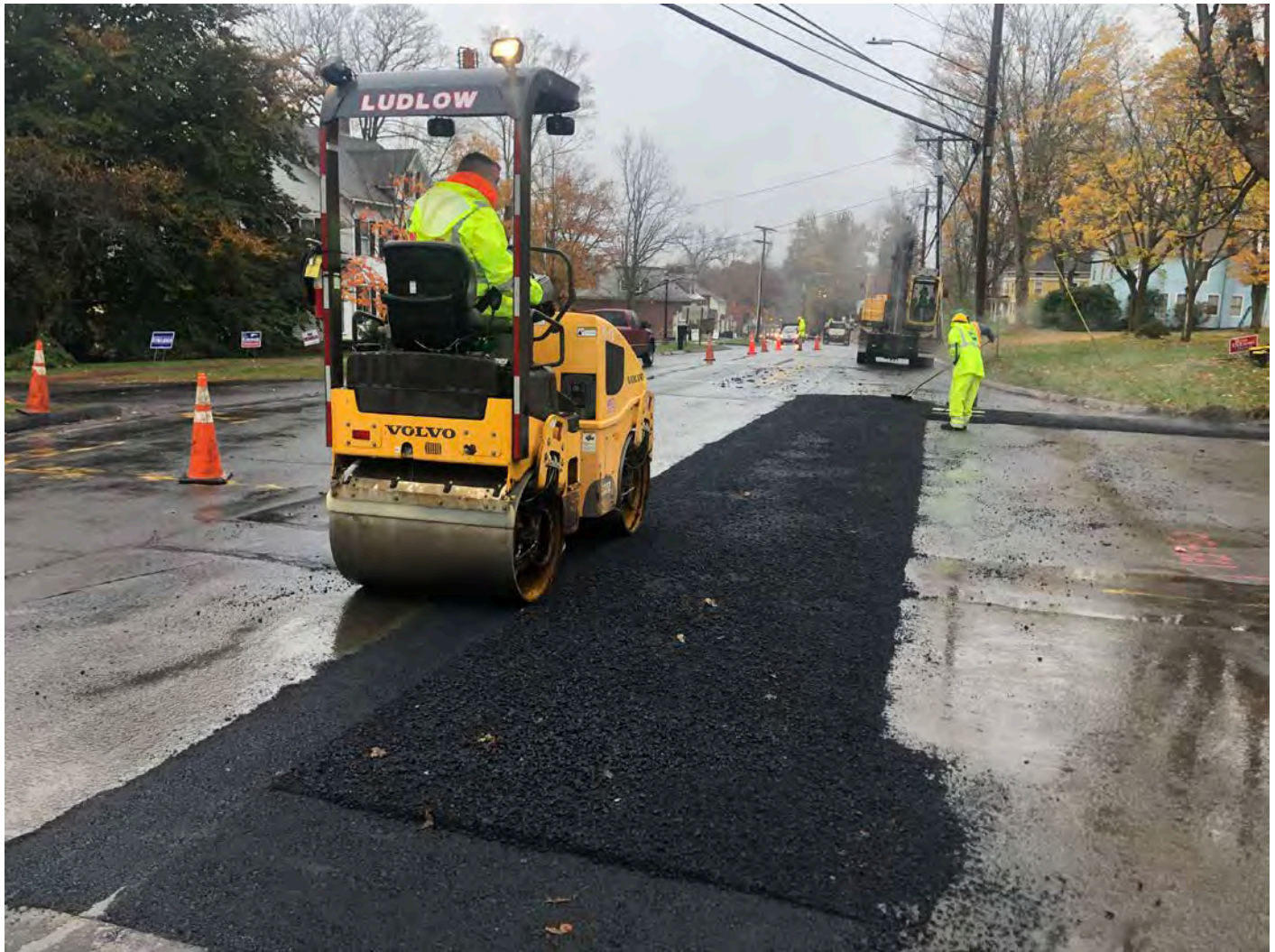
Picture 5: Ludlow compacting the third of three 3" lifts of asphalt between Stations 195+30 to 195+85 as part of permanent paving activities on the southbound lane of Main Street, Durham. View to the south.
