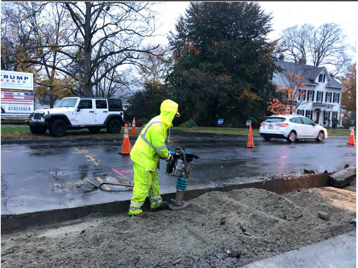
Picture 3: Ludlow compacting 1.5" processed gravel between Stations 195+30 to 195+85 as part of permanent paving activities on the southbound lane of Main Street, Durham. View to the southeast.
