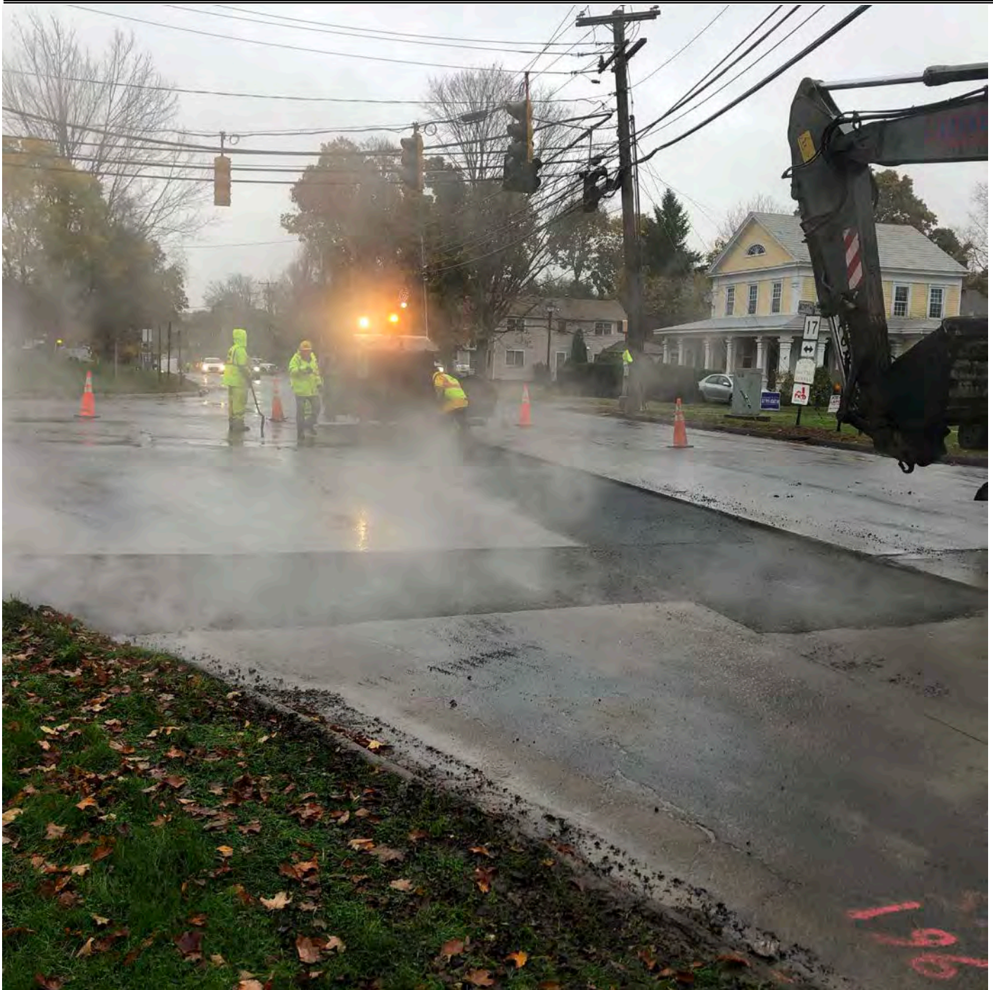
Picture 4: Ludlow placing asphalt on trench overcut between Stations 195+30 to 195+85 on the southbound lane of Main Street, Durham, as part of permanent paving activities. View to the north.
