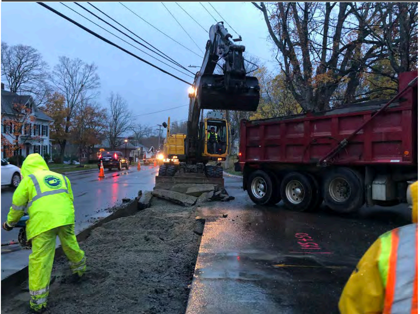
Picture 2: Ludlow stripping pavement away from trench overcuts between Stations 195+30 to 195+85 on the southbound lane of Main Street, Durham, as part of permanent paving activities. View to the south.
