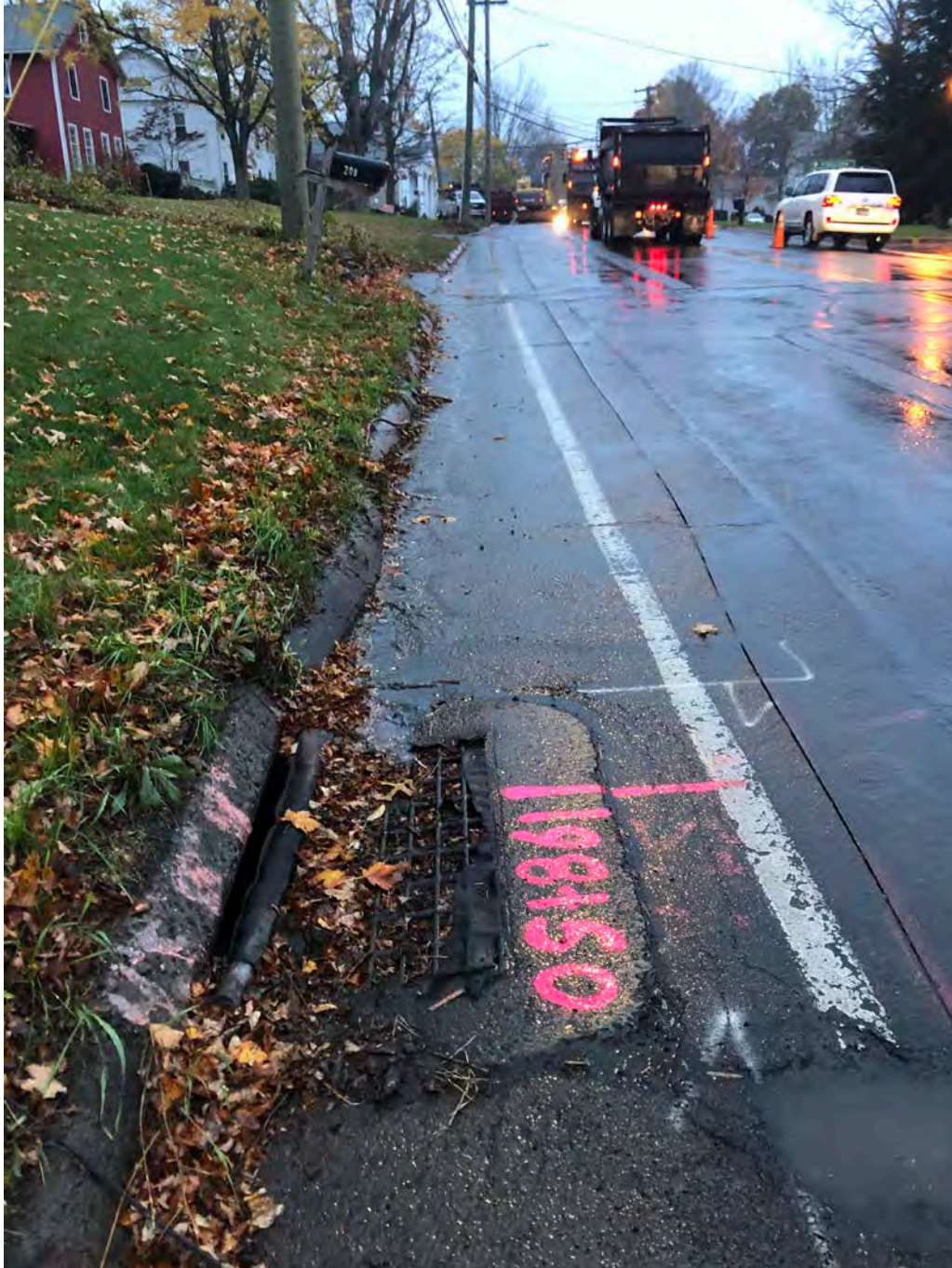
Picture 1: Catch basin with installed silt sock located at Station 198+50 located downstream and south of where Ludlow is placing permanent paving between Stations 195+30 to 195+85 on the southbound lane of Main Street, Durham. View to the north.
