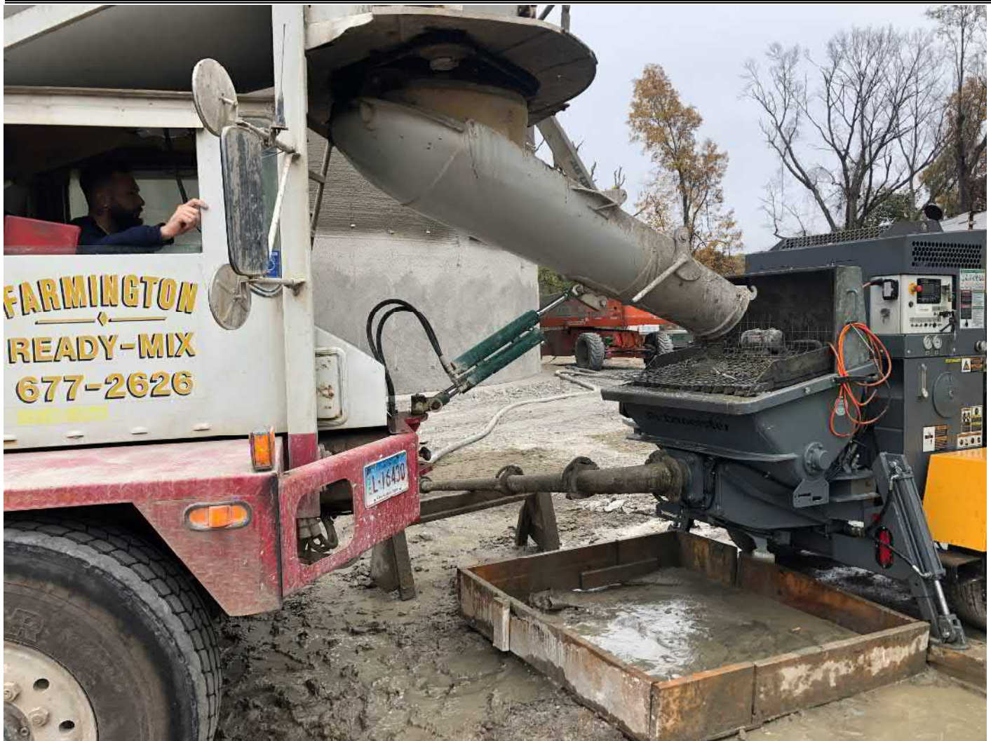
Picture 2: Farmington Ready Mix feeding shotcrete into pumper/mixer as DN Tanks applies the shotcrete to the exterior of the water tank. Water tank work zone located east of the Shared Access Driveway, Middletown.
