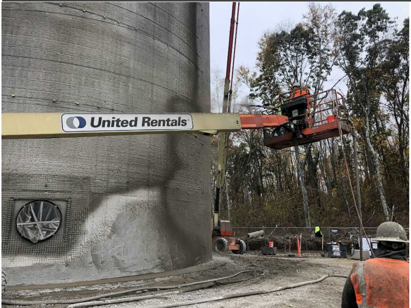
Picture 1: DN Tanks applying shotcrete to the northeast side of the water tank. Water tank work zone located east of the Shared Access Driveway, Middletown. View to the north.
