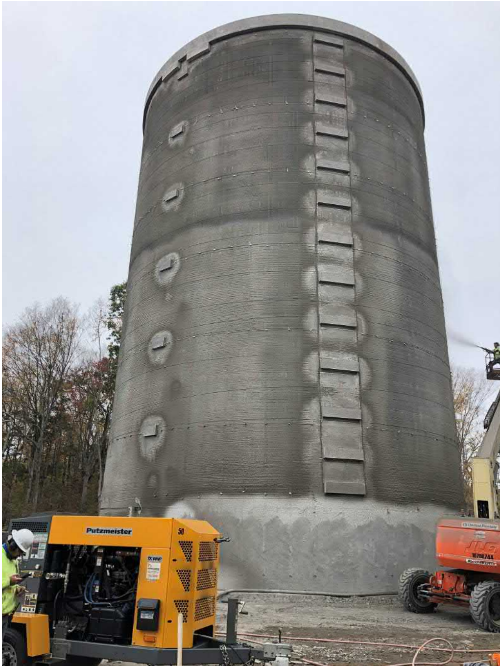
Picture 4: View of radio antennae supports (left) and ladder supports (right) after application of shotcrete last week. Water tank work zone located east of the Shared Access Road, Middletown.
