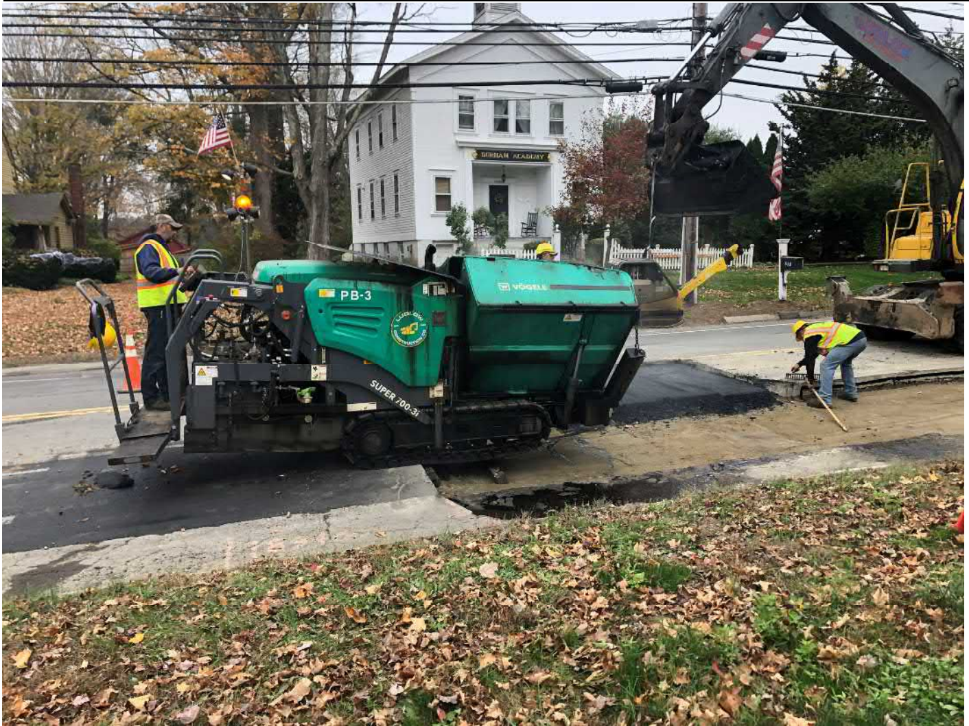
Picture 3: Ludlow preparing to place first of three 3" lifts of asphalt between Stations 189+00 and 192+70 on the southbound lane of Main Street, Durham. View to the east.
