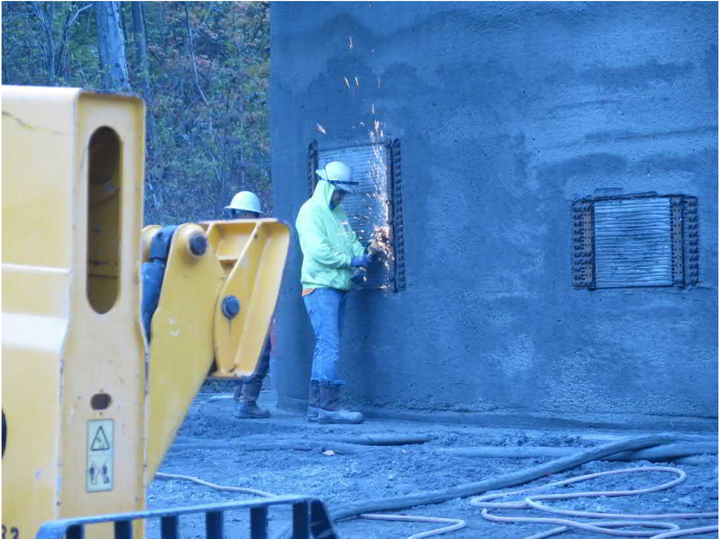
Picture 2: DN Tanks cutting pre-stress wires between clamps on the northwest manway. Water tank work zone located to the east of the Shared Access Driveway, Middletown. View to the northeast.
