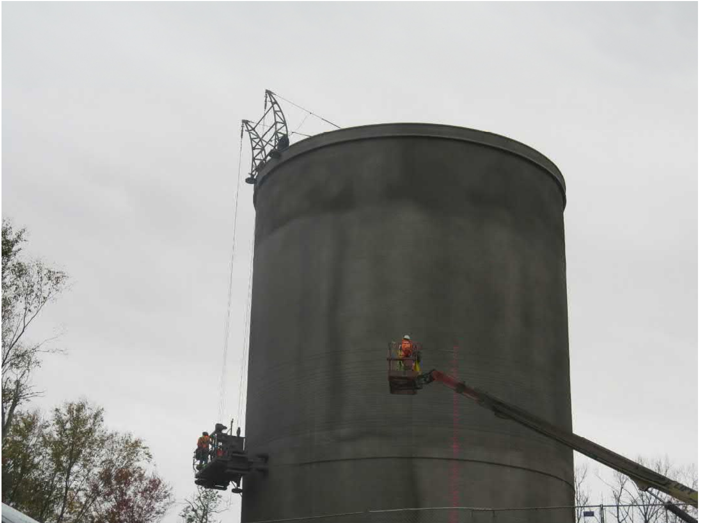
Picture 3: DN Tanks applying pre-stress wire to middle portion of tank wall. Water tank work zone located to the east of the Shared Access Driveway, Middletown. View to the east.
