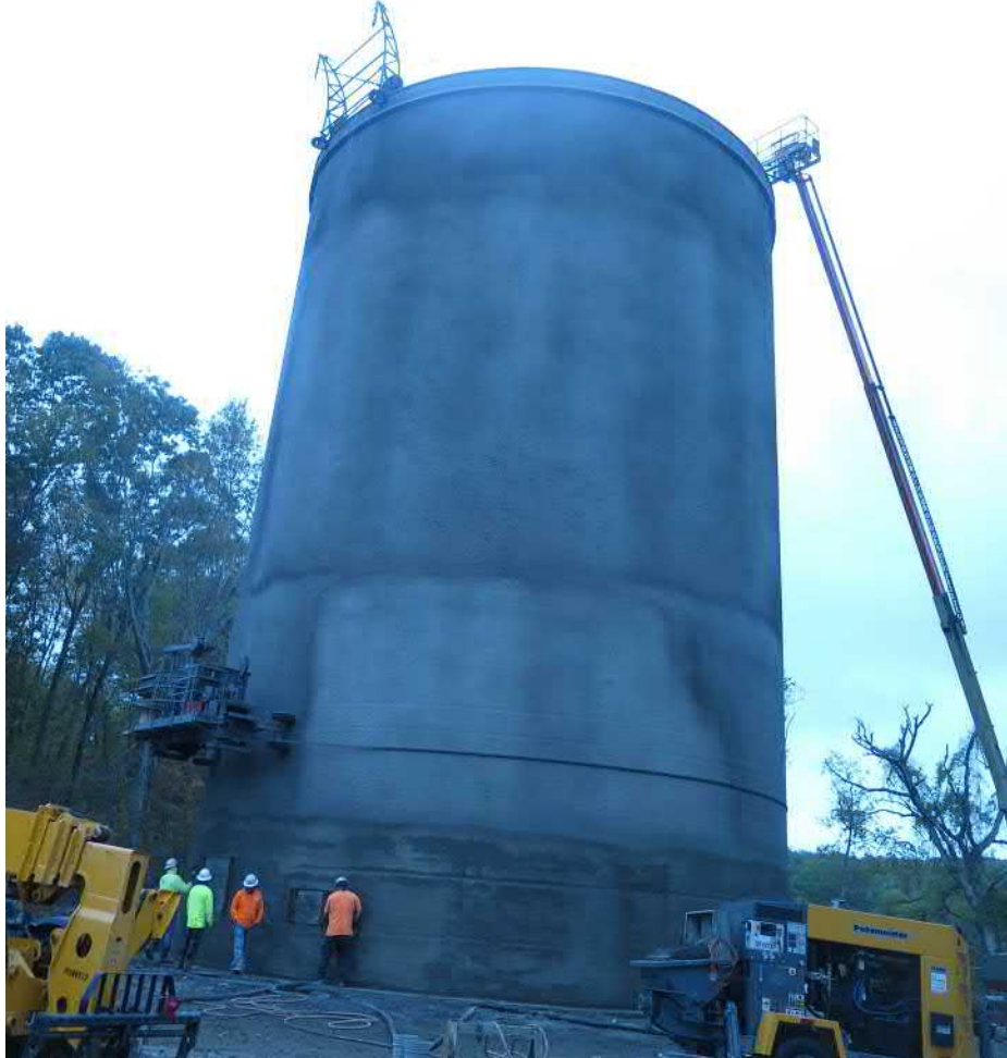
Picture 1: DN Tanks performing final tightening of wire clamps on overflow penetration. Water tank work zone located to the east of the Shared Access Driveway, Middletown. View to the east.
