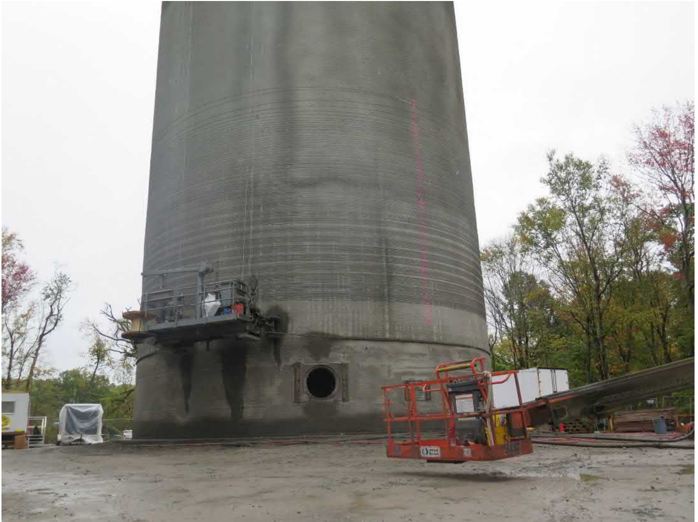
Picture 5: Extent of wire wrap completed today; within approximately 6 feet of top of manway. Water tank work zone located to the east of the Shared Access Driveway, Middletown. View to the east.
