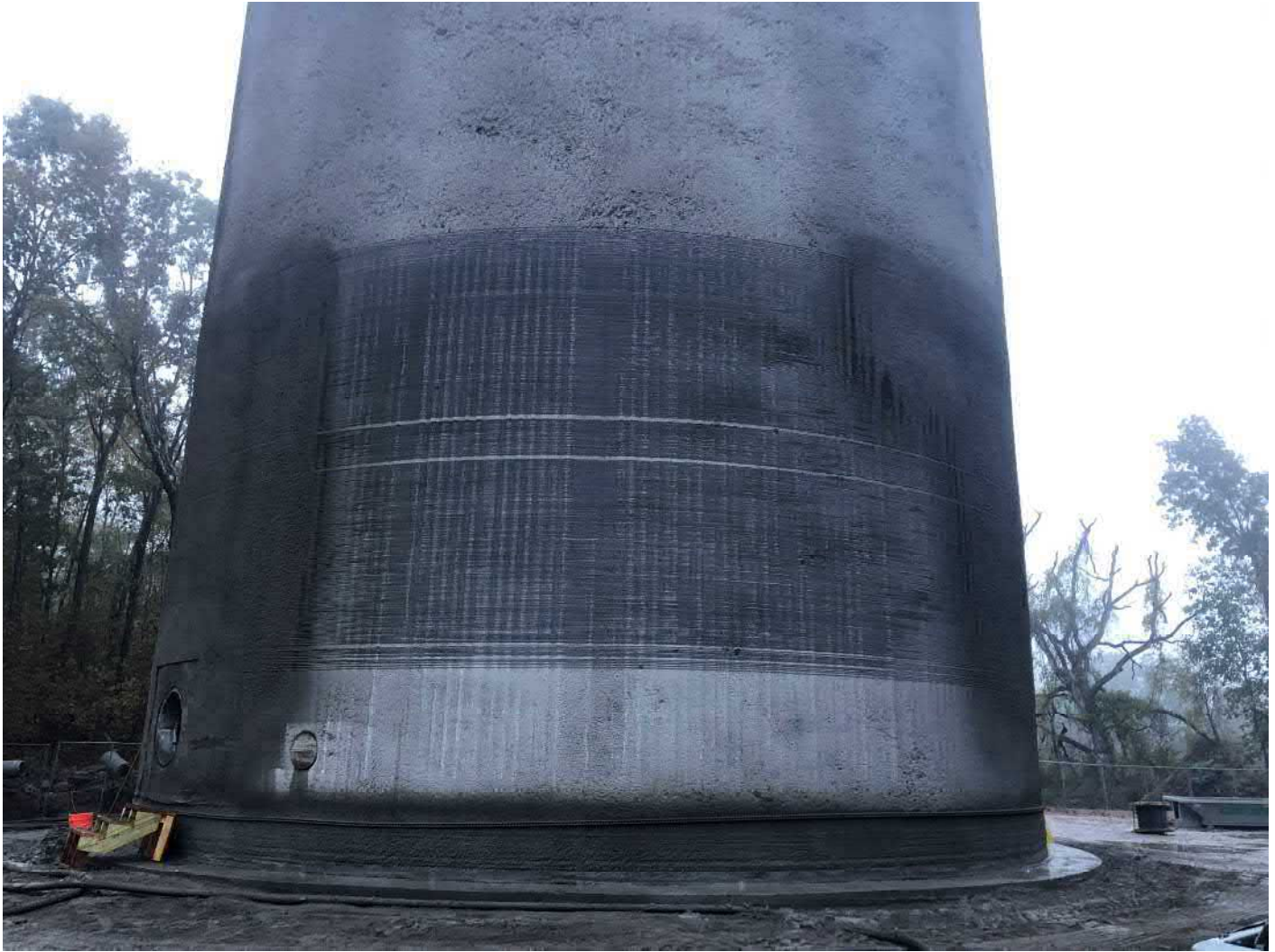
Picture 1: Prestressed wire on the southwest side of the tank was left exposed because DN Tanks ran out of shotcrete yesterday while it was being applied. Water tank work zone located to the east of the Shared Access Driveway, Middletown. View to the east.
