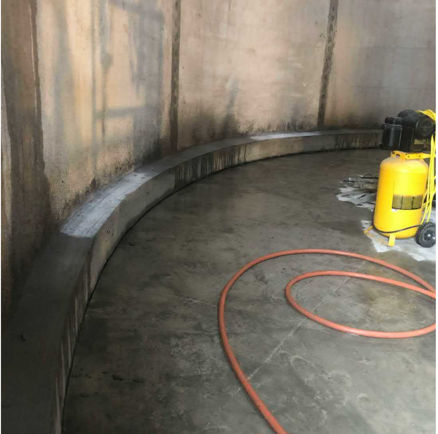
Picture 2: C.I.P cove with the concrete forms removed on the interior of the water tank. Water tank work zone located to the east of the Shared Access Driveway, Middletown.
