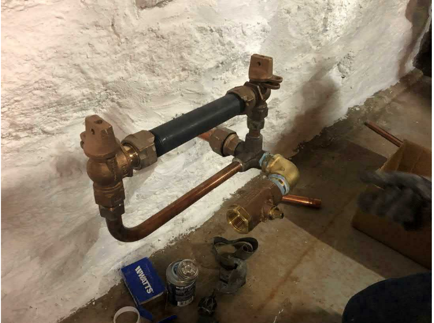
Picture 8: Plumbing associated with the connection of 13 Maple Avenue, Durham, to the public water supply. View to the southwest.
