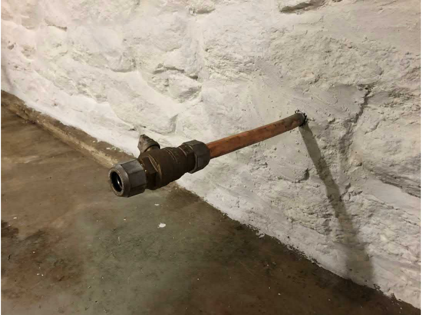
Picture 4: Water service line previously brought into the basement of the residence located at 13 Maple Avenue, Durham. View to the southeast.
