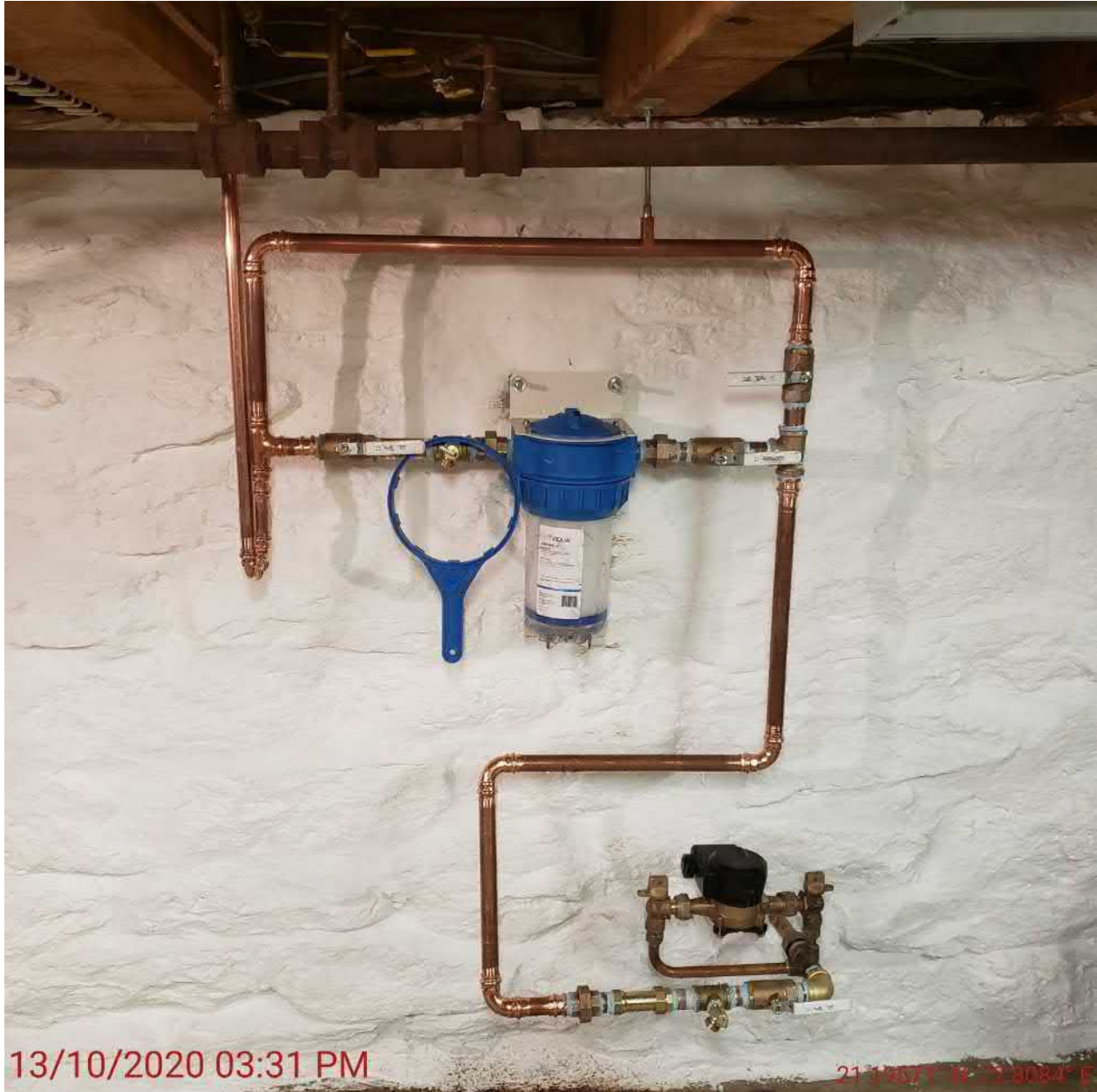
Picture 9: Water meter, backflow preventer and filter installed at 13 Maple Avenue, Durham.
