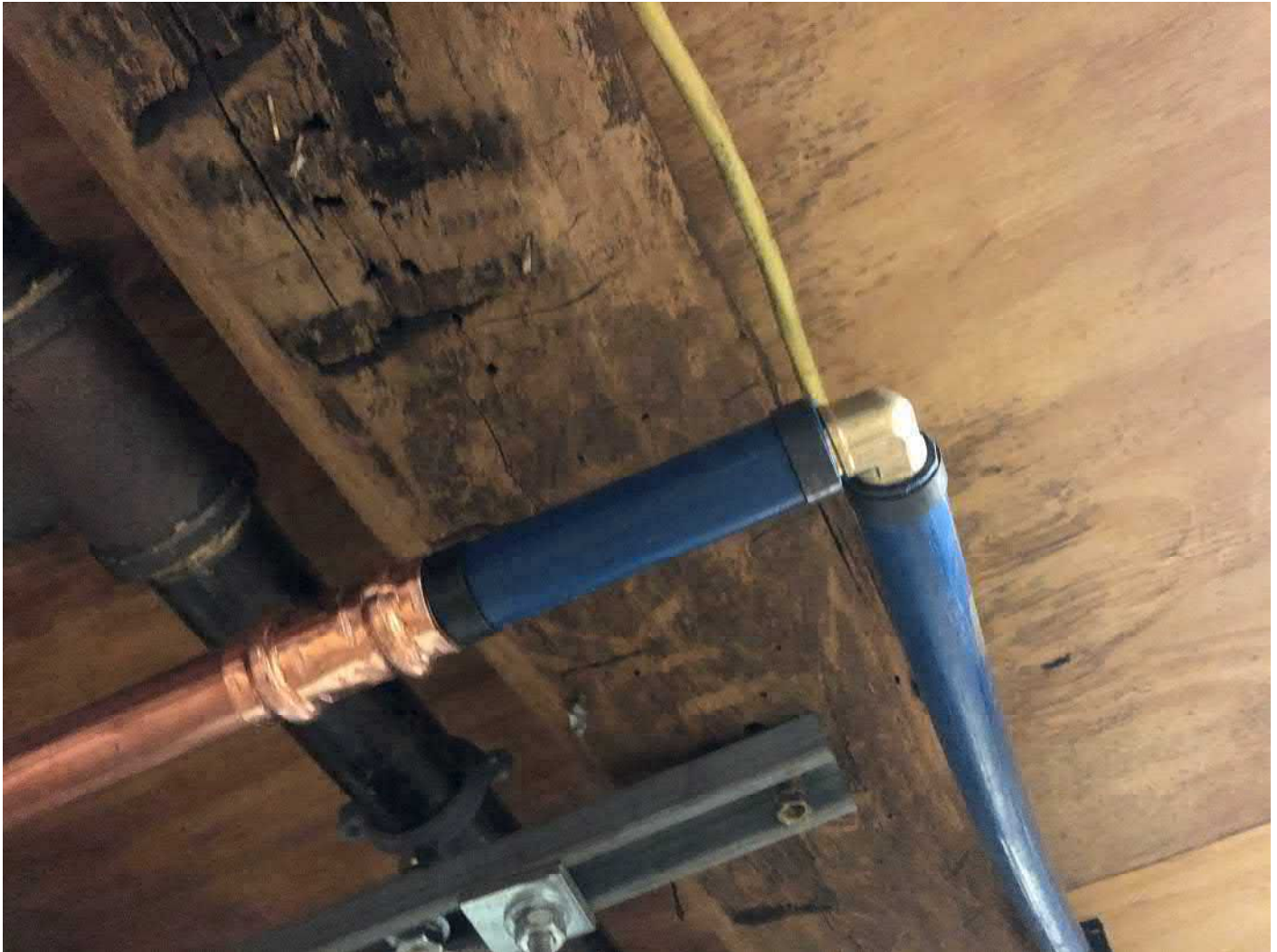
Picture 6: Copper pipe and PEX tubing used in connecting the residence at 13 Maple Avenue, Durham to the public water supply.
