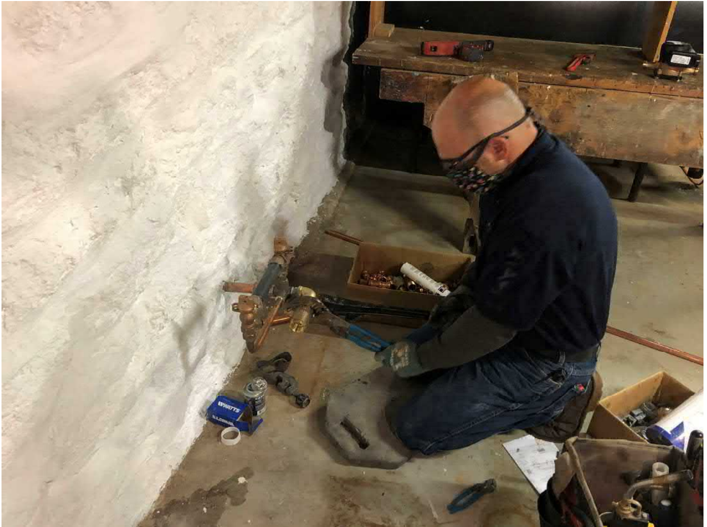
Picture 5: Fazzino working on connecting the residence at 13 Maple Avenue to the public water supply. View to the southwest.
