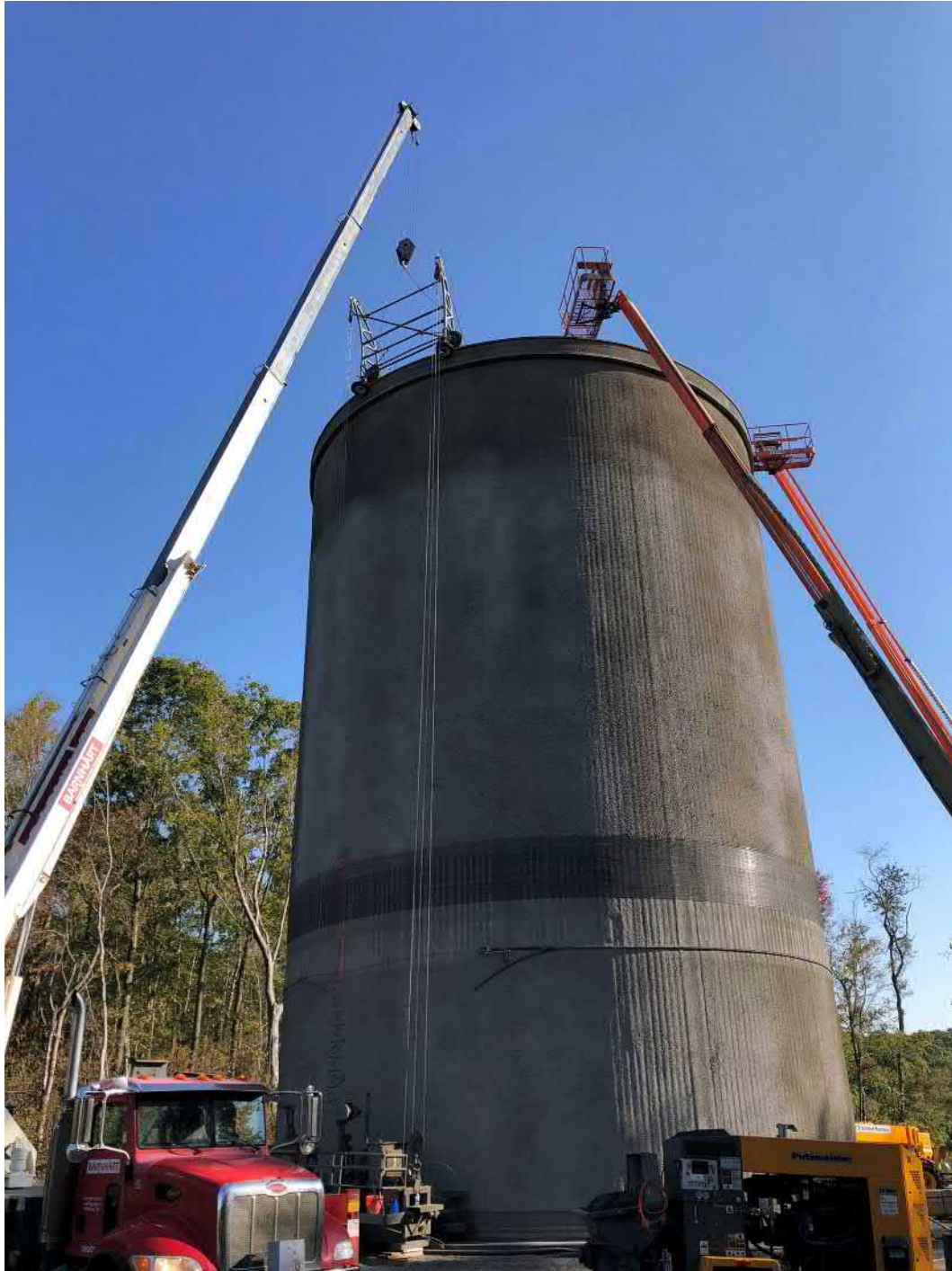
Picture 4: Barnhart operating crane to assist in DN Tanks in adjusting the anchor point for the wire wrapping cart on the top of the water tank. Water tank work zone located to the east of the Shared Access Driveway, Middletown. View to the northeast.
