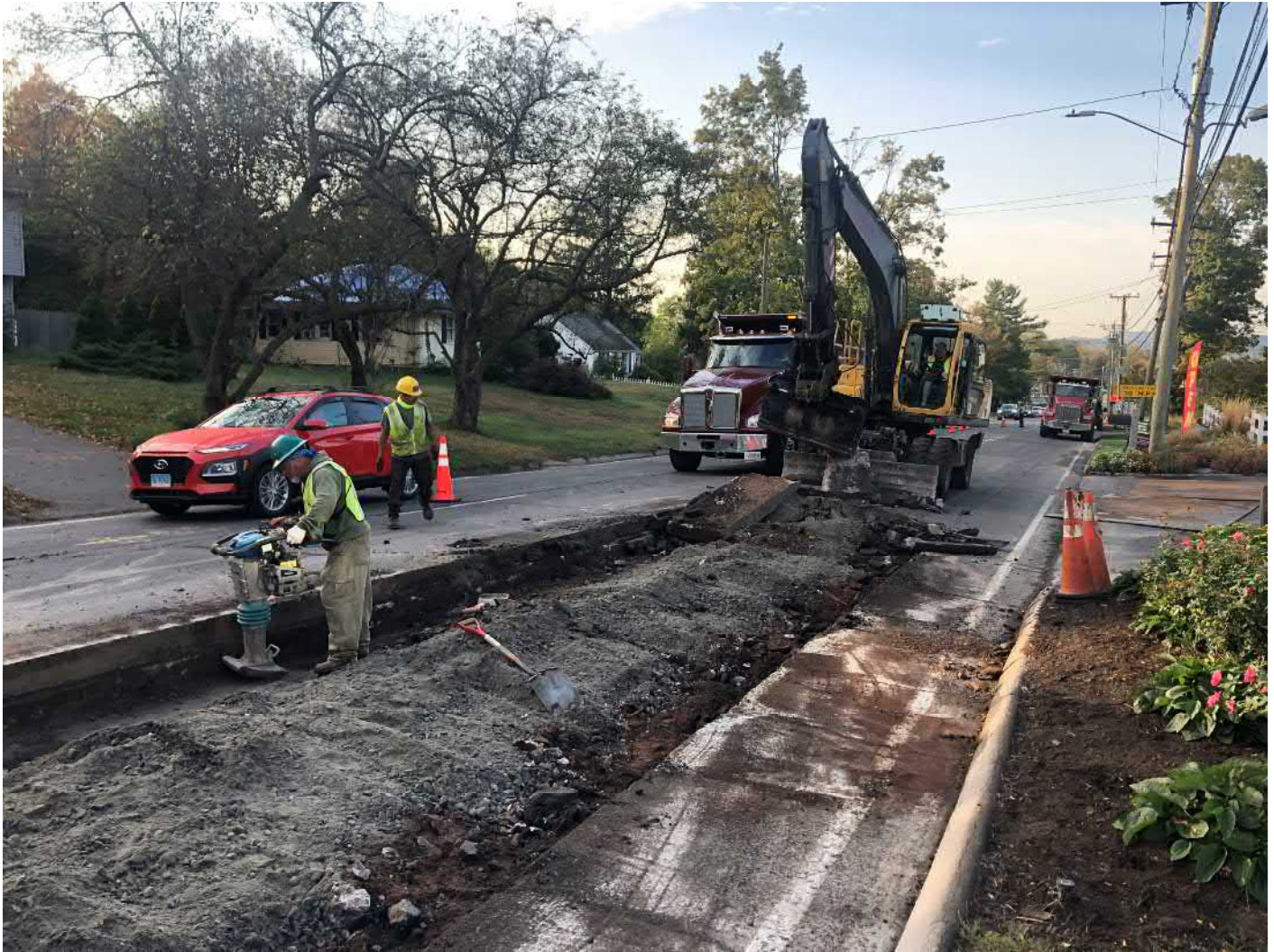
Picture 3: Ludlow using a Jumping Jack to compact 1.5” processed gravel as they also remove asphalt in preparation for the placement of permanent paving on the southbound lane of Main Street, Durham. View to the southeast.
