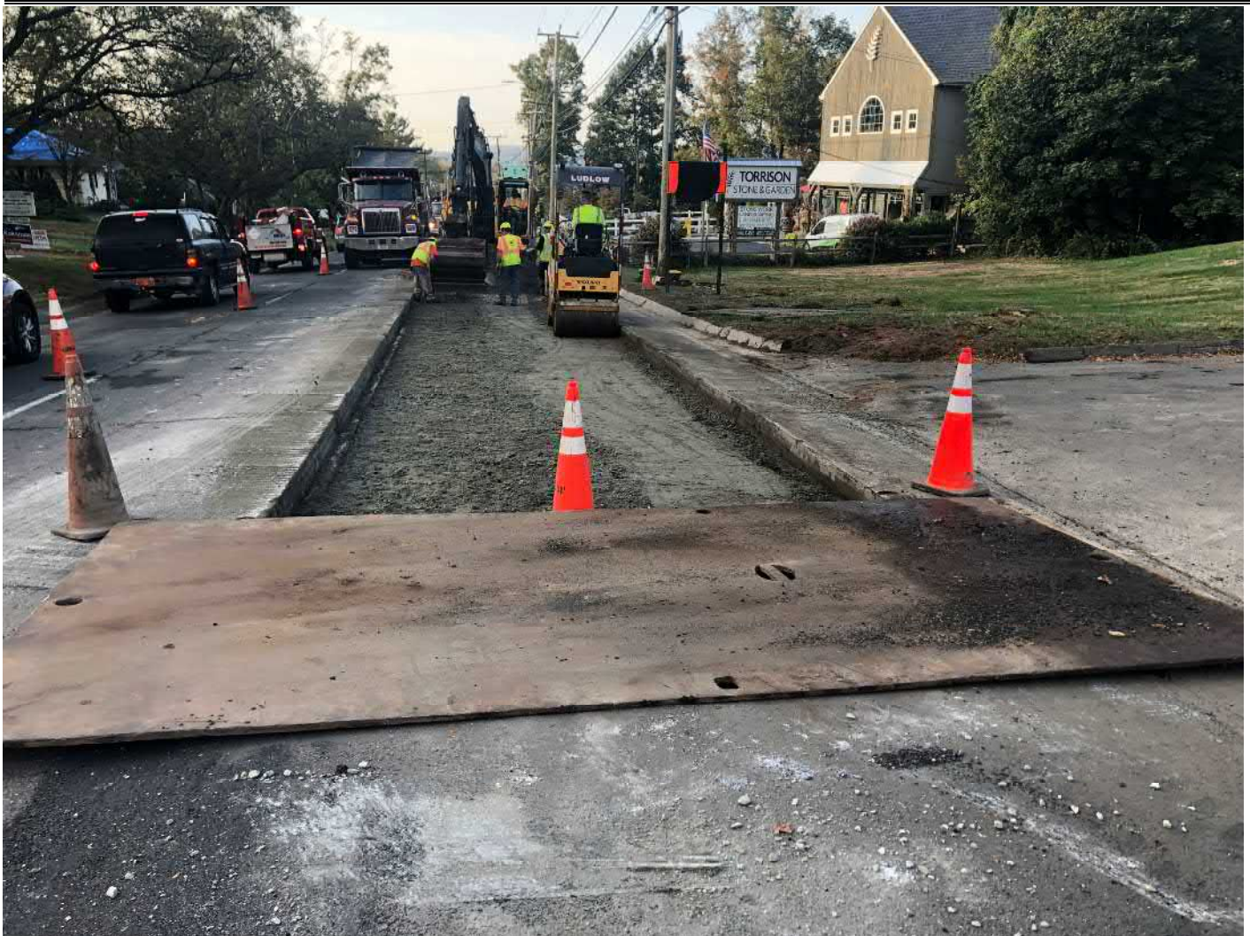
Picture 2: Ludlow stripping back asphalt and compacting 1.5” processed gravel as they prepare to place permanent paving on the southbound lane of Main Street, Durham. View to the south.
