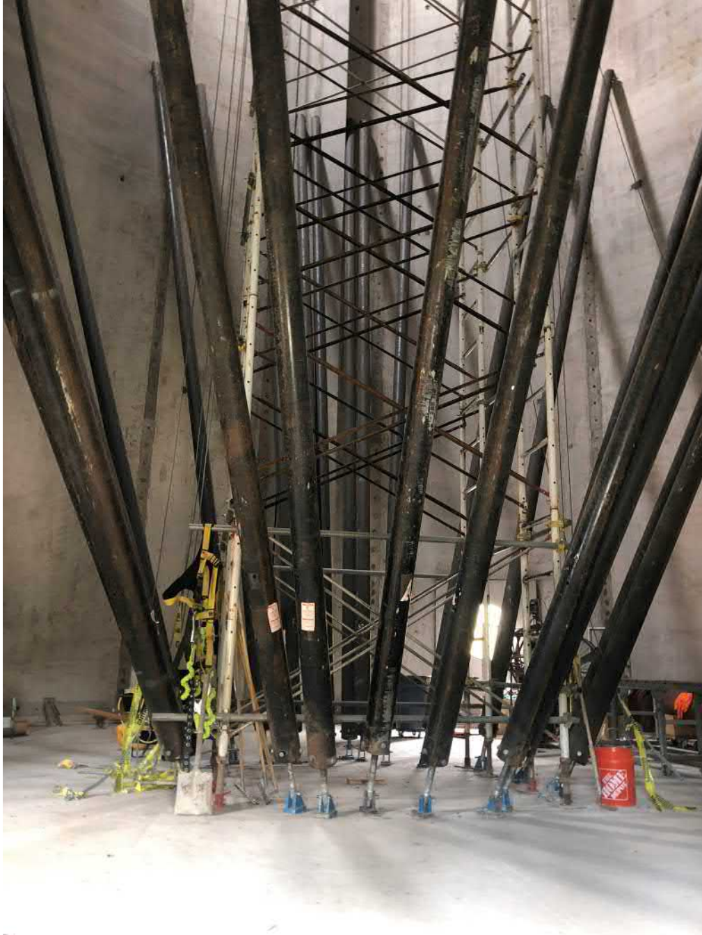
Picture 6: Knee braces in place inside of the water tank. Water tank work zone located to the east of the Shared Access Driveway, Middletown. View to the northeast.
