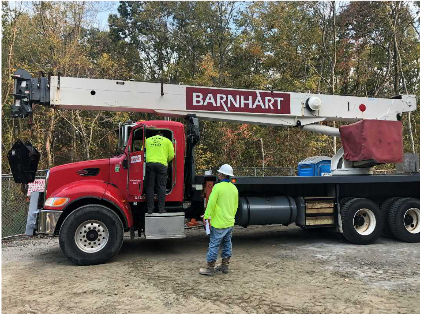
Picture 1: Small crane from Barnhart that DN Tanks had mobilized to the water tank work zone east of the Shared Access Road to assist with wire wrapping activities. View to the north.
