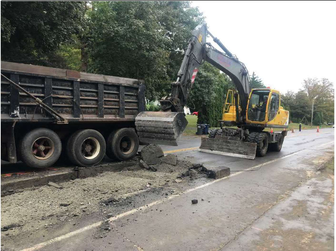
Picture 2: Ludlow stripping back asphalt as they prepare to place permanent paving on the southbound lane of Main Street, Durham from Stations 146+30 to 148+65. View to the southeast.
