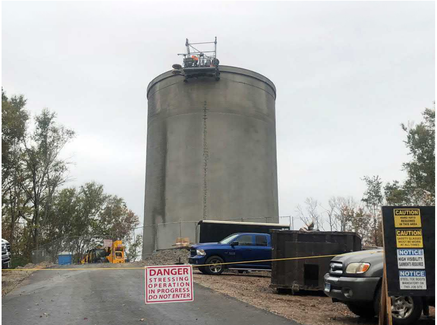
Picture 1: DN Tanks placing a second layer of prestressed wire around the dome rim of the water tank. Water tank work zone, east of the Shared Access Driveway, Middletown. View to the northeast.
