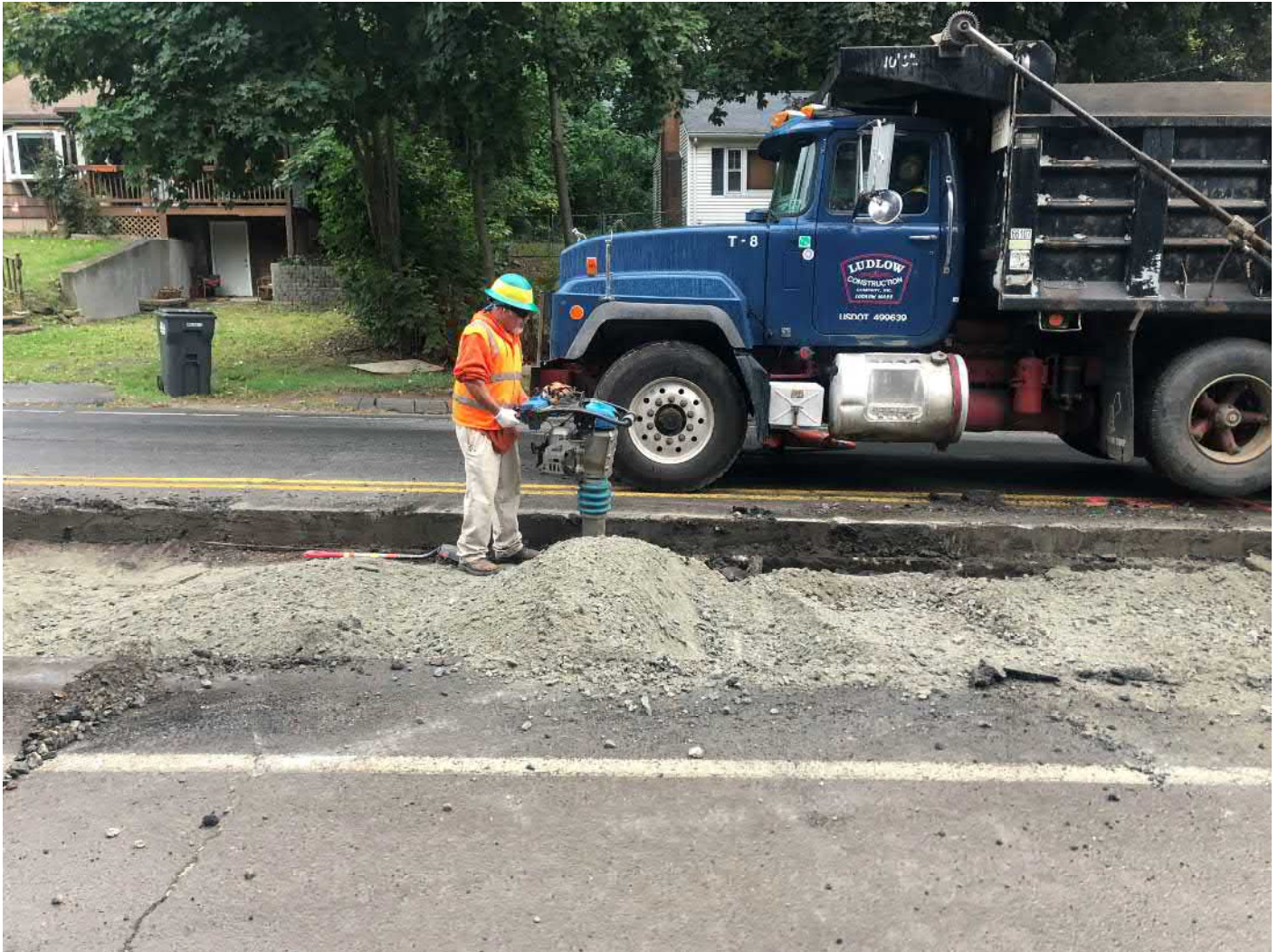
Picture 3: Ludlow compacting 1.5" processed gravel as part of permanent paving on the trench cutbacks on the southbound lane of Main Street, Durham from Stations 146+30 to 148+65. View to the east.
