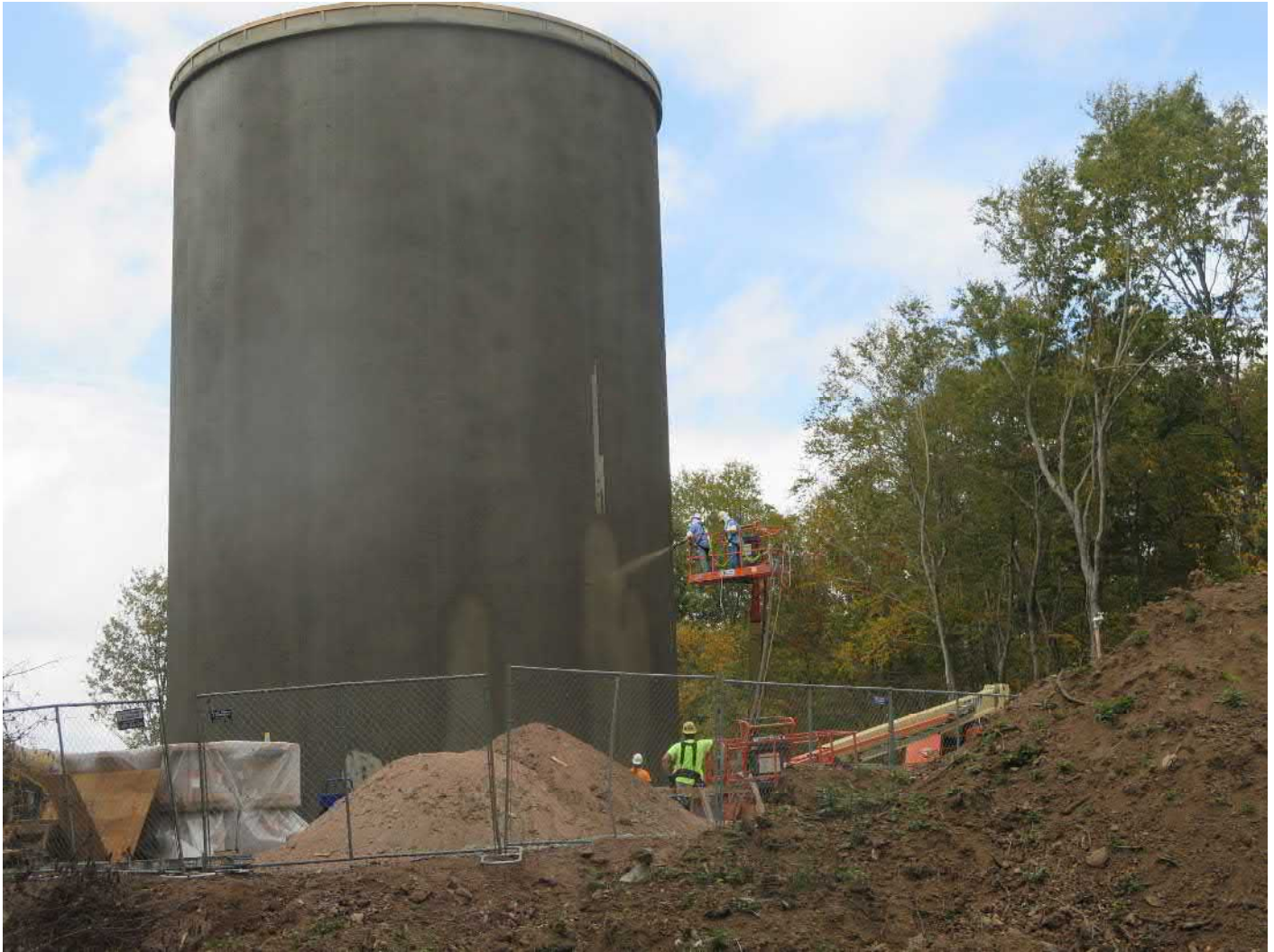
Picture 5: DN Tanks crew re-coating gap in concrete coat on northeast side of tank. Shared access driveway, Middletown; view to the northwest.
