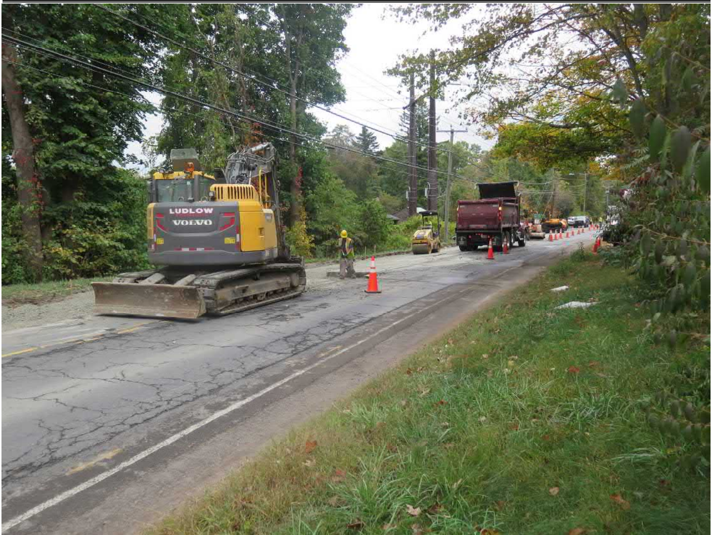
Picture 1: Grading and compacting cut-back trench on southbound lane of South Main Street, Middletown. View to the north.
