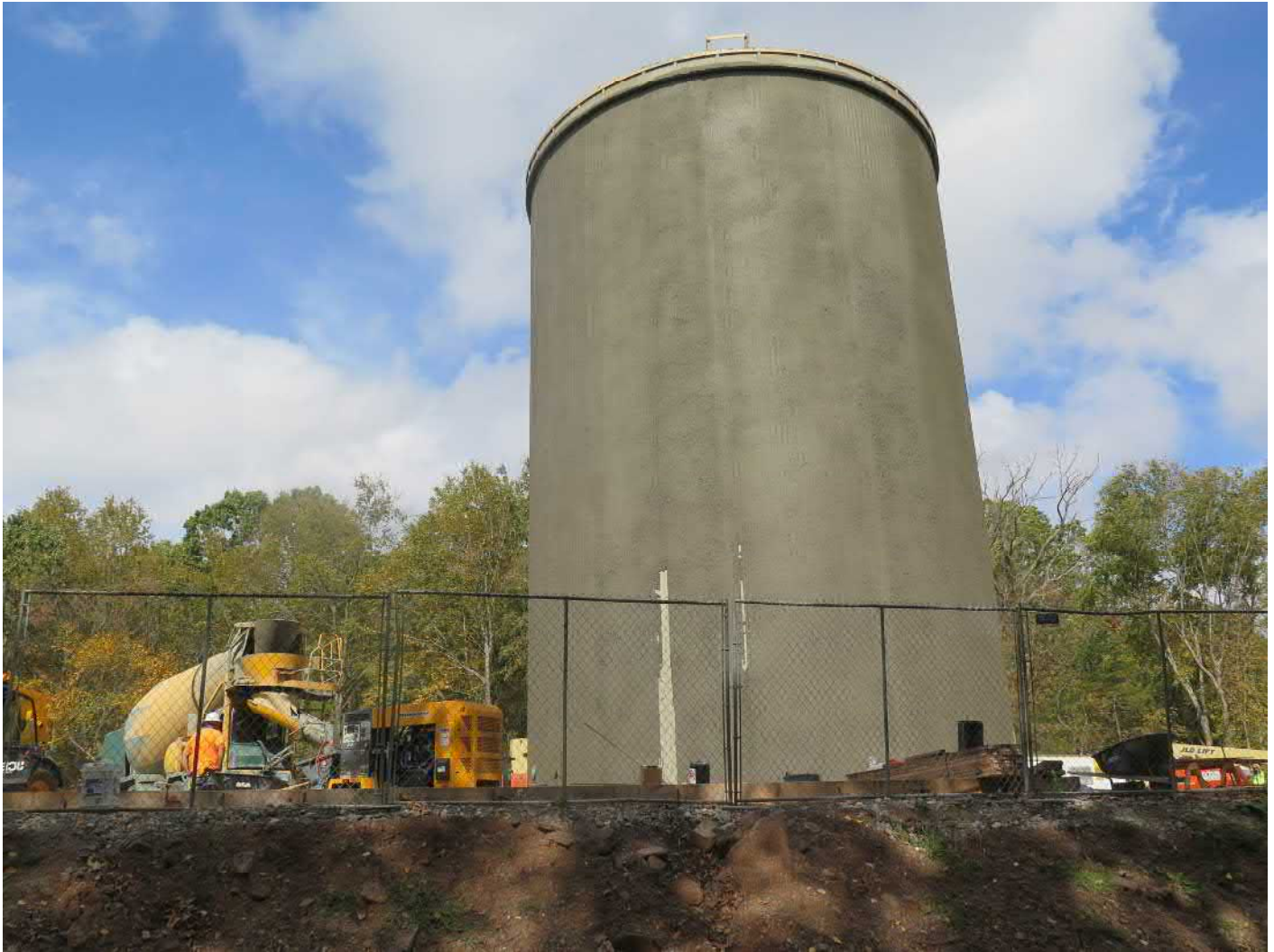
Picture 4: Completed coat of shotcrete on tank walls, showing a small gap in the coat. Shared access driveway, Middletown; view to the north.
