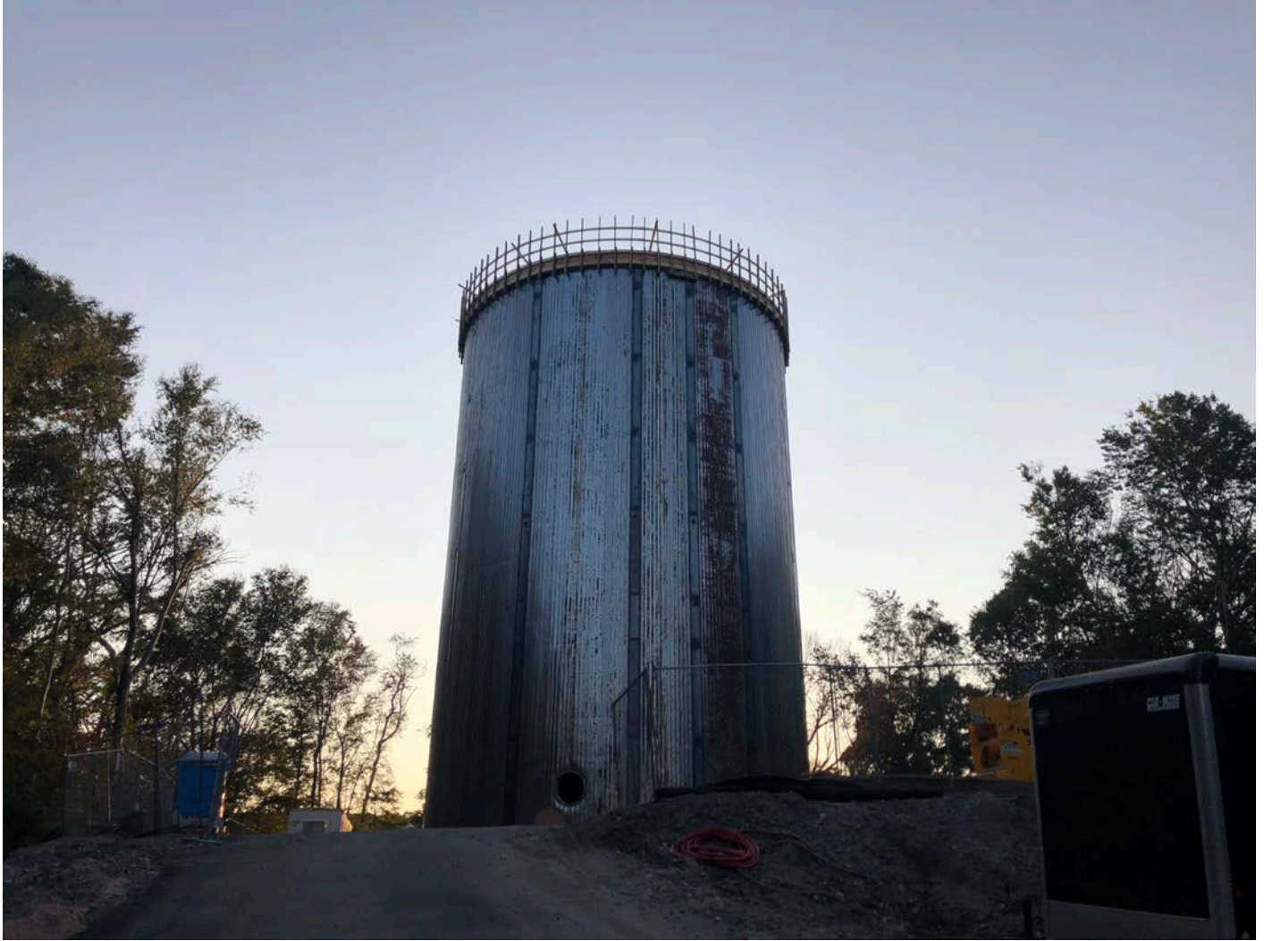
Picture 1: Guardrails and toe boards installed along the perimeter of the top of the water tank by DN Tanks. Water tank work zone, east of the Shared Access Driveway, Middletown. View to the east.
