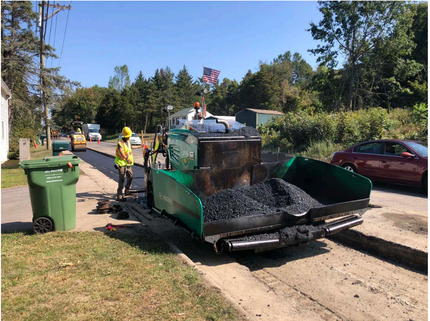
Picture 3: Ludlow placing the first of three 3” lifts of asphalt between Stations 122+75 and 126+00 as part of trench cutback paving activities on the southbound lane of S. Main Street, Middletown. View to the north.
