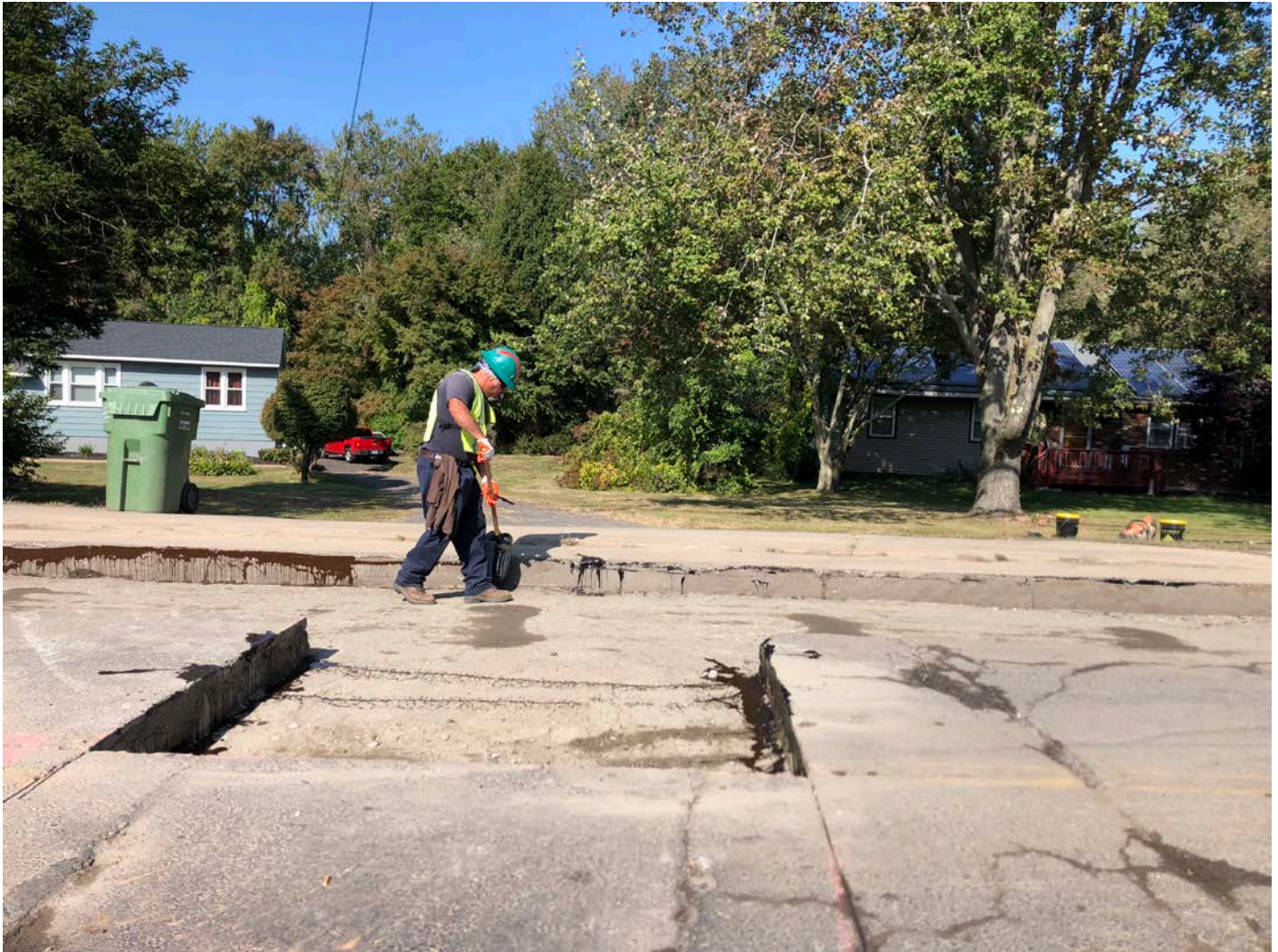
Picture 2: Ludlow applying tack coat to the cut edges of pavement as part of trench cutback paving activities on the southbound lane of S. Main Street, Middletown. View to the west.
