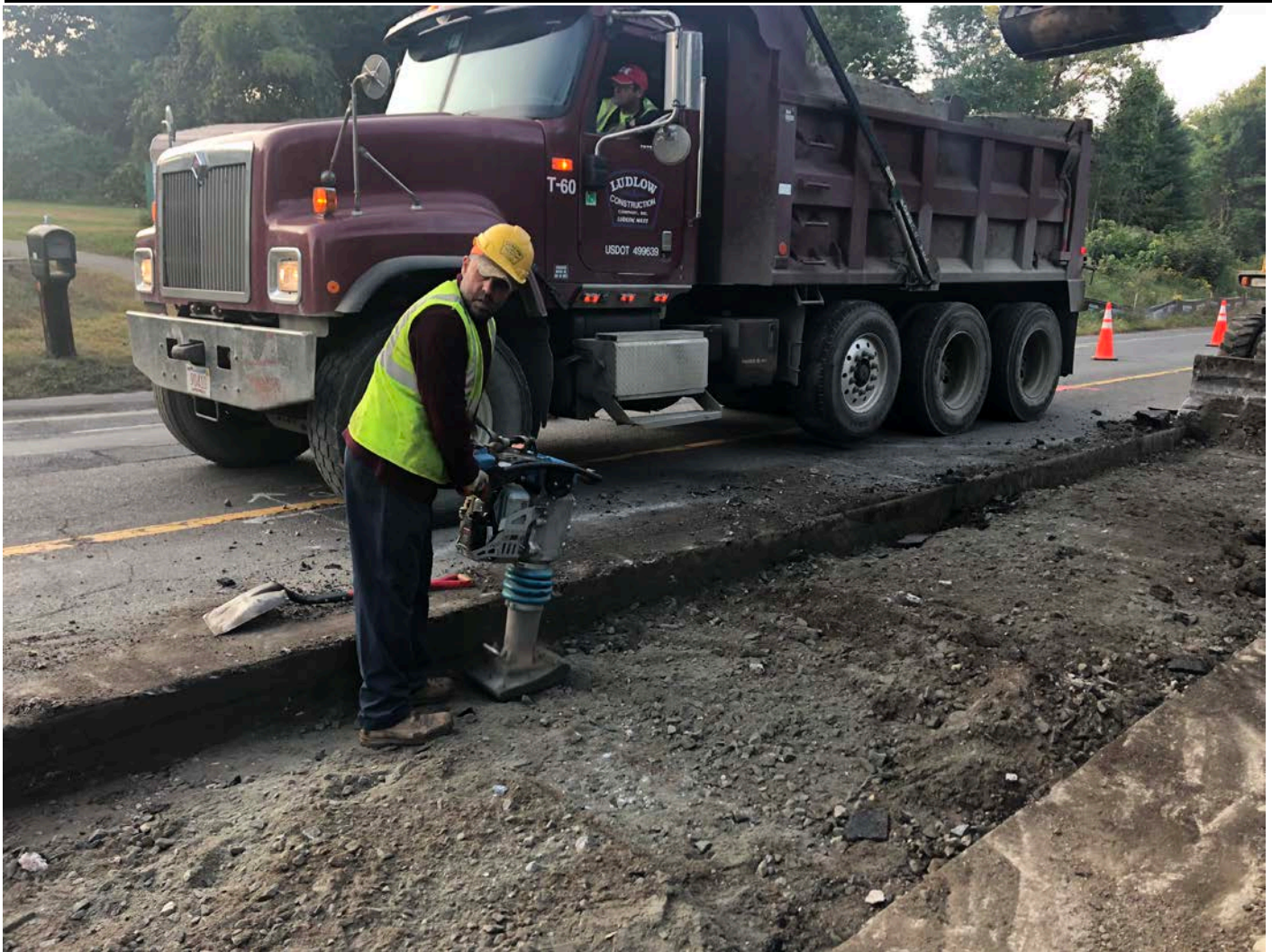
Picture 4: Ludlow using a jumping jack to compact 1.5” processed gravel along the edge of cut pavement as part of trench cutback paving activities on the southbound lane of S. Main Street, Middletown. View to the north.
