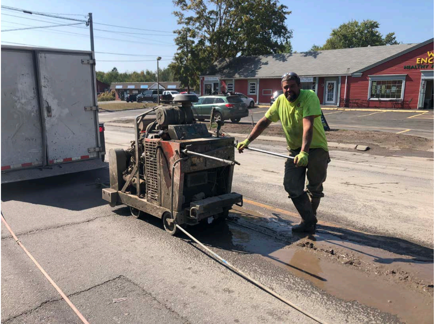
Picture 5: Veilleux saw cutting on the northbound lane of Main Street, Durham at Station 165+50. View to the southwest.
