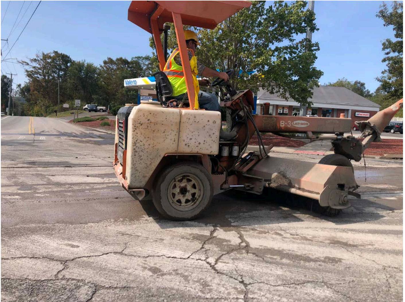
Picture 4: Ludlow cleaning up with the Broce Broom after saw cutting activities on Main Street, Durham. View to the west.
