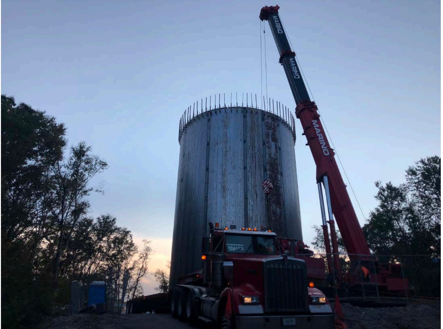
Picture 1: P-brackets installed along the perimeter of the top of the water tank as DN Tanks continues to construct guardrails. Water tank work zone, east of the Shared Access Driveway, Middletown. View to the east.
