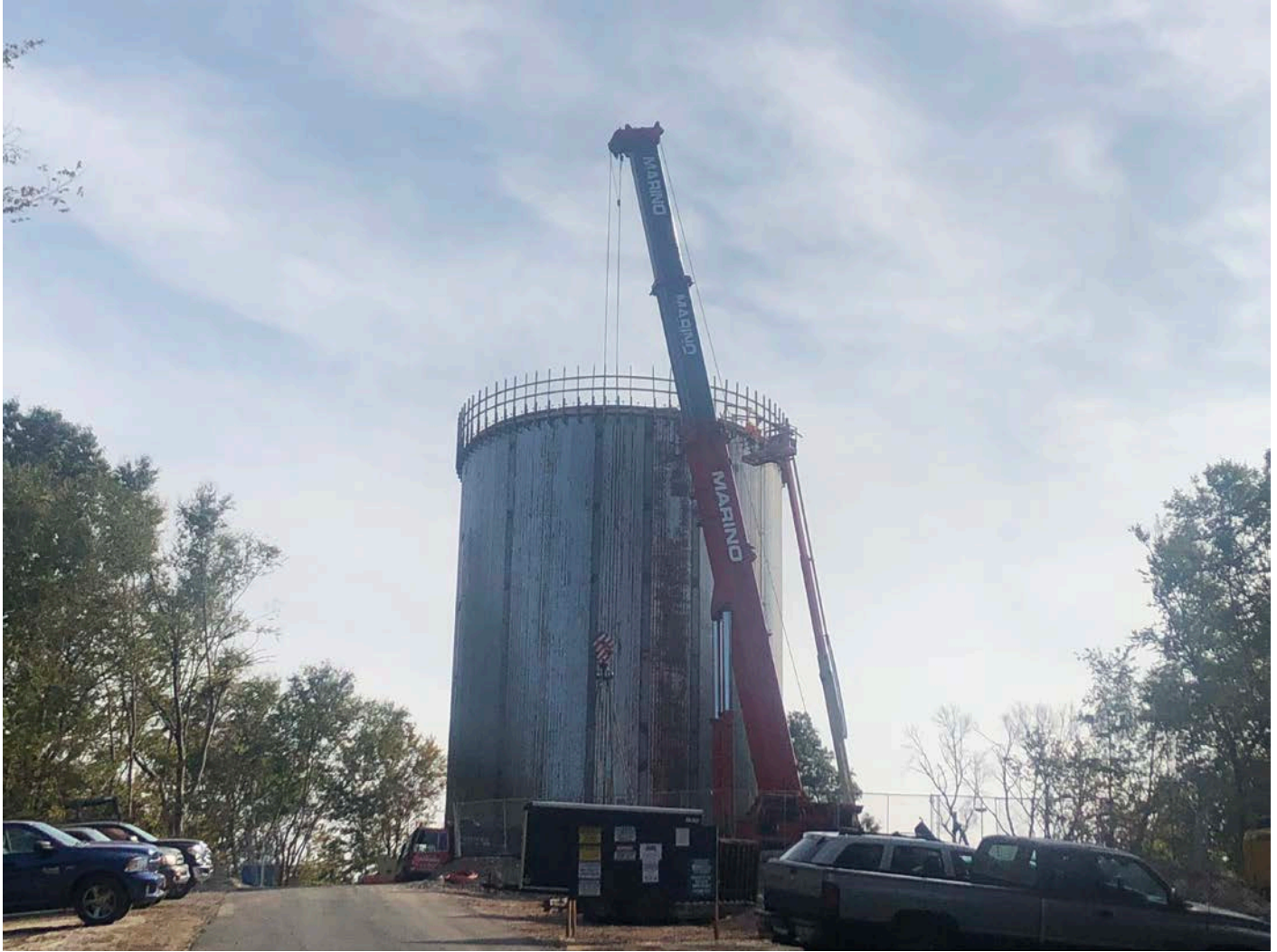
Picture 3: View of progress as DN Tanks continues to construct a guardrail along the perimeter of the top of the water tank. Water tank work zone, east of the Shared Access Driveway, Middletown. View to the east.
