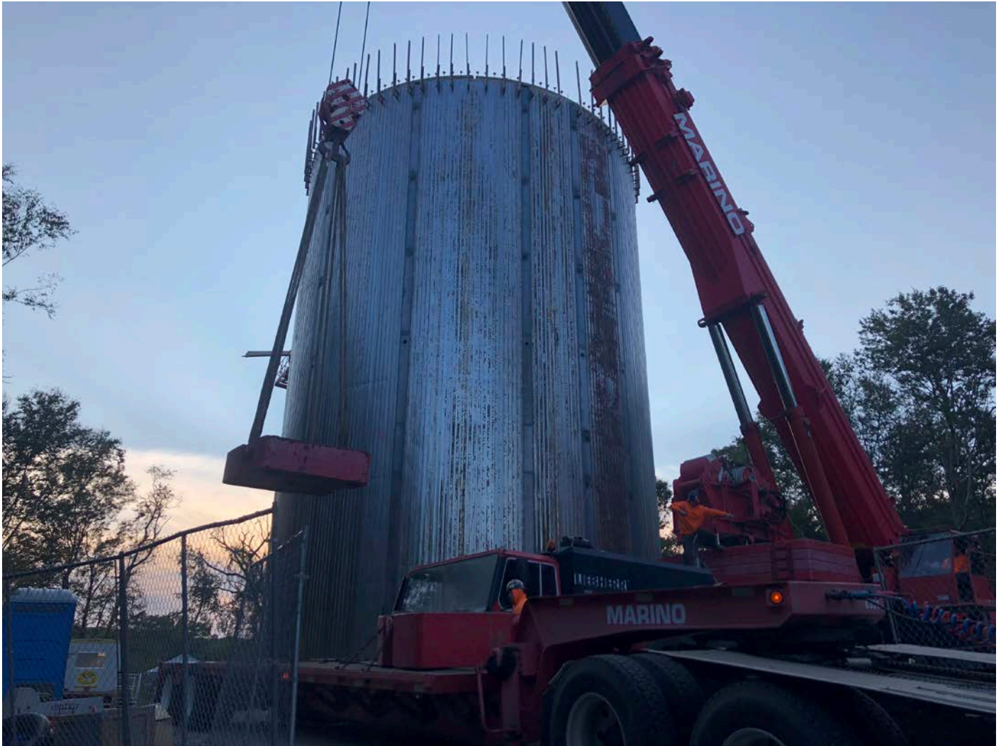
Picture 2: Marino placing one of the counterweights from the 400-ton crane onto the bed of a flatbed as they prepare to demobilize from the site today. Water tank work zone, east of the Shared Access Driveway, Middletown. View to the east.
